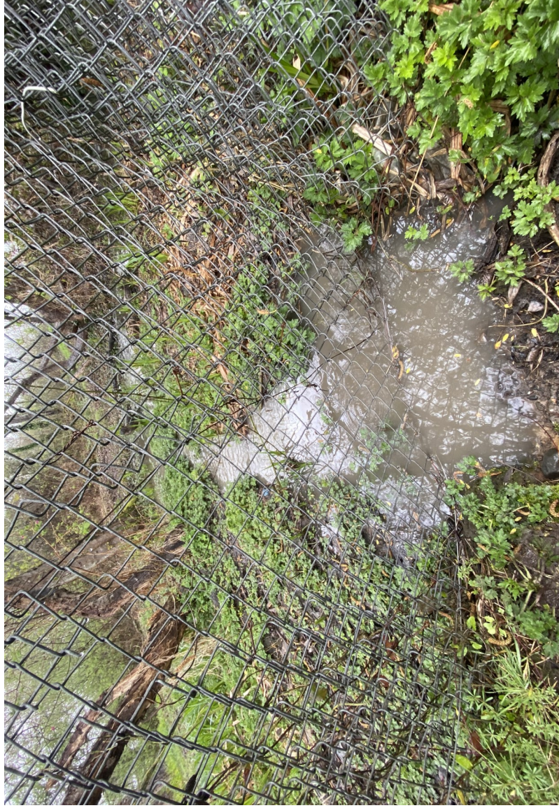
Northern discharge sampling location, D#2. Discharge received from subsurface corrugated pipe receiving runoff from concrete lined ditch and adjacent areas.
