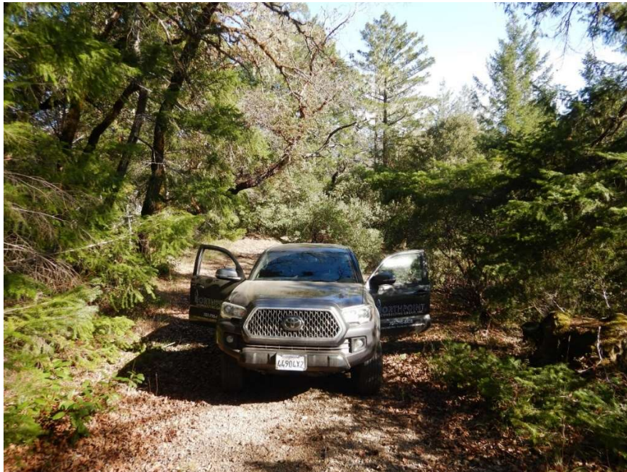
Figure 26: RP 25. Pinch Point. Vegetation growth in roadway. 13-ft wide. Vehicle traveling north-west. Photo taken facing south-east. (40.079638°, -123.766867°)
