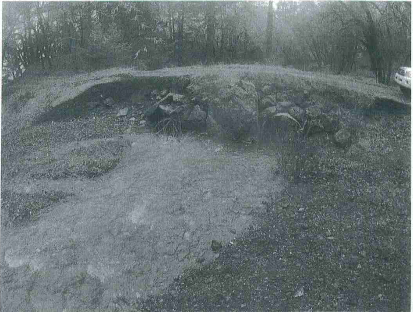
Site 50: Double barrel Class II watercourse crossing, consisting of a 48" metal culvert and a 48". See mitigation report for details.
