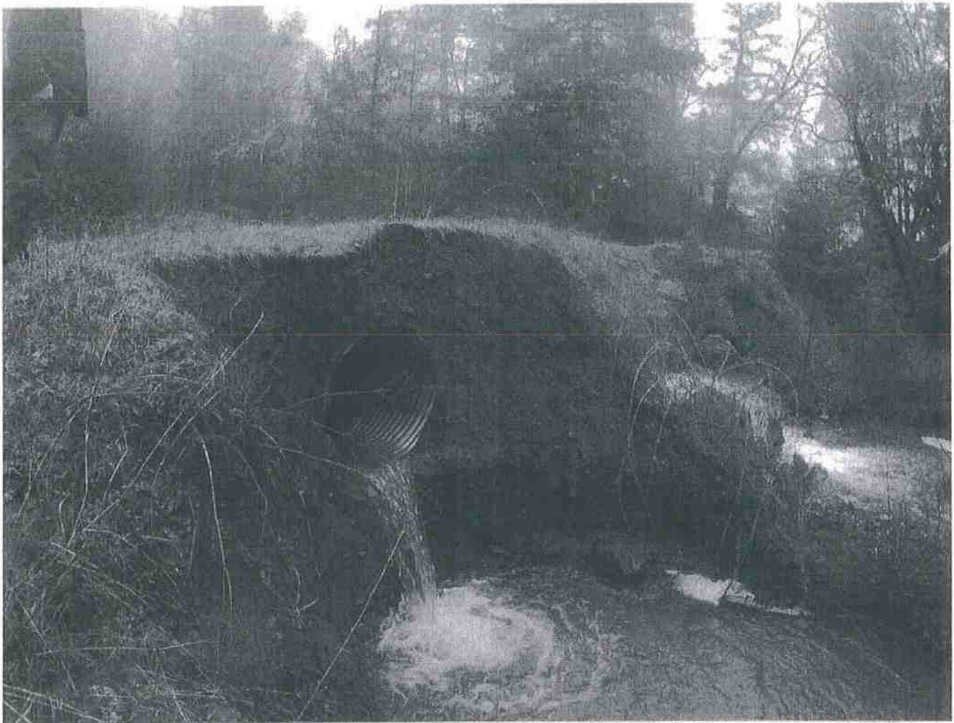
Site 50 – Alternate view, this watercourse crossing is not functioning adequately due to the culverts being inadequately sized and too short. Additionally, the inlet of the metal culvert is crushed and obstructed. See mitigation report for further details.
