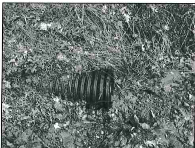
Photo #17 Cobb Rd Looking @ Exposed Culvert
