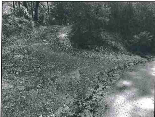
Photo #15 Cobb Rd & Private Driveway Looking SE @ Exposed Culvert
