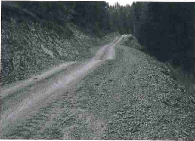
Figure 8. Rolling dips installed to drain an out-sloped road. Source: Bill Weaver, Pacific Watershed Associates.
