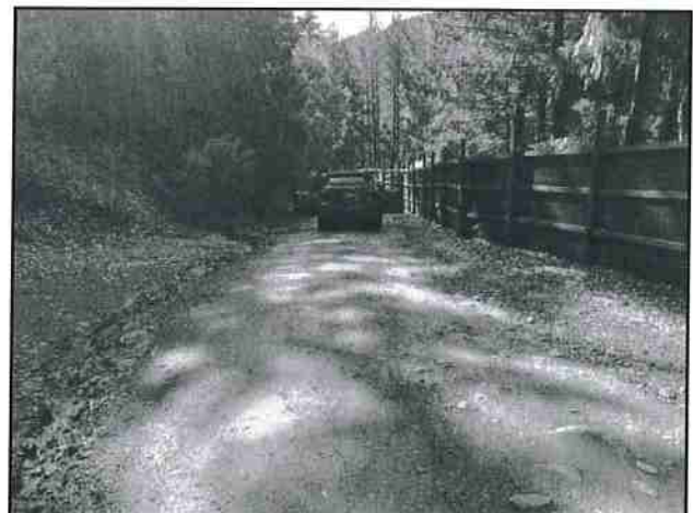
Photo #16 Cobb Rd & Private Driveway @ Pullout Looking South @ Exposed Culvert
