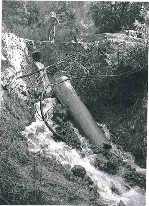
Figure 34. Outlet of a concrete culvert (30 inches in diameter) before the project. The culvert was placed too high in the fill, resulting in a 10-foot drop to the channel at the outlet. This caused erosion of the road fill and stream banks, eventually undermining the outer section of the culvert. Photo: Jared Gerstein.
