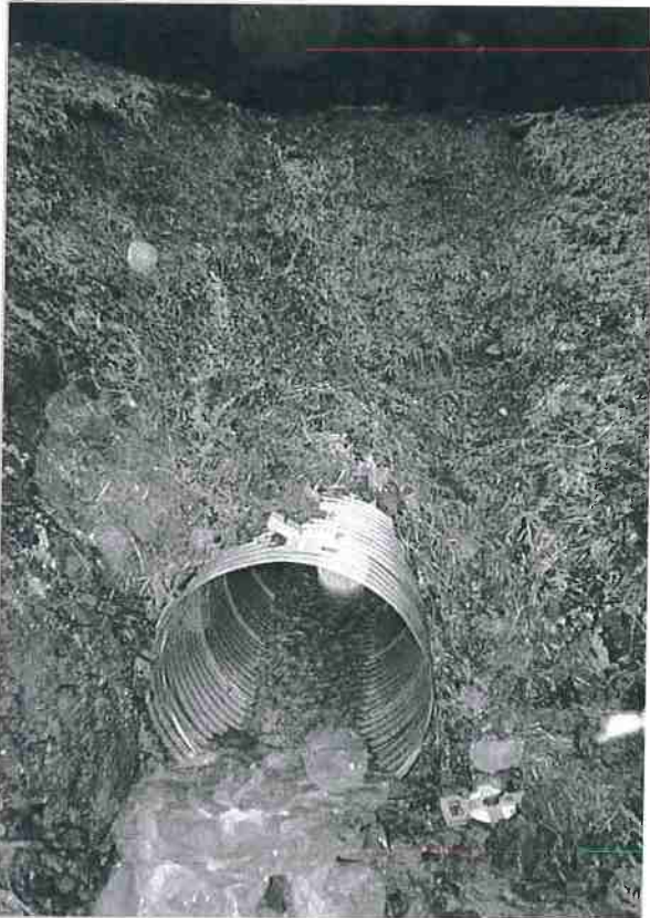
Figure 2. This cross drain delivers sediment from the roadside ditch under the road surface to a nearby stream. The road fill is also eroding. Photo: Jared Gerstein.
