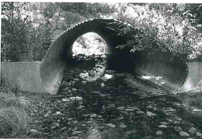
Figure 28. An arched pipe installed on a fish-bearing stream to minimize impacts on fish habitat and migration. Source: Keller and Sherar 2003.
