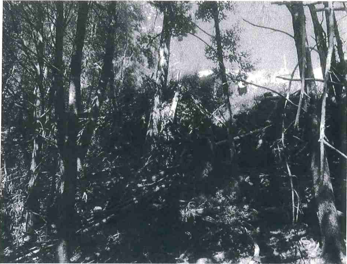
Picture 1: Perched and unstable fill material located at the southeastern corner of Cultivation Site A. Photo date 6-15-2018.
