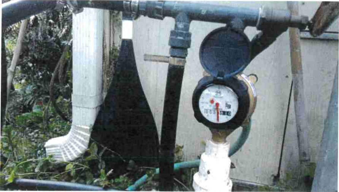
Photo 13. Water meter installed – 2/13/18
