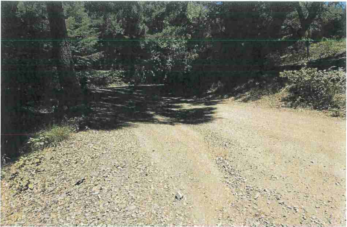
Photo looking up grade at the erosion at Site 11.
