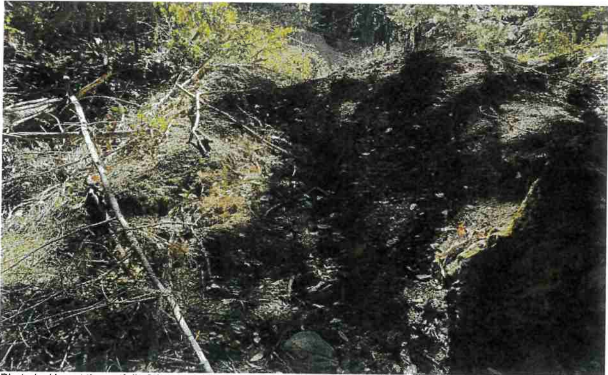
Photo looking at the outfall of the roadside ditch that starts at Site 14 and extends down to Site 13.
