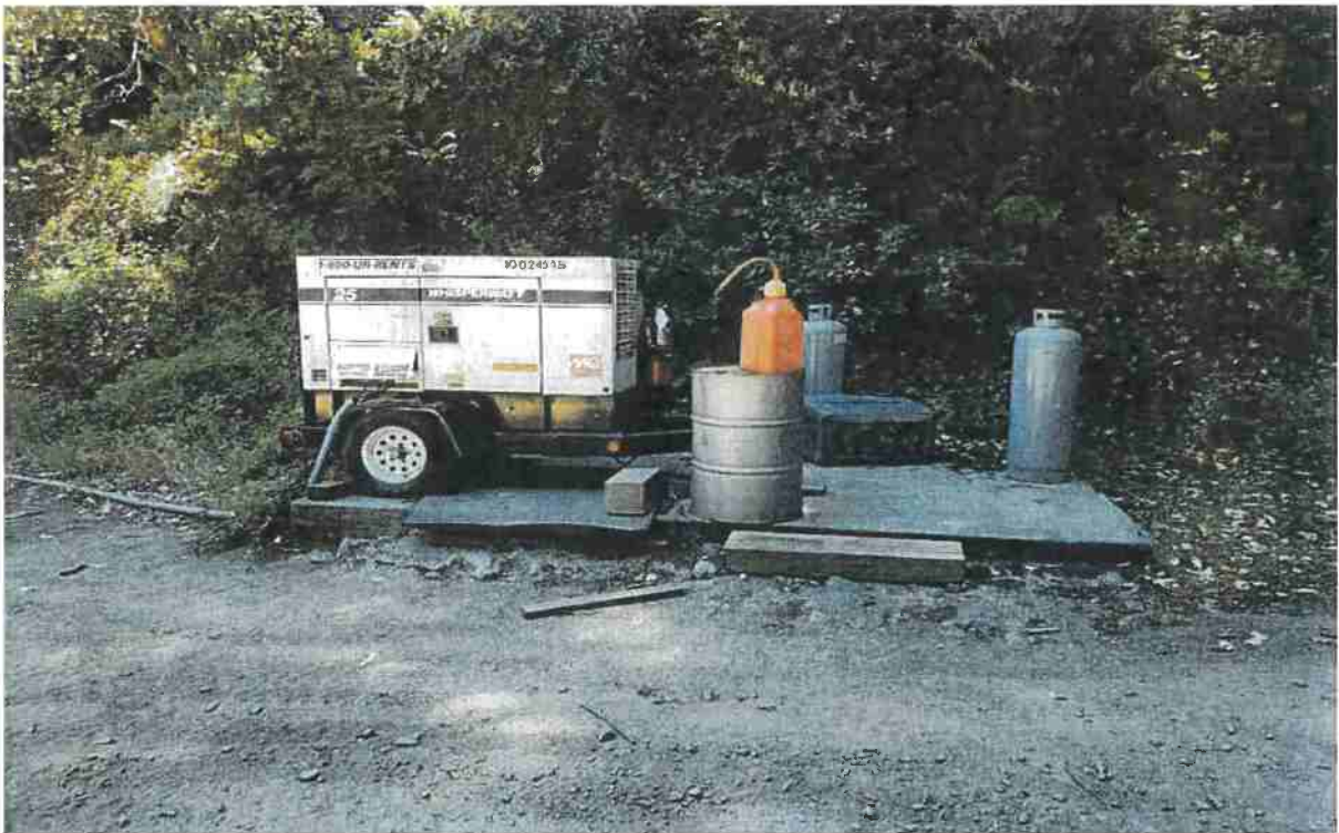
Photo looking at the uncovered diesel generator at Site 20.
