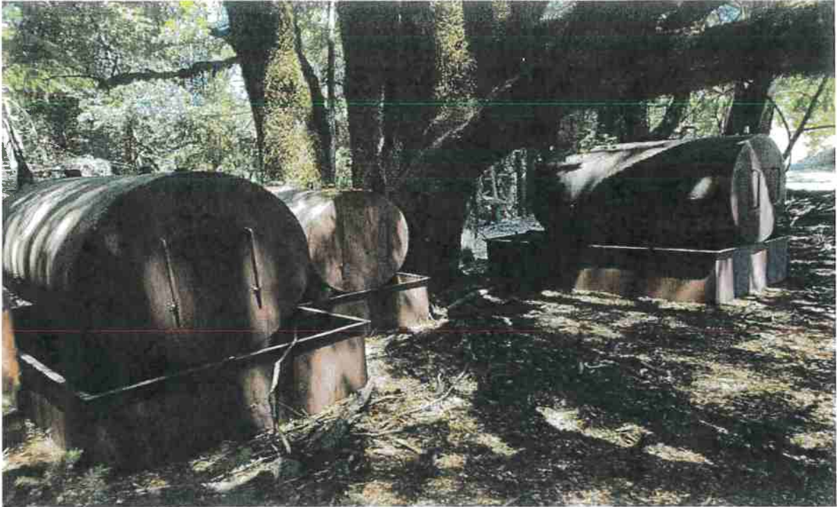
Photos looking at the petroleum tanks that don't have proper cover at Site 21.
