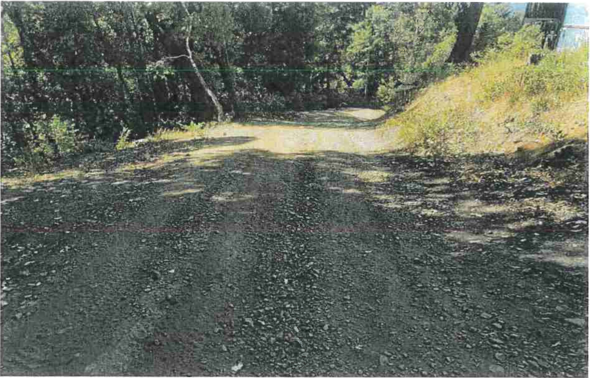
Photo looking down grade at the erosional gully at Site 03.
