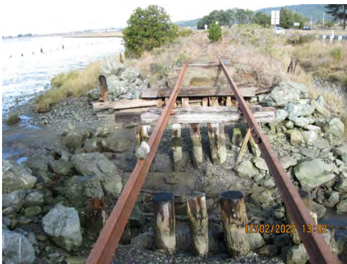
Railroad ties will need to be replaced in locations (example above) along the project alignment.
