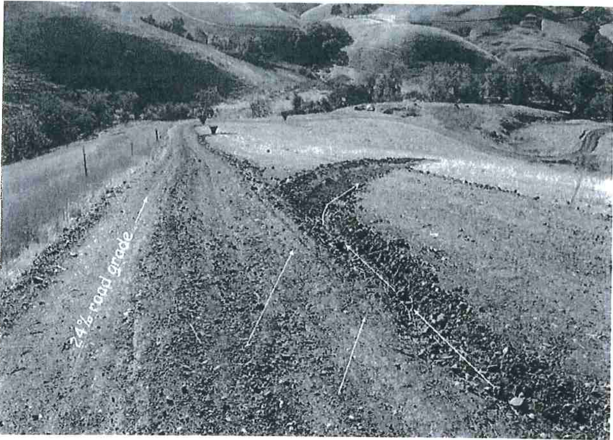
FIGURE 55. Steep roads that go straight up or down a hillside are very difficult to drain. This steep, fall line road developed a through cut cross section that was drained using lead out ditches to direct runoff off the road and onto the adjacent, vegetated hillside. The road was "outsloped" to drain runoff to the right side, and the lead out ditch was built slightly steeper than the road grade, to be self-cleaning. Four lead out ditches have been constructed at 100-foot intervals to the bottom of the hillside.
