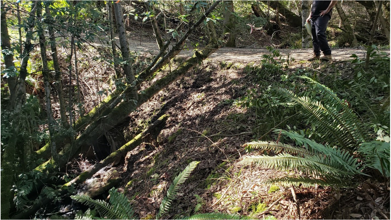
Photo looking southwest at the outlet of the watercourse crossing outlet at WQ-7 from PM 15.
