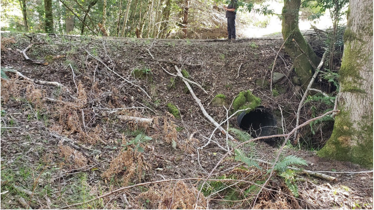
Photo looking southeast at the inlet of the watercourse crossing at WQ-7 from PM 14.
