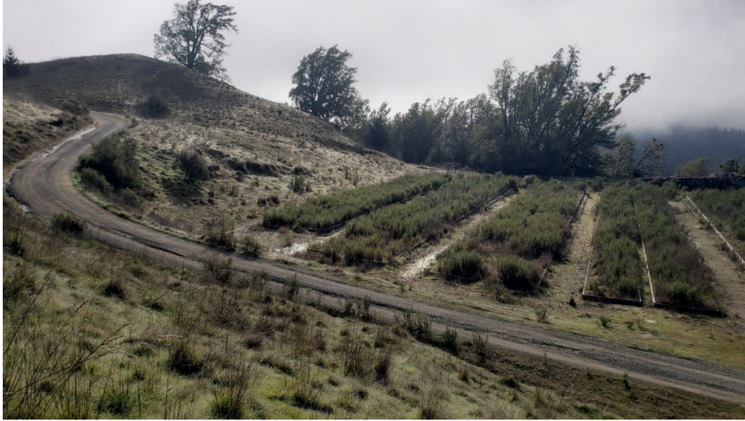
Photo looking southeast at the easternmost edge of WQ-1 grading area from PM 1. March 2 nd , 2021
