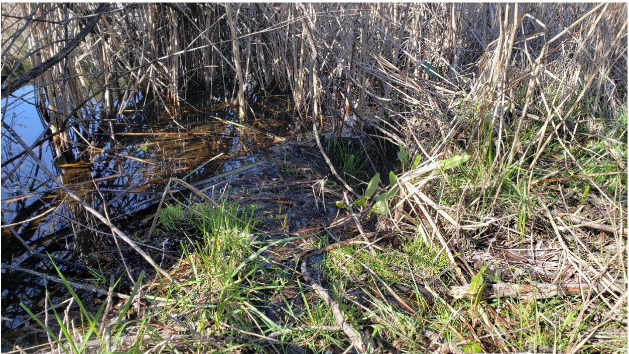
Photo looking northwest at the inlet of the impoundment overflow structure inlet at WQ-9. March 2 nd , 2021
