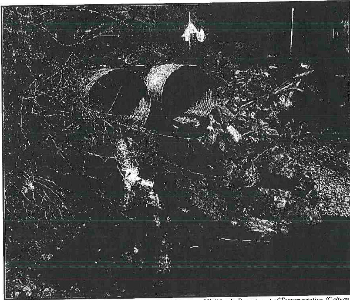
Figure 3. Rock armoring on shotgun culvert outlet. Photo Courtesy of California Department of Transportation (Caltrans).
