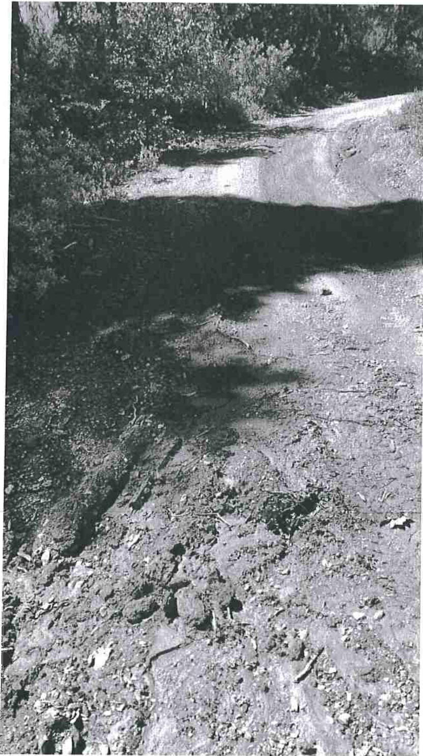
Road Point 2: Rilling is occurring on the road in the upper right hand corner. Owner will place a water bar above and maintain the rolling dip at the bottom so that water is adequately diverted. 7/12/2016
