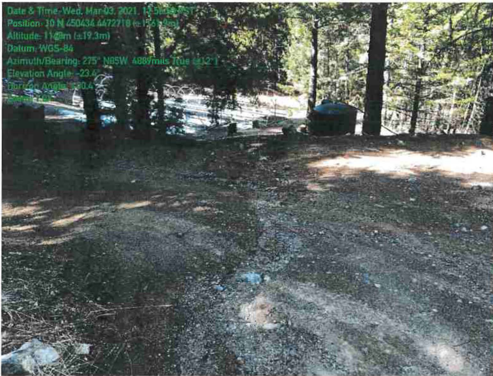
9.0 Erosion from Spring Across Road at Cultivation Site C
