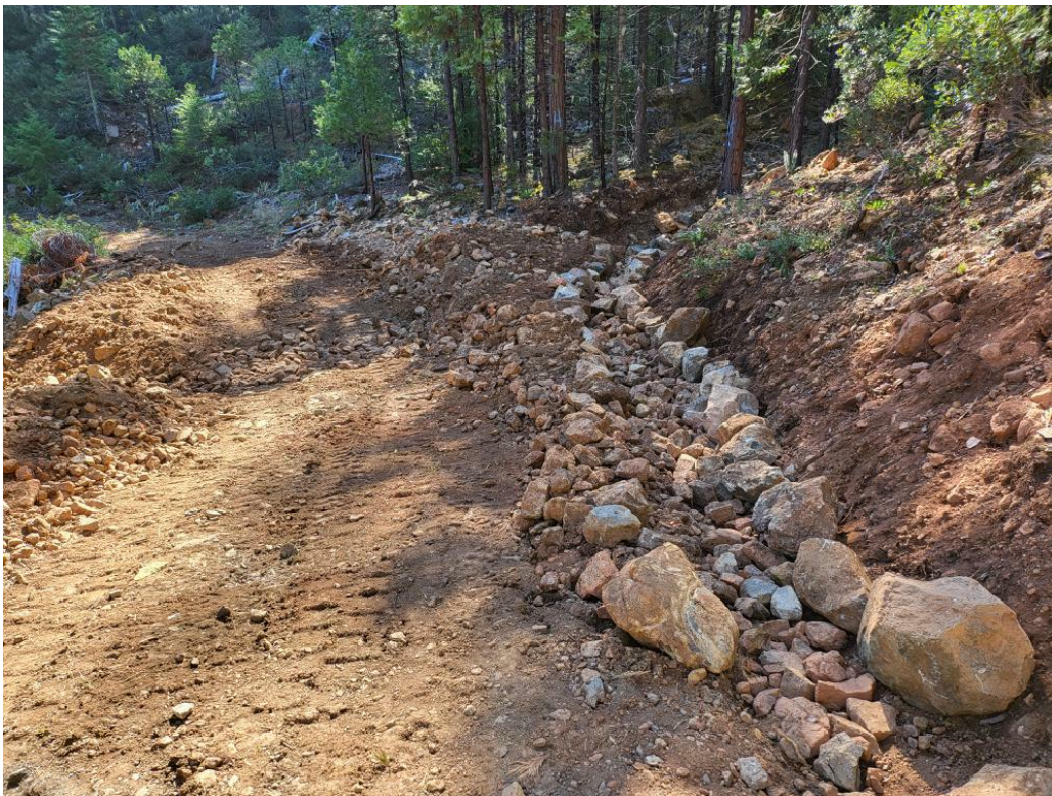
Figure 8: MP4 rocked ditch disconnecting spring from roadway.
