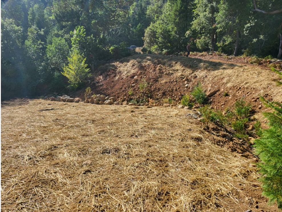
Figure 43: MP13 slope pulled back, stream restored with revegetation efforts currently succeeding as of 10/5/2022.
