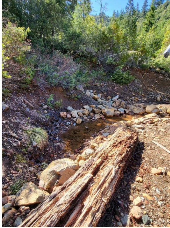
Figure 25: MP8 stream channel excavation to connect spring flow to Class II channel.
