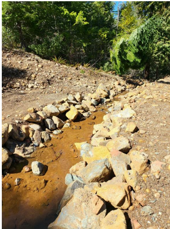
Figure 26: MP8 stream channel excavation to connect spring flow to Class II channel.
