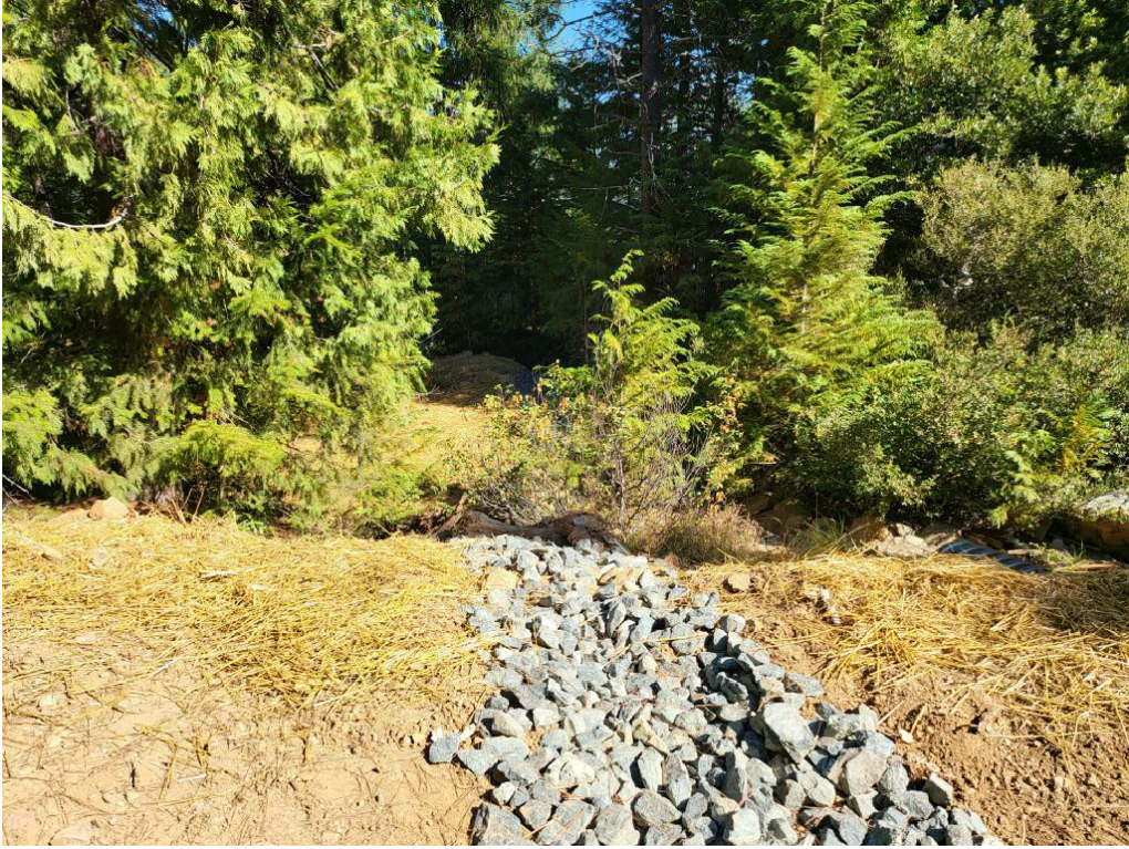
Figure 35: MP10 disconnected road surface from watercourse.
