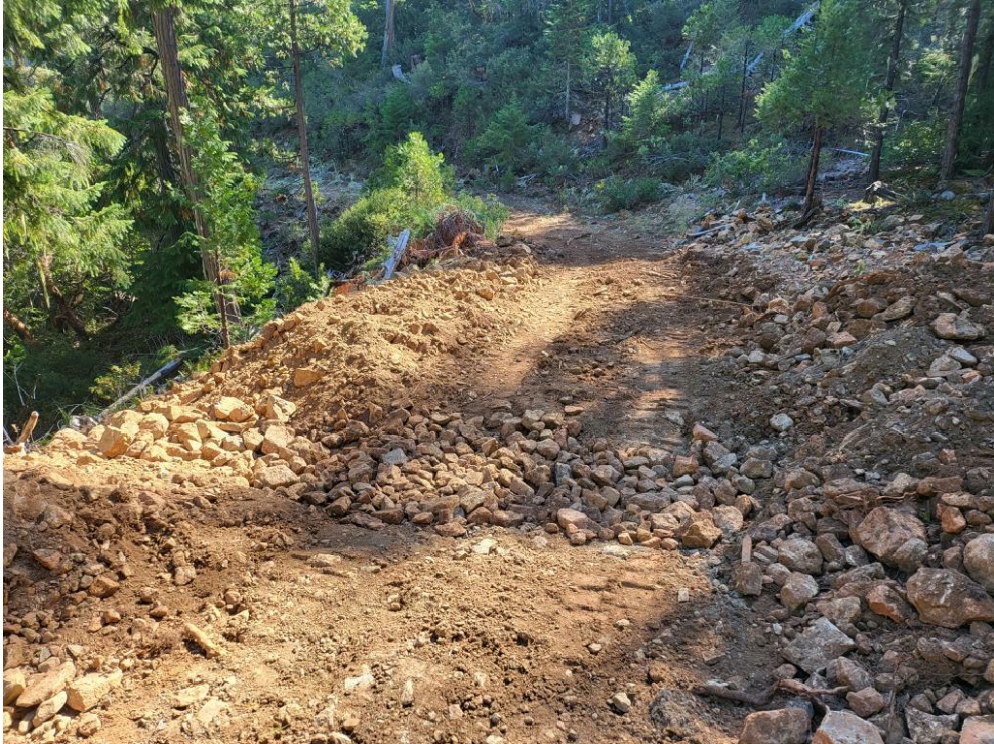
Figure 9: MP4 disconnected roadway.
