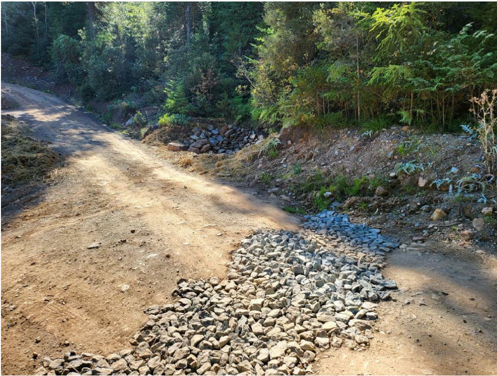
Figure 34: MP10 disconnected road surface from watercourse.
