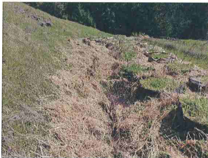
Figure 5: CA#6 view looking Northeast showing pots which require removal and revegetation of native grasses on the flat itself. Note potential drainage issues with water collecting alongside the uphill side of the graded flat.
