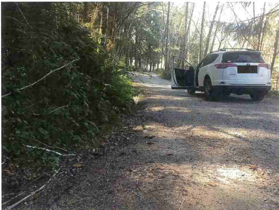
Figure 8: RP4. Outlet of 12' ditch relief culvert. Image facing west; toward Dows Prairie Rd.
