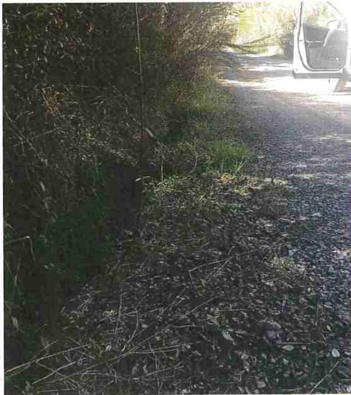
Figure 10: RP 5. Inlet of 12' ditch relief culvert. Image shown facing west; toward from Dows Prairie Rd.
