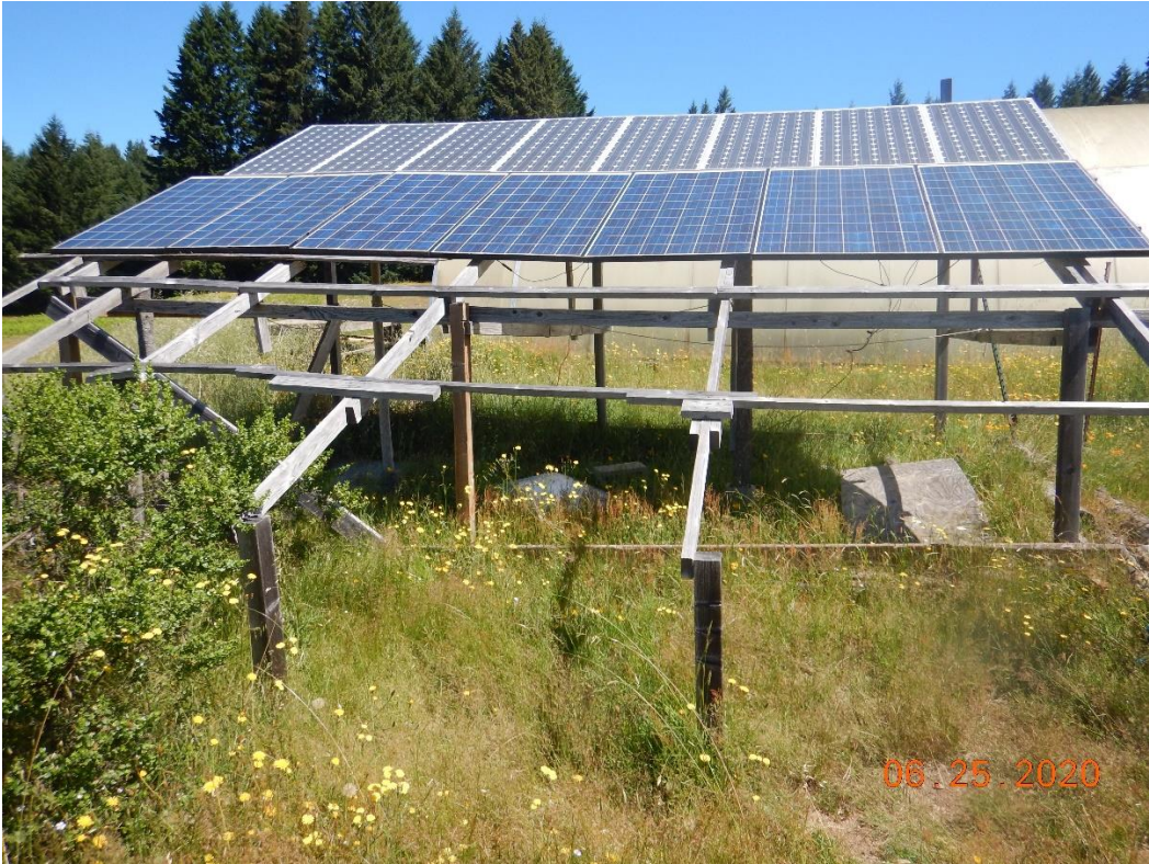
Photo 25. Alternate View of Solar Panels
