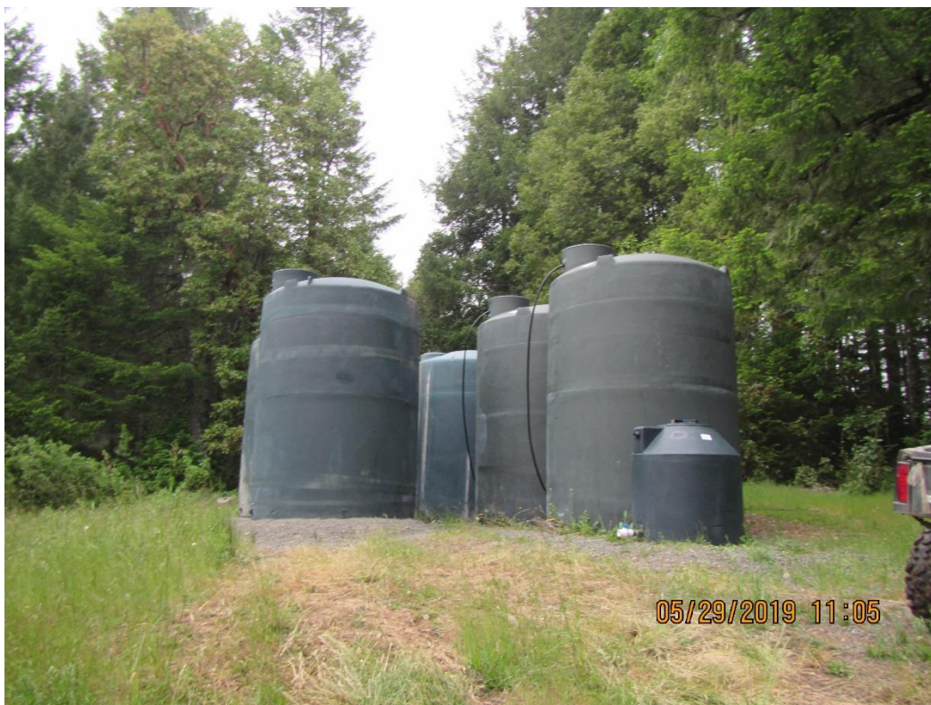
Photo 28. 24,000 Gallon Tank Farm
