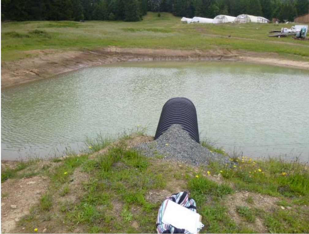
Photo 1. Project 1- Large pond, The inlet of the overflow culvert on the large pond.
