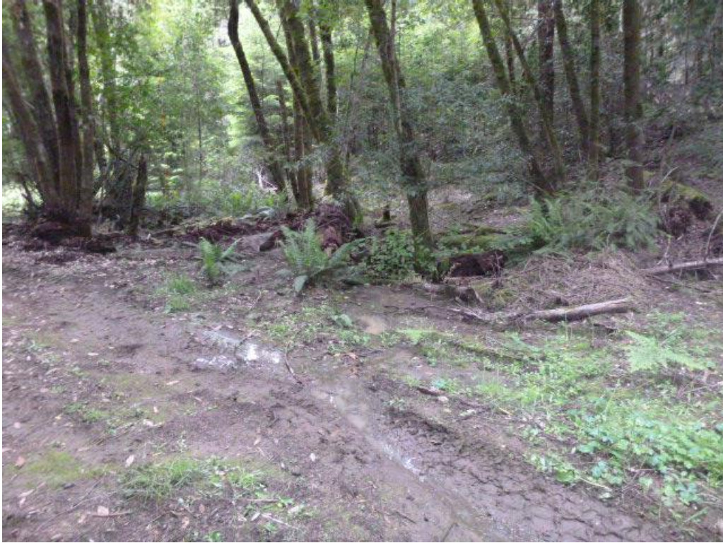
Photo 6. Additional Point 2 (Non-project). Captured surface flow exits the road and filters through the brush just above Additional Point 3, where it saturates the road surface before delivering to the head of the Class III watercourse.
