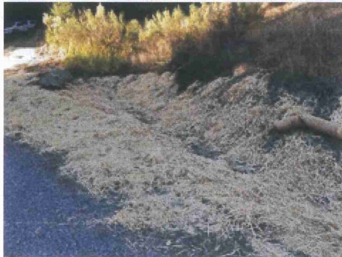
Picture 1 & 2: Crossing #1's inlet (top). Looking upstream from Crossing #1's inlet in the process of Erosion Control being applied. (bottom photo was provided by the Applicant on 11-12-2020.)
