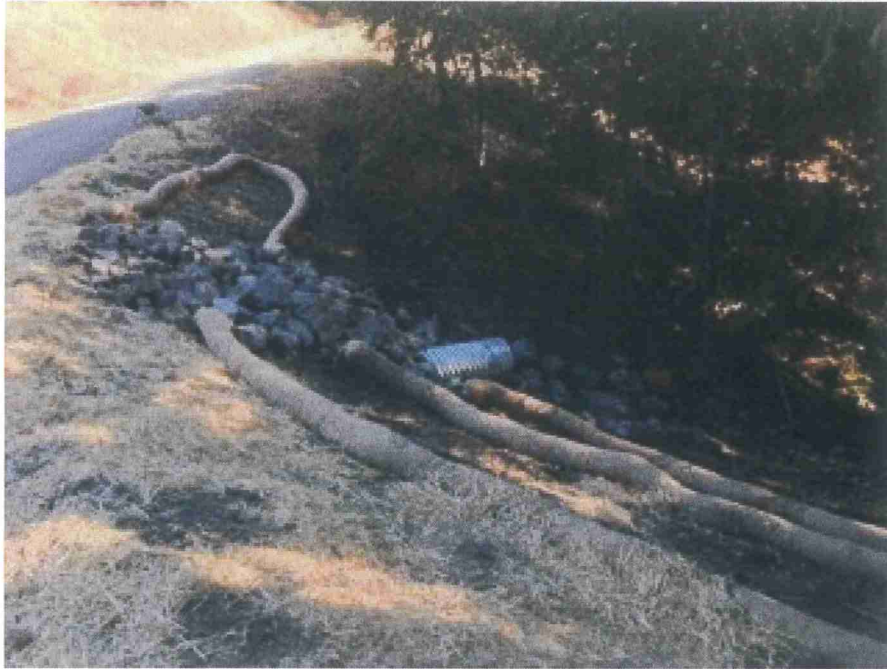
Picture 4: Crossing #1's outlet in the process of Erosion Control being applied. (photo was provided by the Applicant on 11-12-2020).
