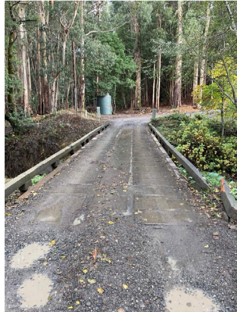
Image 2. Single-Lane Bridge (looking west). Note large turnout at opposite end of bridge.
