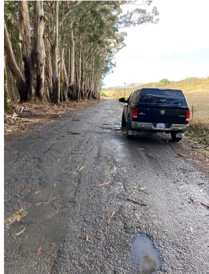
Image 4. Representative of RS2 conditions (looking west). Details asphalt surface, 20'+ average road width, shoulders, turnouts, crowned geometry with fair drainage, average slopes <5% - max <12%.
