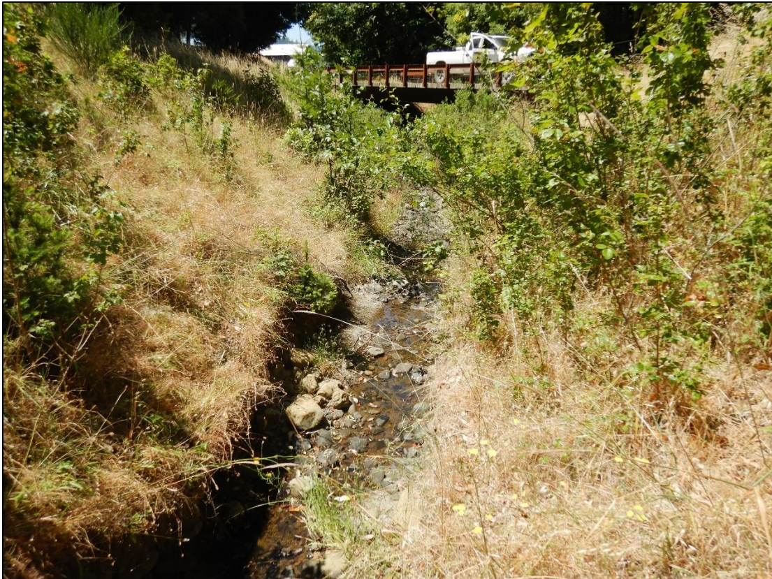
Photo 2. The unnamed Class II watercourse on APN: 105-101-011. Photo taken from the stream looking down stream towards the west facing the bridge.
