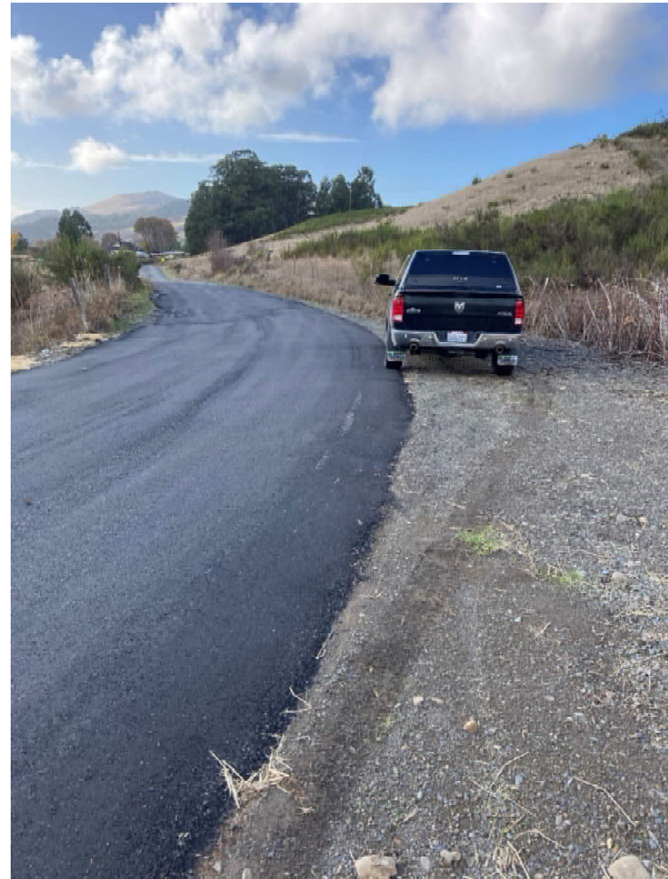
Image 6. Representative of RS2 conditions (looking west). Details asphalt surface, 20'+ average road width, shoulders, turnouts, crowned geometry with fair drainage, average slopes <5%.
