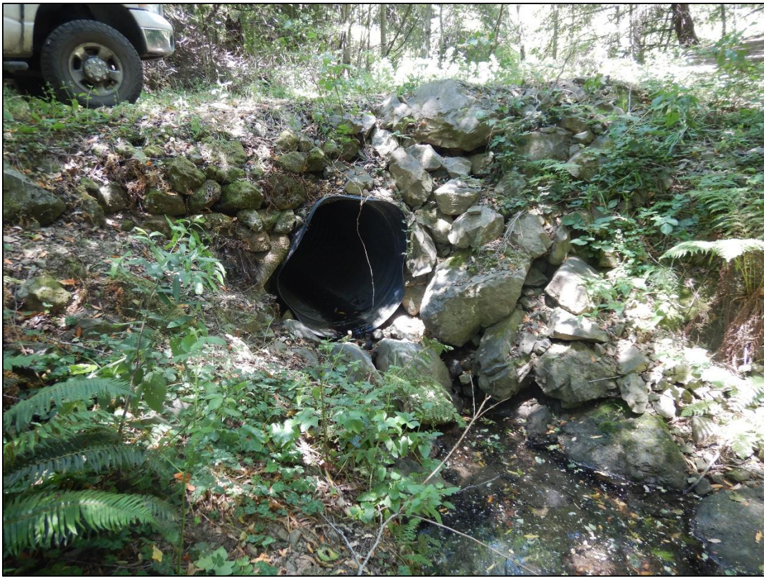
Photo 7. The culvert and stream crossing over the unnamed Class II watercourse in the northwestern portion of APN: 105-101-011. This may need to be replaced in order to comply with regulation sizing (Map 2).
