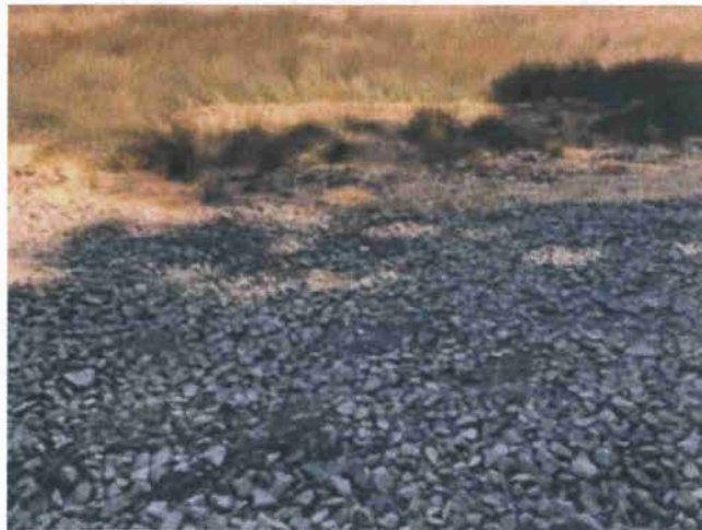
Picture 11 & 12: Existing Rock Ford at Crossing #1 at the head of a Class III watercourse. Photos date 8-13-2018.
