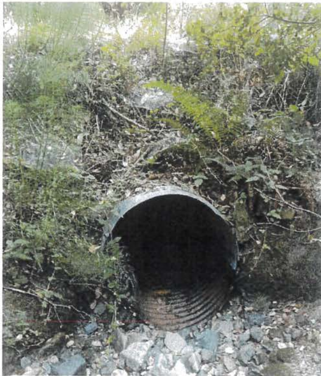
Photo looking at the inlet of the watercourser crossing at Site 22. Photo date 6-11-2016
