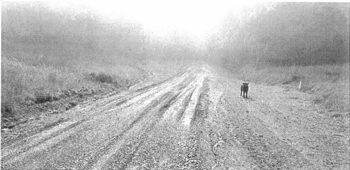
Photo looking downgrade at Site 10. Note road rutting and rock surfacing. Additional competent rock surfacing (4" – 6" crushed angular) will be required here.
