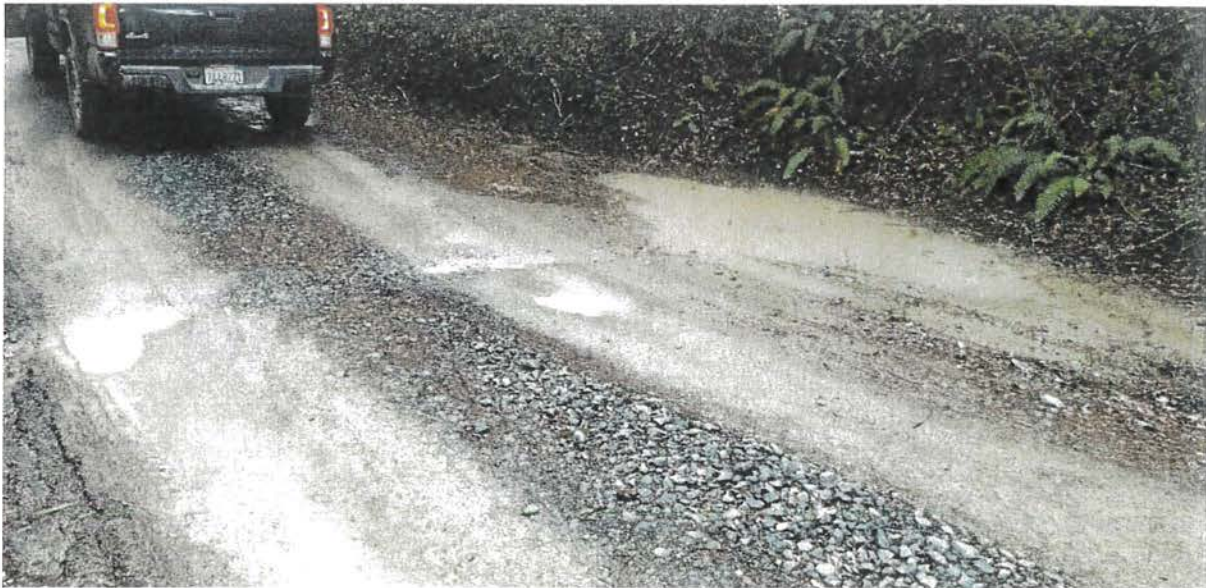
Photo looking at Site 05. A 15" diameter ditch relief culvert shall be installed here.
