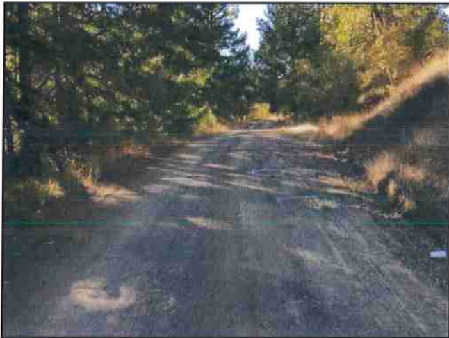
Photo #207 River Rd Looking West @ Drainage Issue
