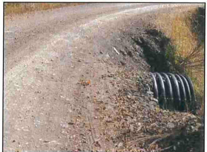
Photo #280 River Rd Looking @ 24" Culvert Out w/ Drainage Issue & Erosion Issues
