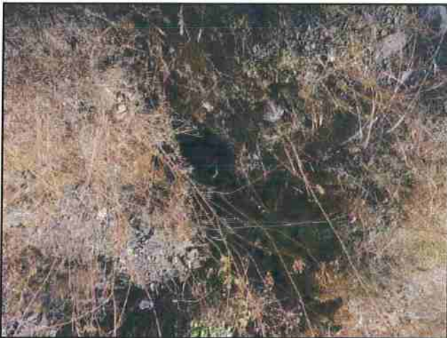
Photo #111 River Rd Looking @ Partially Clogged 36" Culvert In
