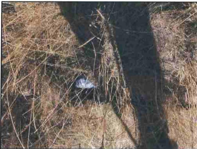
Photo #393 River Rd Partially Clogged 24" Culvert In (Photo 389 24" Culvert Out)
