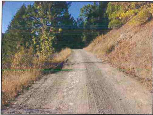
Photo #211 River Rd Looking NW @ Drainage Issue
