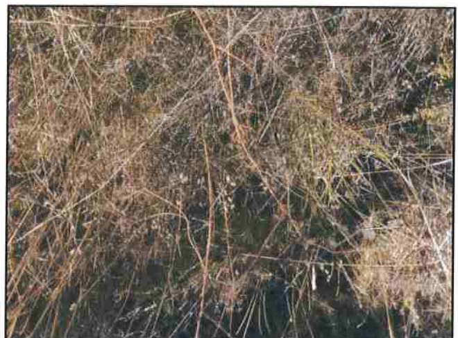
Photo #256 River Rd Clogged Culvert In (Size Unknow)
