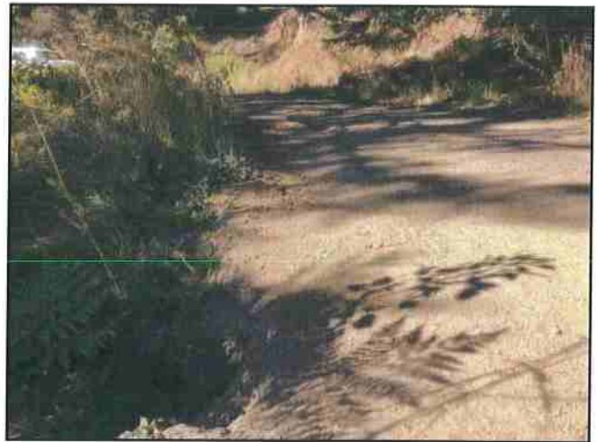
Photo #446 River Rd @ Curve w/ Turnout Looking NW @ Erosion Issue
