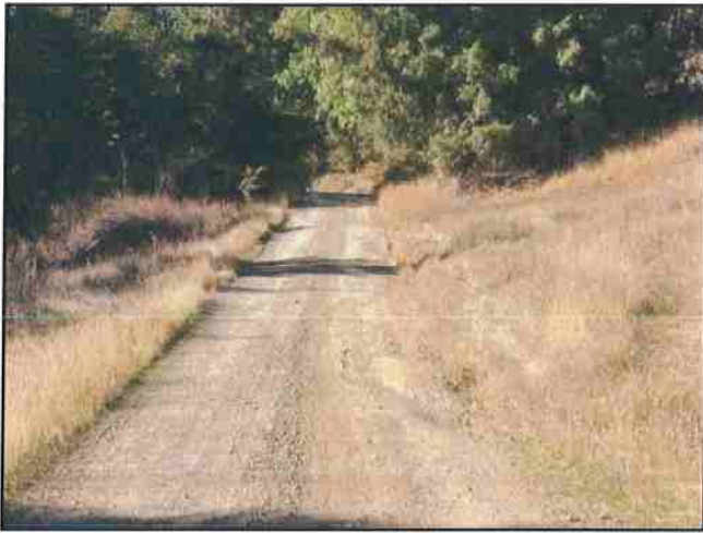
Photo #325 River Rd Looking NE @ Hillside Slip Creating Drainage Issue and Rutting
