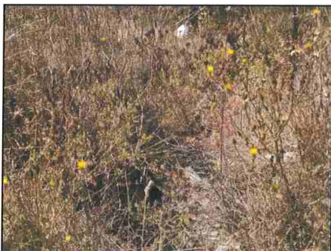
Photo #257 River Rd Clogged Culvert Out (Size Unknow)
