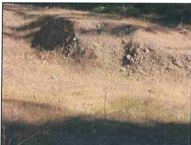
Photo #311 River Rd Looking @ Hillside Slip
