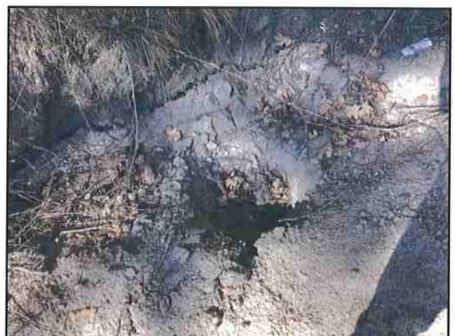
Photo #114 River Rd Looking @ Erosion Issue
