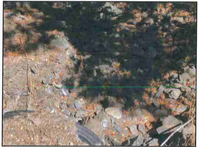
Photo #278 River Rd Looking @ Partially Clogged 24" Culvert In
