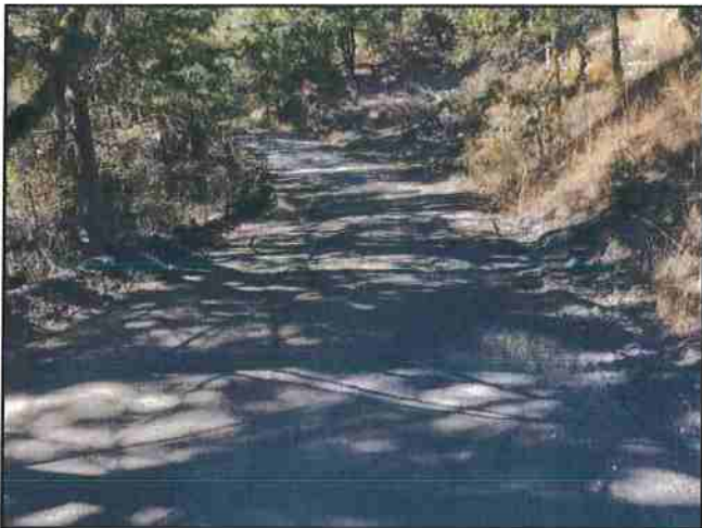
Photo #99 River Rd Looking NW @ Drainage Problem
