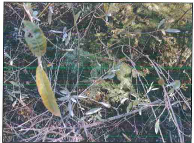
Photo #164 River Rd Looking @ Partially Clogged 24" Culvert Out
