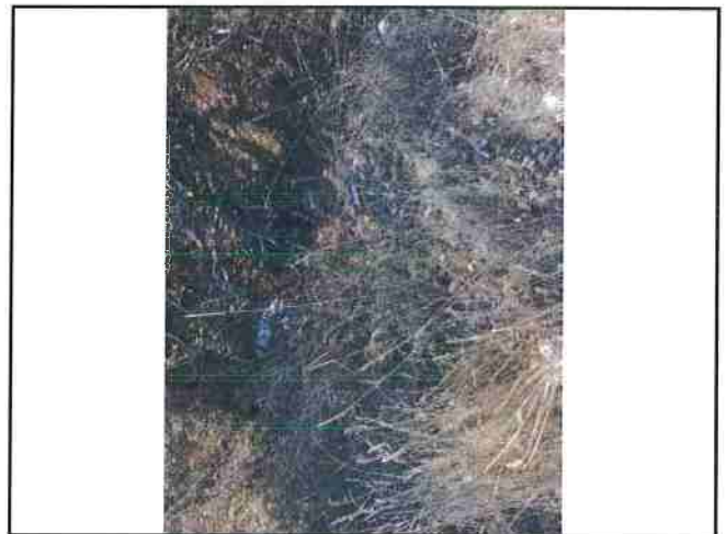
Photo #28 River Rd 12" Clogged 12" Culvert Out
