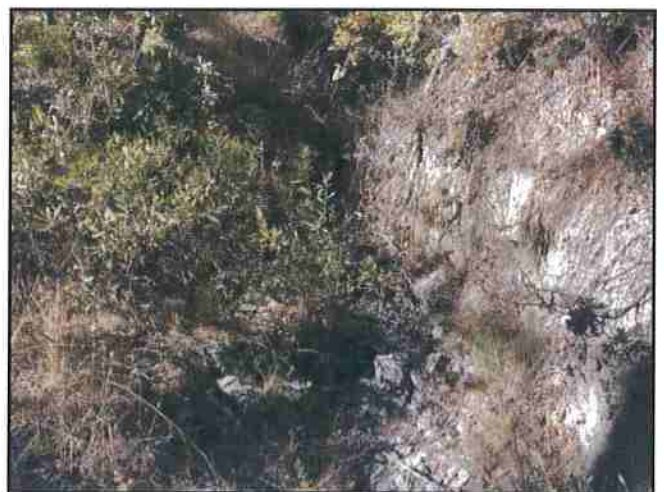
Photo #90 River Rd Looking @ Clogged 24" Culvert In
