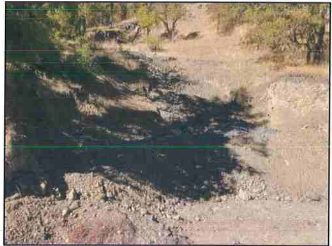
Photo #56 River Rd Looking @ Slide
