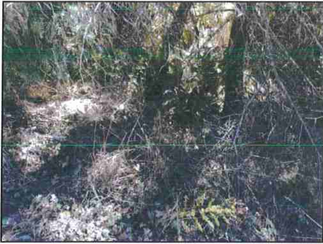
Photo #61 River Rd Looking @ Clogged Culvert In
