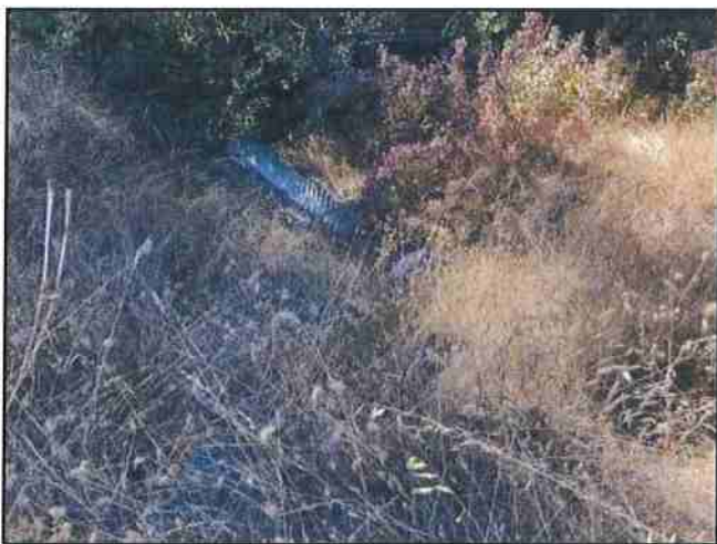
Photo #389 River Rd 24" Culvert Out
