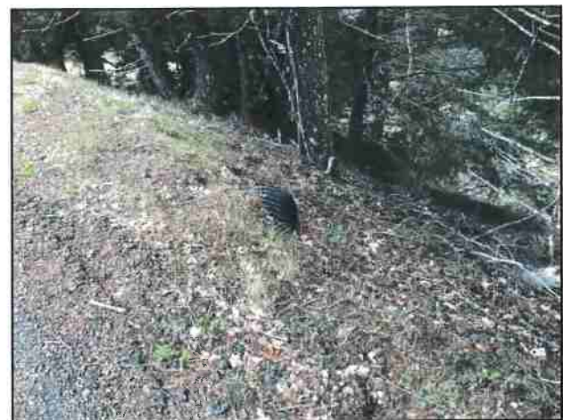
Photo #126 Private Access Rd Looking @ Partially Clogged 18" Culvert Out (Size Unknown)
