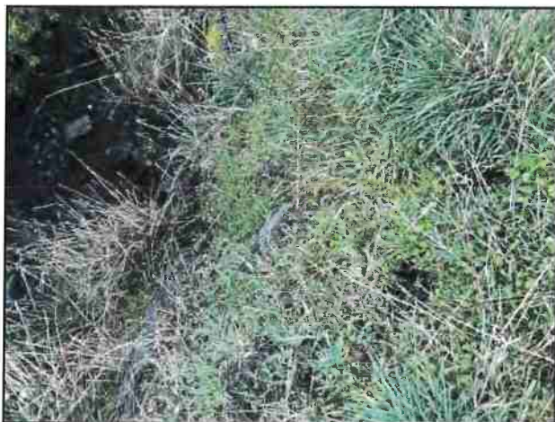
Photo #83 Private Access Rd Looking @ Partially Clogged 18" Culvert Out
