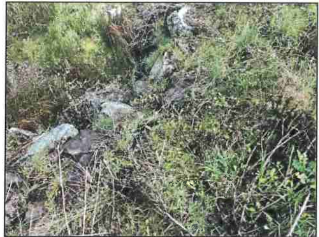
Photo #116 Private Access Rd Looking @ Partially Clogged Culvert In (Size Unknown)
