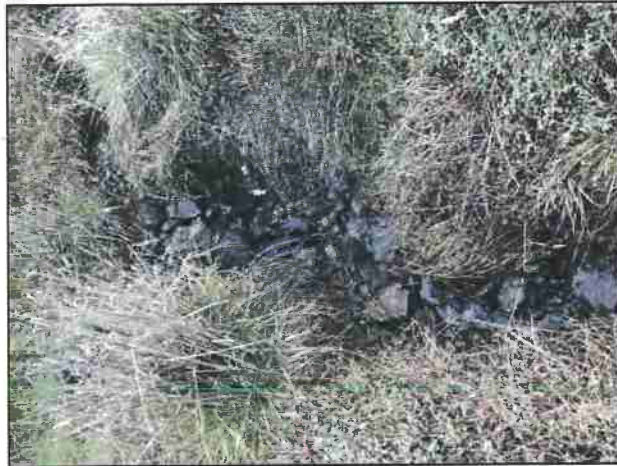
Photo #63 Private Access Rd Looking @ Partially Clogged 18" Culvert In
