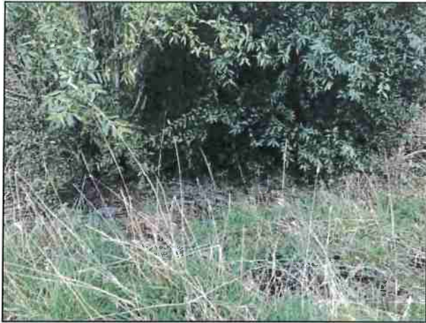
Photo #115 Private Access Rd Looking @ Partially Clogged Culvert Out (Size Unknown)
