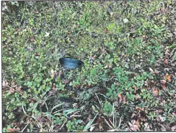
Photo #37 Private Access Rd Looking @ Partially 12" Culvert In
