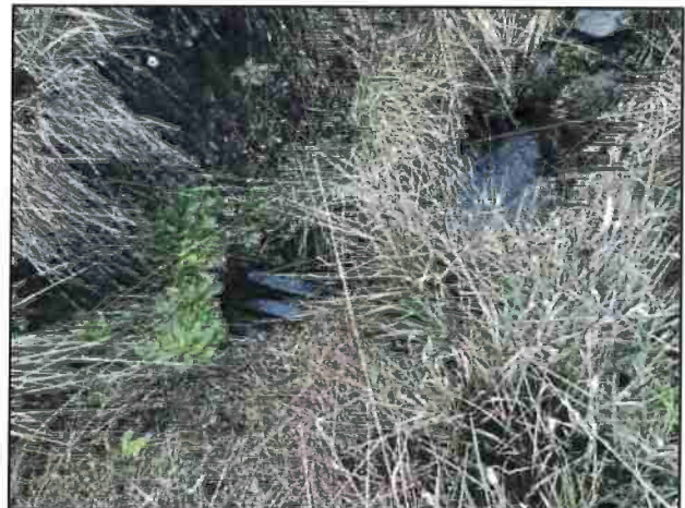
Photo #82 Private Access Rd Looking @ Partially Clogged 18" Culvert In
