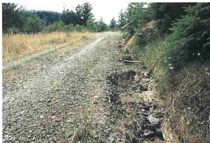
Figure 20. Eroding inboard ditch on an in-sloped road. This is a symptom of inadequate cross drains for conveying ditch flow across the road. Photo: Richard Harris.
