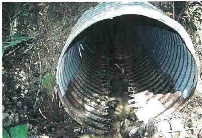
Figure 17. Culvert with rusted bottom and breakage caused by sediment. Photo: Angela Wilson, Central Valley Regional Water Quality Control Board.
