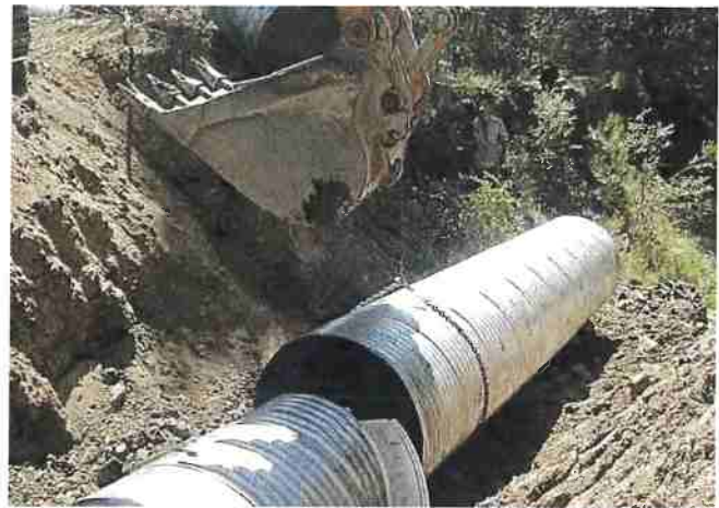
Figure 30. Installation of a new culvert after the old one was excavated. Photo: Jared Gerstein.
