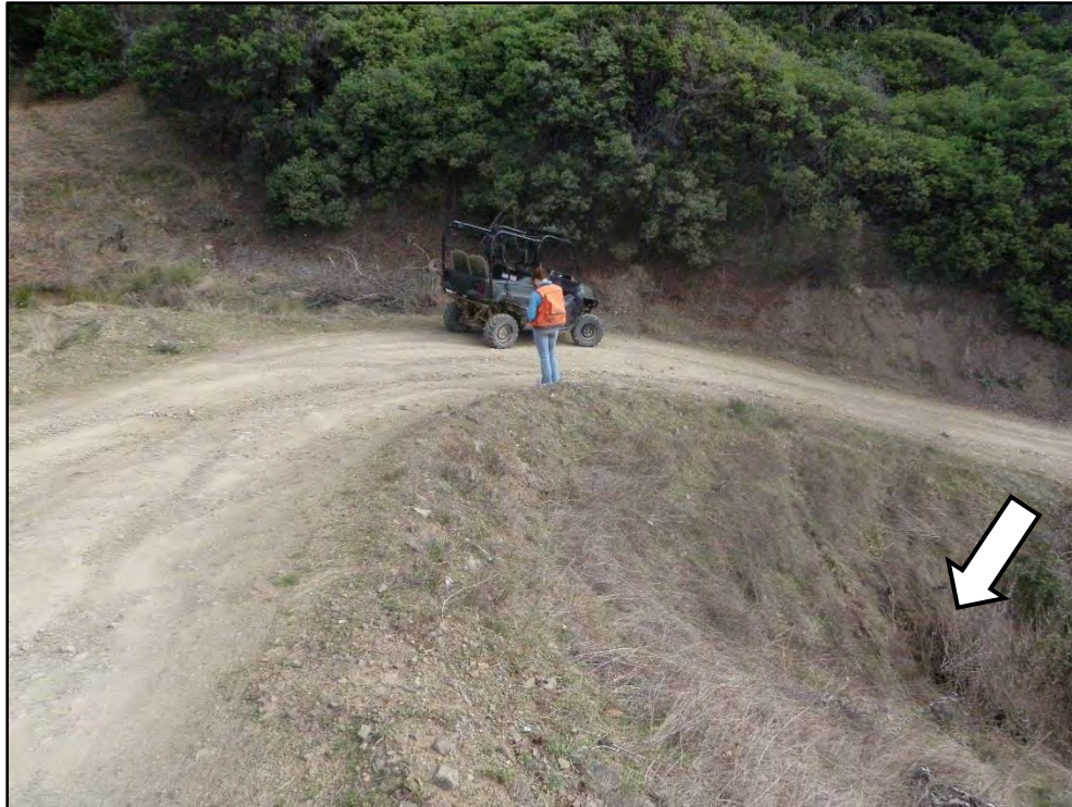
Photo 5 – Project #2, View of SC #1 from the right road approach. Note the culvert outlet (arrow) set high in the outboard fill face.
