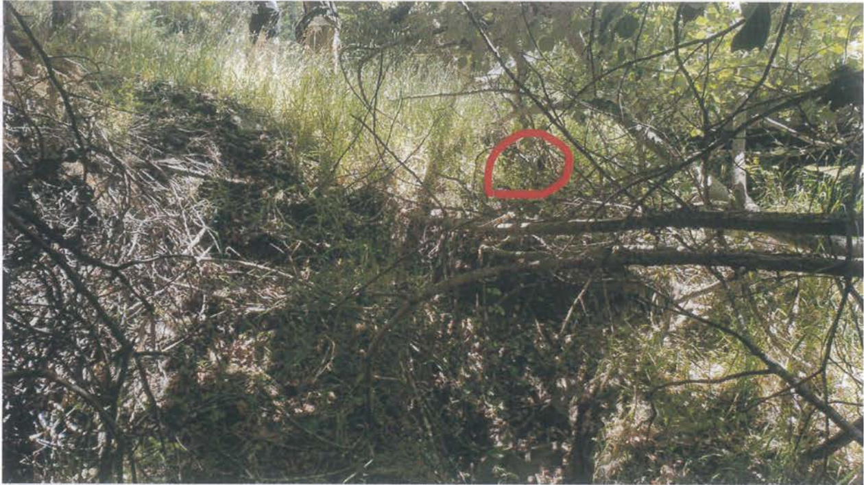
Site 35. Looking at the outlet(circled). The culvert upgrade will re-align the watercourse to its original channel, which will require the outlet to be placed in the lower left of the photo.
