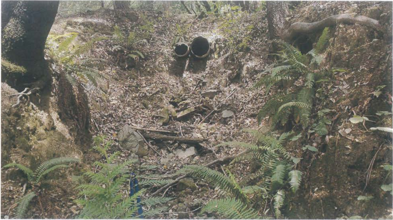
Outlet of watercourse crossing at Site 23. The blue flag represents the proposed outlet of culvert upgrade.
