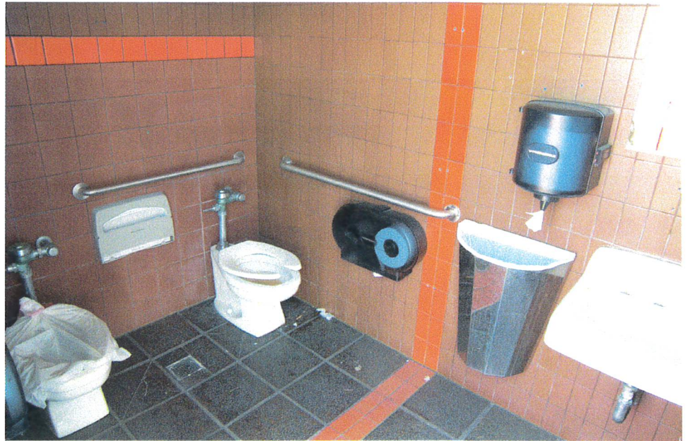
Southern restroom which has been enlarged and updated to partially comply with ADA.
