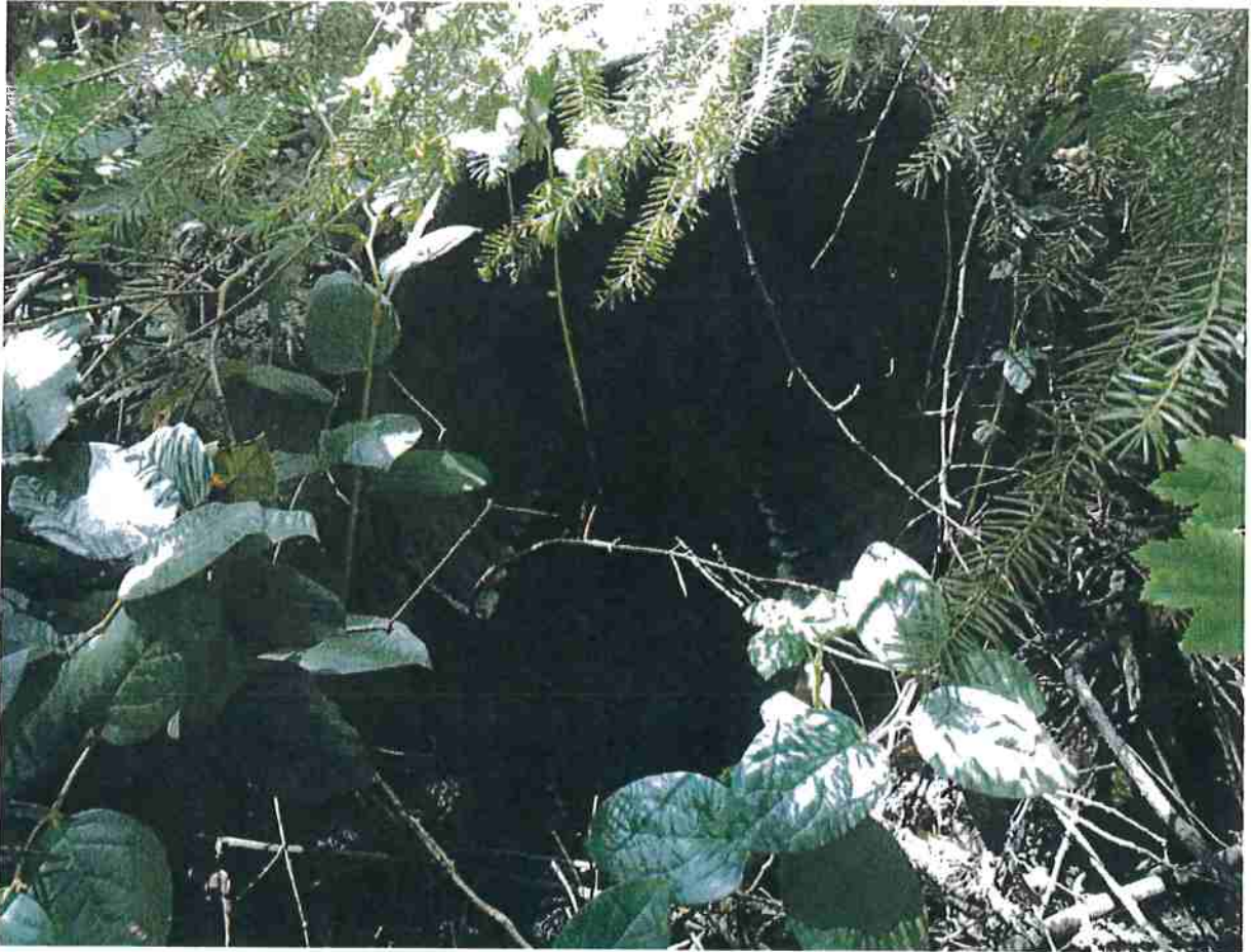
Photo #2: This is an image of the culvert outlet at Stream Crossing #1 (SC 1), which is positioned slightly above the natural stream channel. The Discharger shall rock armor the outlet of this culvert per the attached specifications. Photo Date: 06/06/2017.
