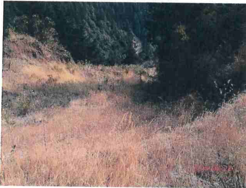
Photo 2-5C: Outboard landing fillslope failure looking downslope from near the right center of feature. Note natural revegetation of bare soil areas as compared to 2016 photos. (Photo taken August 22, 2018).
