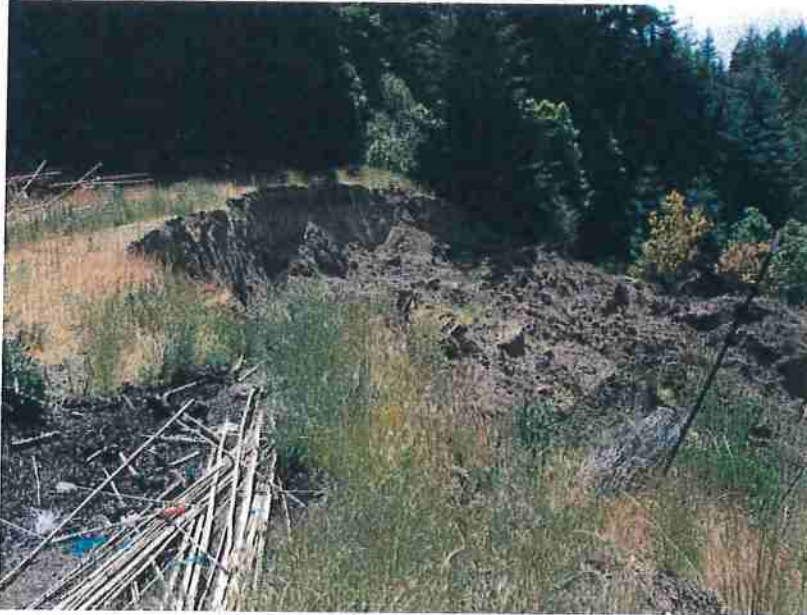
Photo 1-5A: Outboard landing fillslope failure looking southeast from the right edge of head scarp. (Photo taken June 13, 2016).
