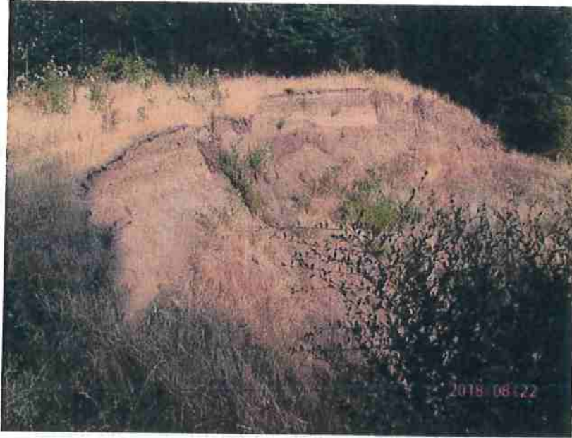
Photo 2-5B: Outboard landing fillslope failure looking southeast from the right edge of landslide head scarp. (Photo taken August 22, 2018).
