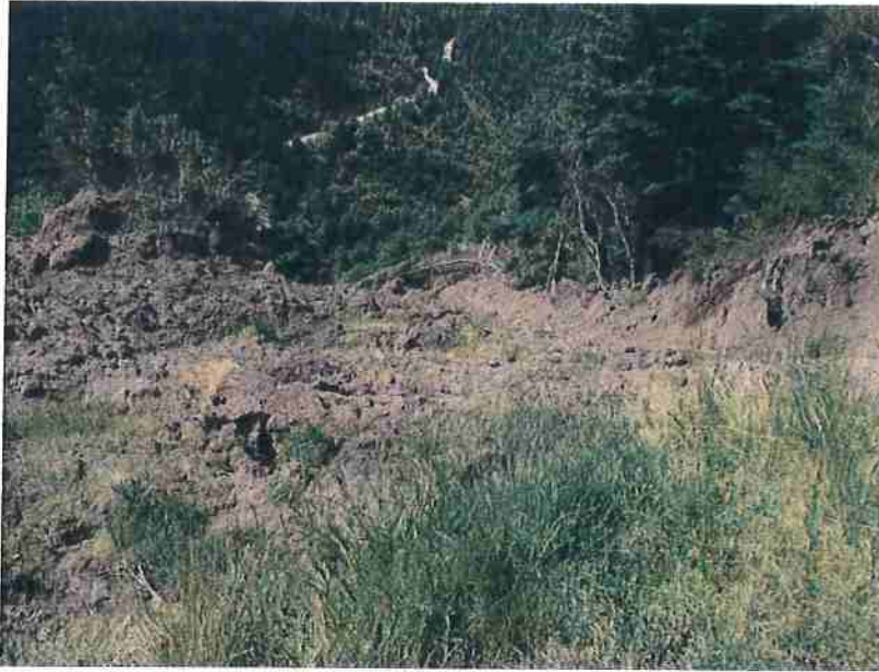
Photo 1-5C: Outboard landing fillslope failure looking downslope from near the center of feature. (Photo taken June 13, 2016).
