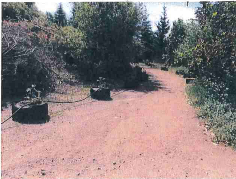
Photo 4-5A: View of the northern portion of the lower road bench at CA #5 looking south in the direction of the outboard fillslope failure (not shown) from the intersection with Access Road #8. (Photo taken June 13, 2016)
