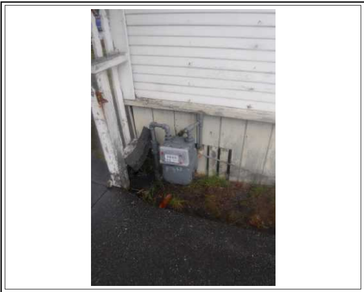
Gas Meter Utility
