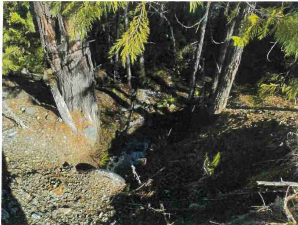
Outlet of MP7, functional
