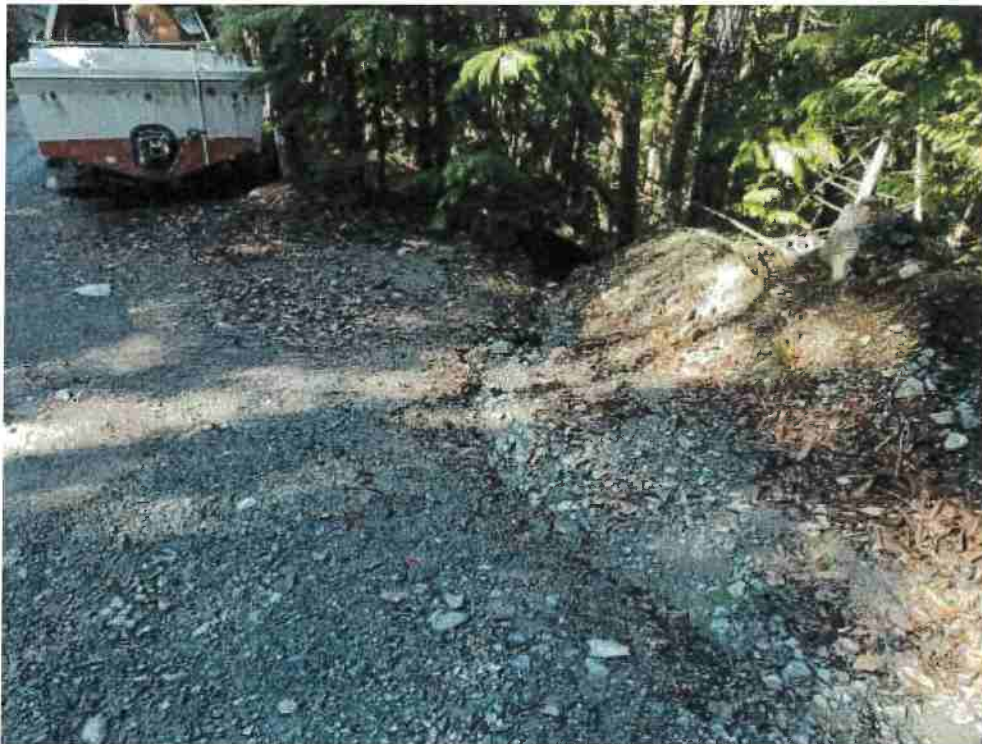
Road surface drains to MP20 with some erosion of road prism
