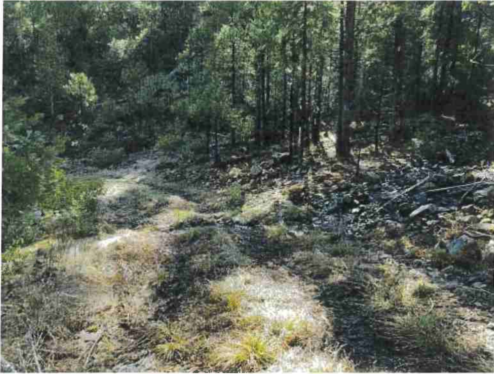
Minor erosion of roadbed but naturally rocky substrate maintains stability
