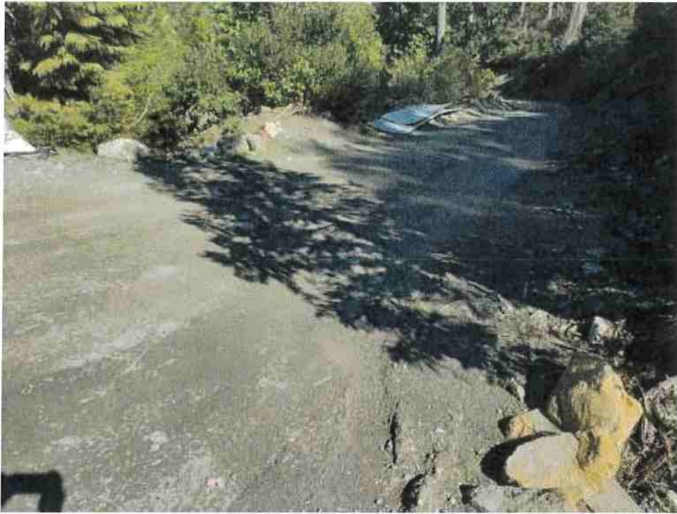
Little erosion at MP19, maybe some overtopping at an earlier date
