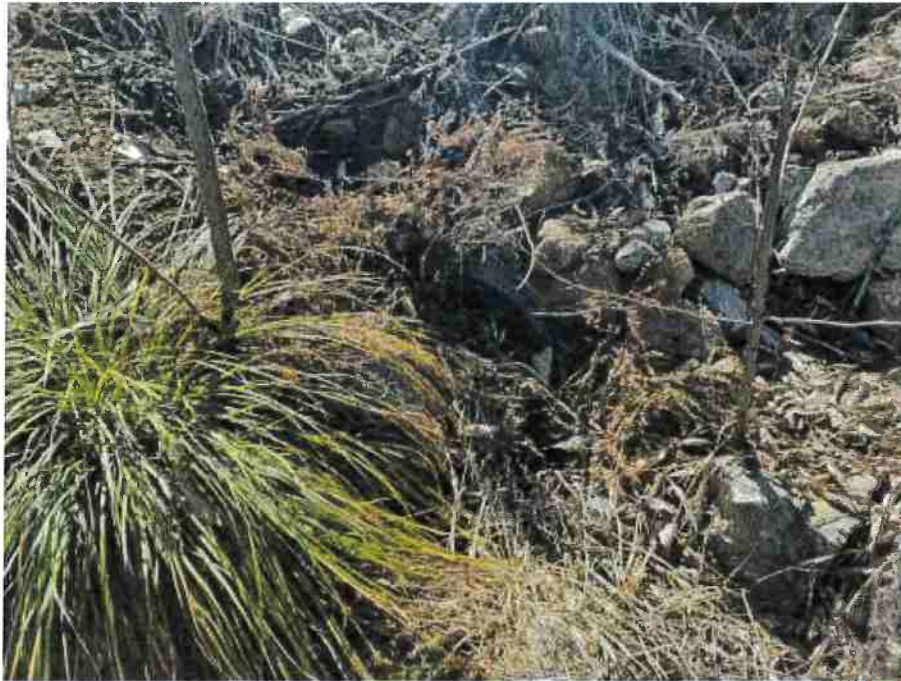
Culvert outlet functioning though partially obstructed
