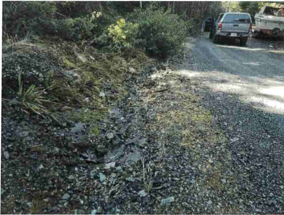
Sediment deposition in inboard ditch that diverts flow at MP20
