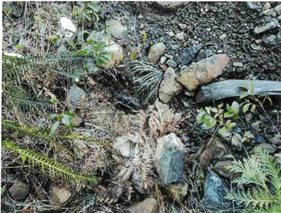
Partially clogged inlet, still functional
