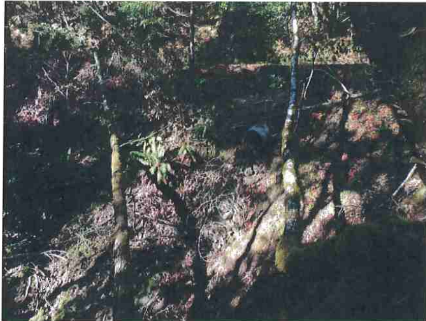
Photo 6. Stream Crossing #3, view of culvert outlet placed high in the fill with 3-4 feet of barrel projection. Culvert is set nearly to the natural grade of the stream channel, and outlets water onto rock armor before plunging approximately 4 foot below to re-enter channel.
