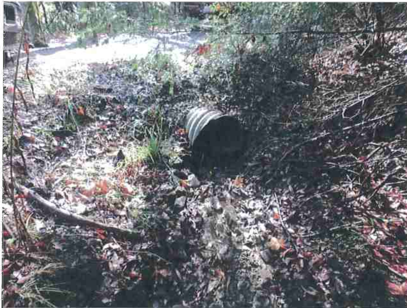
Photo 9. Stream Crossing #4, view of Stream channel entering culvert inlet. Culvert receives sediment contribution from nearby quarry which drains to this crossing during rainfall events.
