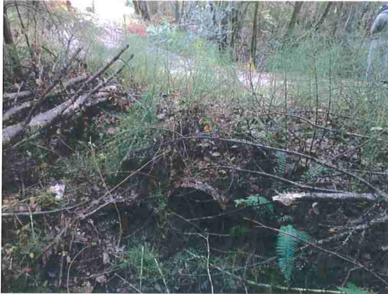
Photo 2. Stream Crossing #1, downstream view of 24-inch diameter culvert inlet and heavily wooded channel. Culvert was not plugged or impeded by woody debris at time of site visit.
