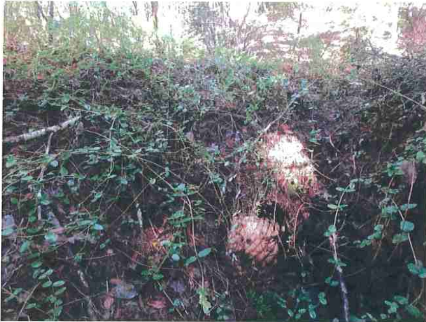
Photo 4. Stream Crossing #2, view of culvert outlet placed short and high in the fill. Culvert is not properly aligned with the natural grade of the stream channel, and outlets water onto rock and fill material.
