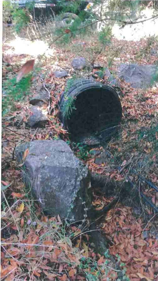
Photo 16. Stream Crossing #7, view of 24-in diameter HDPE culvert outlet. Culvert is properly aligned with the natural grade of the stream channel, and is resting on large roots of nearby conifer.
