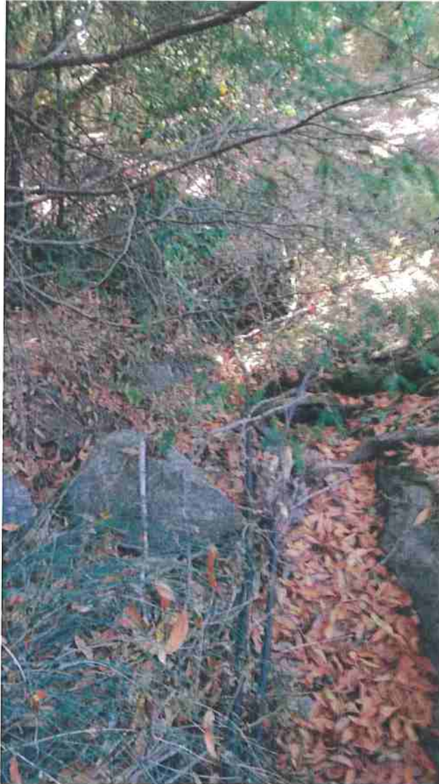
Photo 17. Stream Crossing #7, downstream view of channel below culvert outlet. Significant erosion of the bed and banks was not noted.
