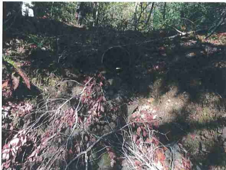
Photo 7. Stream Crossing #3, upstream view of culvert outlet placed short and high in the fill. Significant erosion was not noted at the outlet.
