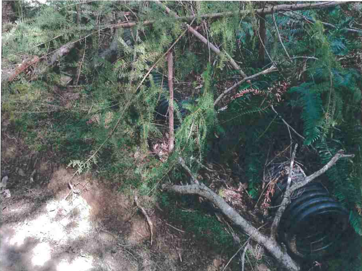
Photo 28. Pond #1-View of Pond #1 spillway culvert outlet. Culvert outlets onto a legacy skid road, which has gullied for several hundred feet down the road before laying out across a natural flat and another legacy haul road.
