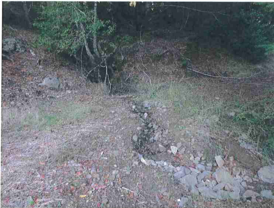
Photo 22. Stream Crossing #9, upstream view of gully incised into a legacy road resulting from a buried culvert inlet. A Class II stream still flows through the 12-inch diameter plastic culvert outlet, and overtops during high flow events following the gully path back into the channel.
