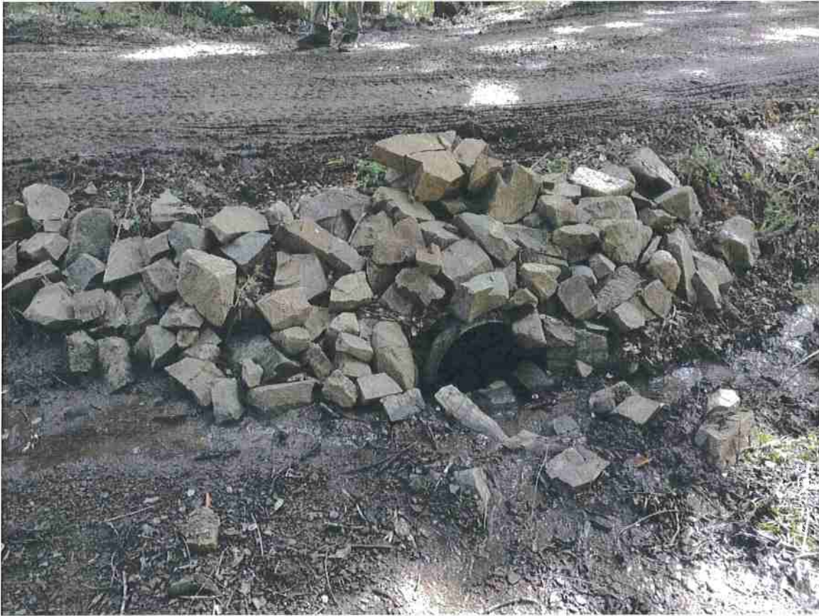
Photo 13. Stream Crossing #6, view of 16-inch diameter HDPE culvert inlet. IBF is armored with 6" plus angular rock, inlet is partially plugged with aggraded sediment and fines.
