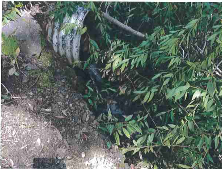
Photo 1. Stream Crossing #1, view of 24-inch diameter culvert outlet. Flow plunges approximately 2 feet before re-entering natural channel. Minor erosion of outboard fill slope noted.
