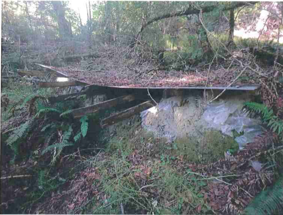
Photo 32. Pond #4 (Guerrilla Pond #2) - View of the concrete embankments, wooden frame and sheet metal roofing of the legacy Guerrilla Pond #2.
