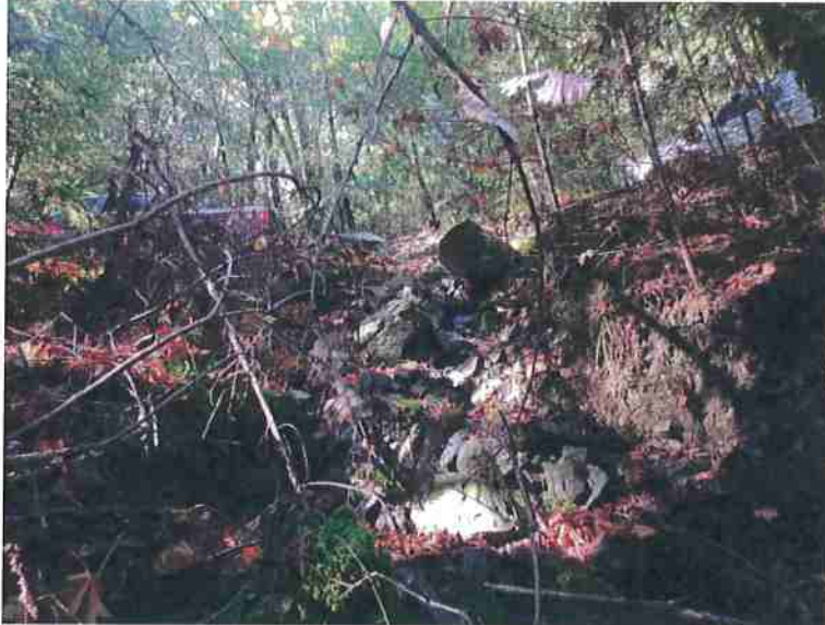
Photo 10. Stream Crossing #4, view of watercourse exiting culvert outlet. Culvert is placed short and high in the fill. Flow path takes an approximate 2-foot plunge at the outlet.
