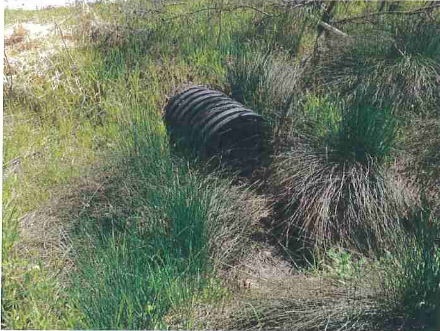
Photo 19. Stream Crossing #8, view of 18-inch diameter culvert. Culvert is properly aligned with the natural grade of the stream channel.
