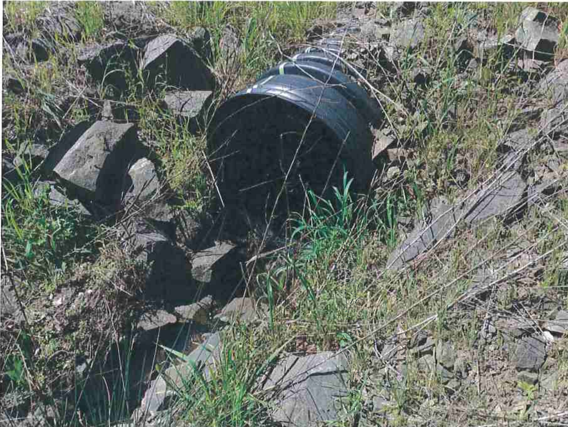
Photo 21. Stream Crossing #8, view of outlet. Stream flow exits culvert onto 6" minus angular rock apron.
