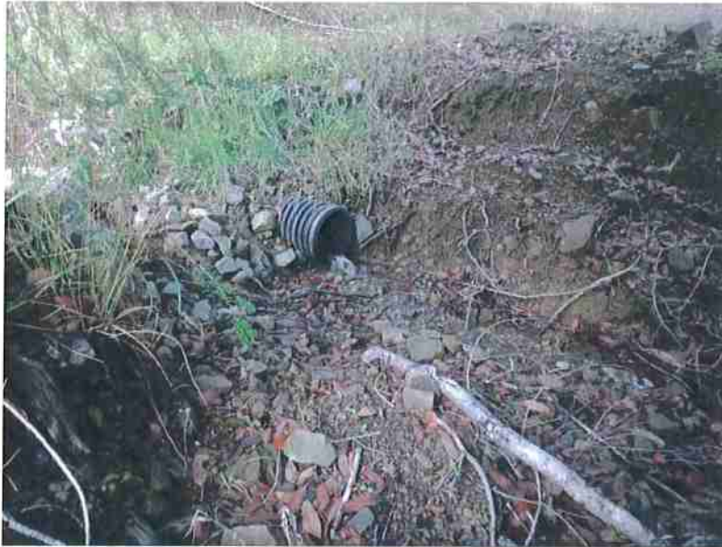
Photo 23. Stream Crossing #9, view of 12-inch diameter culvert outlet. Culvert is properly aligned with the natural grade of the stream channel, and at natural grade but is undersized for the expected 100-year streamflow event and associated debris. Culvert is plugged at inlet, obscured beneath aggraded sediments.
