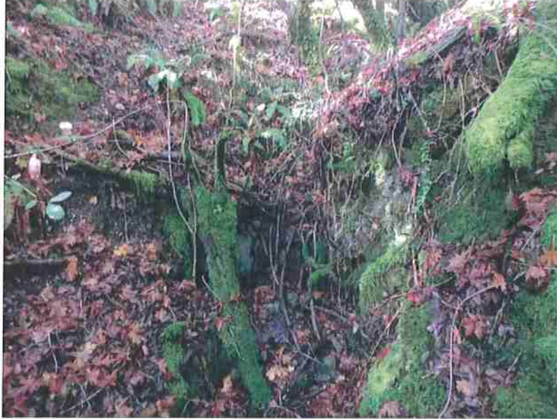
Photo 8. Stream Crossing #4, upstream view of channel of Class II watercourse leading to culvert inlet.
