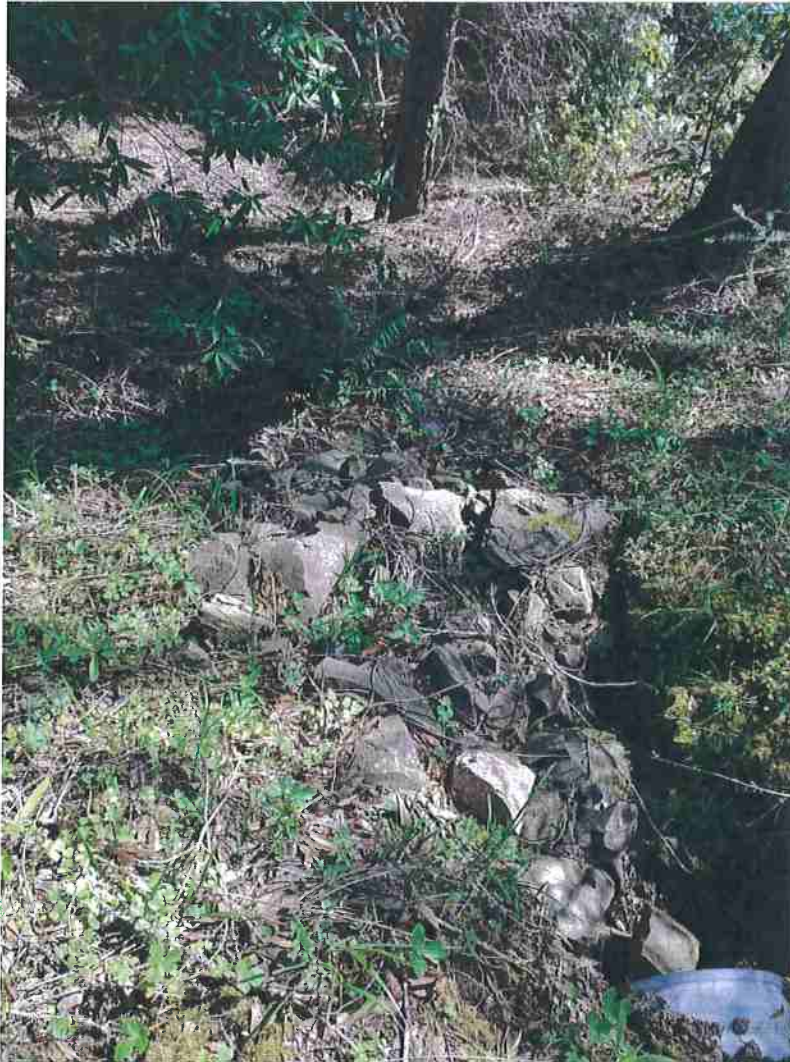
Photo 13. Stream Crossing #5, view of watercourse exiting culvert outlet. Culvert is placed at the natural grade of the stream channel, and outlets onto a well emplaced rip rap apron.
