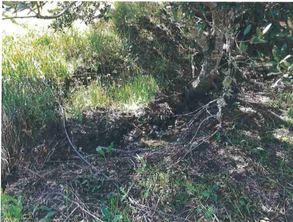
Photo 18. Stream Crossing #8, view of Class III stream channel leading to 18-inch diameter HDPE culvert inlet.
