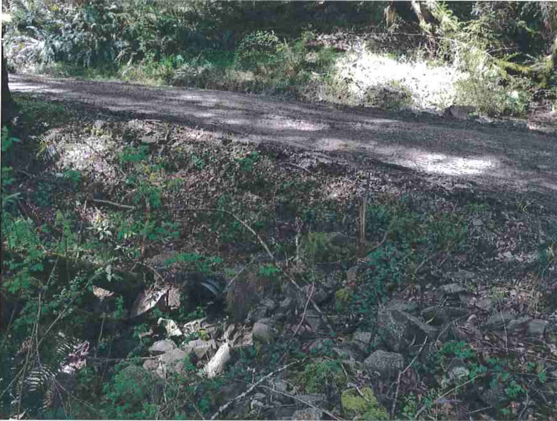
Photo 14. Stream Crossing #6, view of culvert outlet placed short in the fill. Culvert is properly aligned with the natural grade of the stream channel, and outlets water onto rock armor. OBF is armored to prevent erosion. Legacy waste was observed in the channel (tire).
