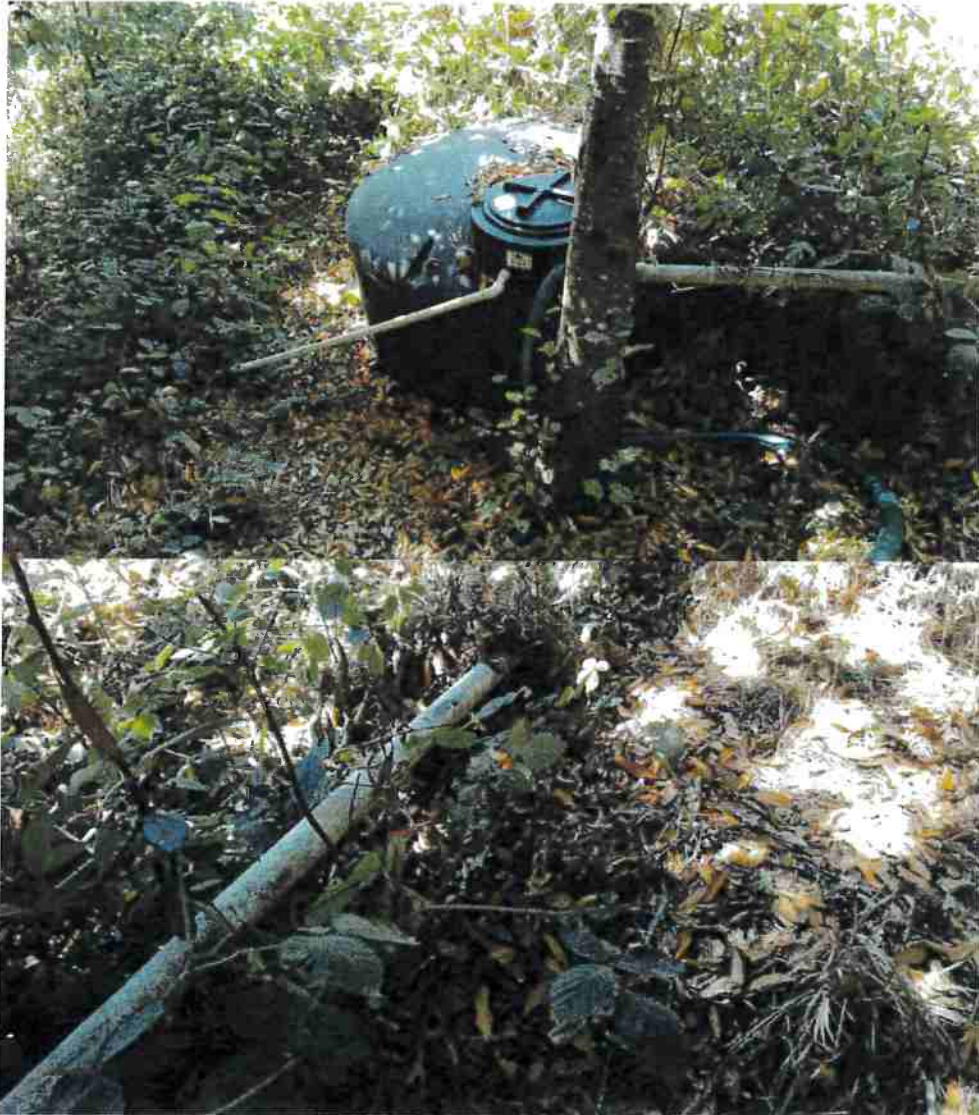
Pictures 6 & 7: These are photographs of the domestic POD #3. This diversion consists of a 3 inch PVC buried into the hillside. The diversion diverts to this 550 gallon storage tank. The rate of diversion is approximately 2 gallons per minute. Photo date: 09/13/2016
