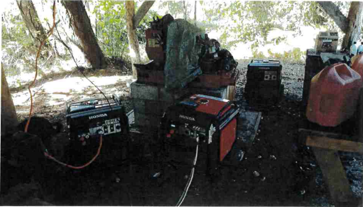
Picture 10: This is a photo of the generator area. The discharger utilizes three Honda generators to provide power to the residence and cultivation sites. Five gallon fuel canisters used for temporary fuel storage can be seen in this photo. The discharger will contain these canisters in plastic tubs to ensure containment. Photo date: 09/13/2016.
