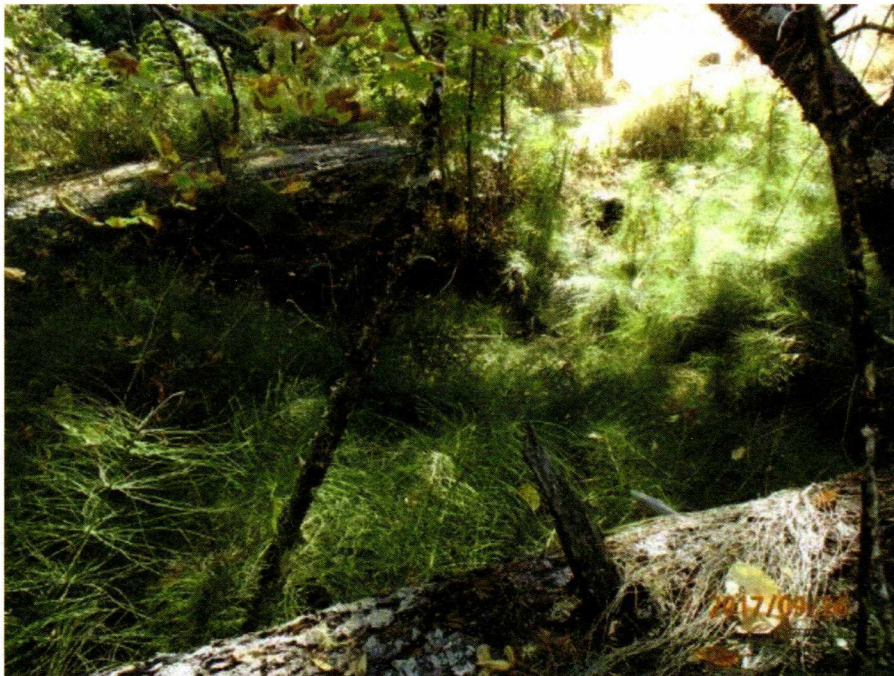
Photo 8 - SC #1. View looking upstream from below the stream crossing near the right bank at the three culvert outlets and existing road bed.
