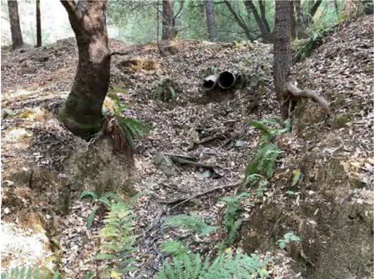
Photo 61: Stream Crossing 23. Looking upstream towards the outlet of the double barreled 18-inch and clogged 12-inch diameter culvert at stream crossing 23. Photo date 9-1-2021.
