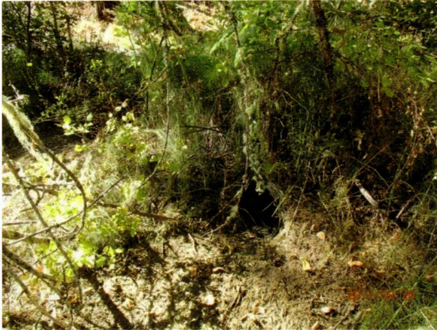
Photo 5 - SC #1. View of the second 15-inch diameter culvert inlet at the right edge of the stream crossing looking downstream.
