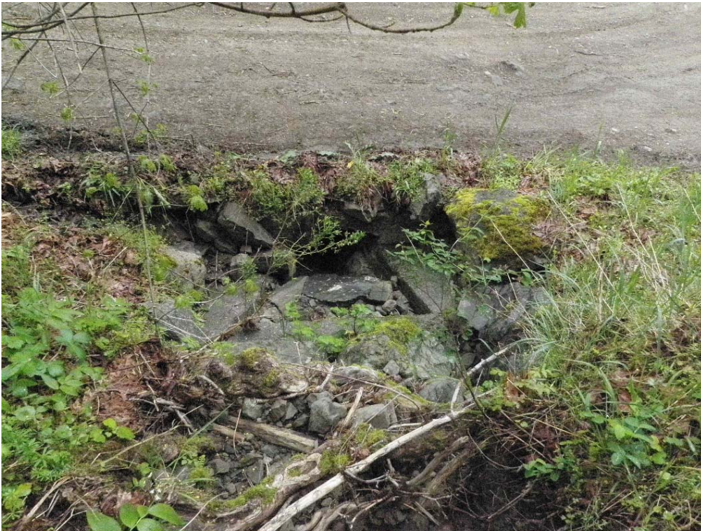
Photo 7- View of 2' long 12" diameter culvert inlet on Waterloo watercourse. Culvert inlet is difficult to observe due to poor placement of rock armor. Photo April 2011
