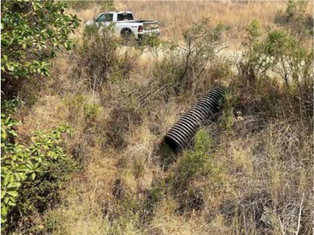
Photo 38: Stream Crossing 11. Looking towards the outlet of the 24-inch diameter culvert at stream crossing 11. Photo date 9-1-2021.
