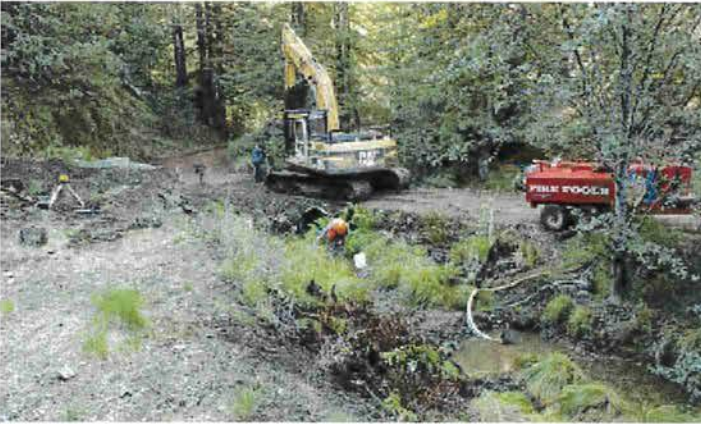
FIGURE 199. For larger streams, pump trucks, large pumps or multiple small pumps can be used to pump streamflow around project work sites. Here, a pump truck is used to temporarily divert flow in a fish bearing stream where dual culverts are being replaced with a riser bridge. Young fish were removed from this fish bearing stream before project work started.
