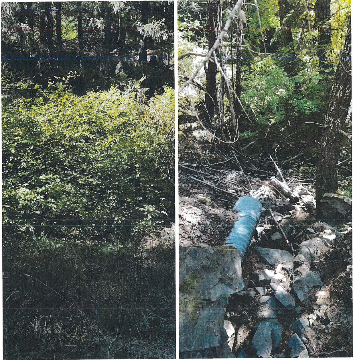
Picture 10 & 11: Looking upstream from the inlet (left) to Crossing #3 and downstream from the outlet (right). Photos date 10-11-19.
