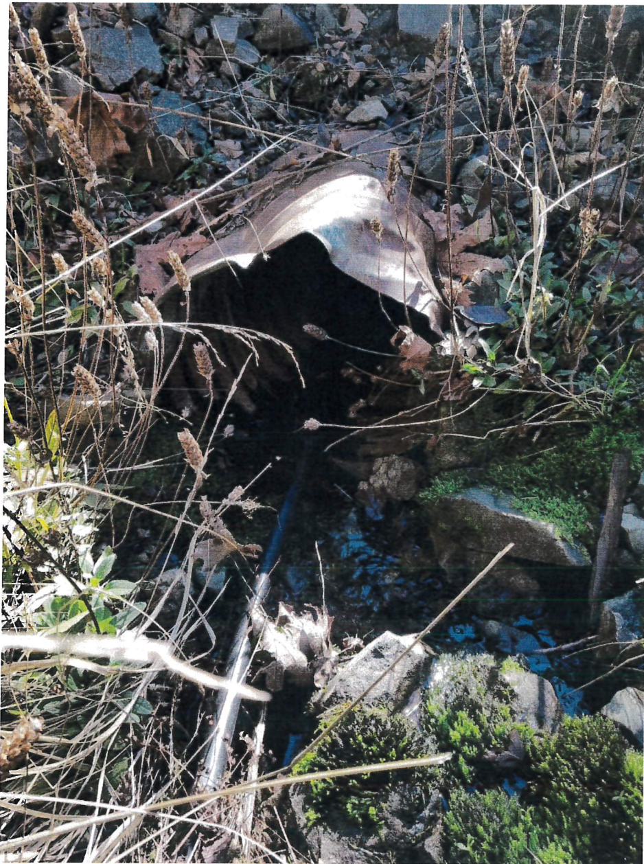
Picture 4: Looking downstream at the inlet to Crossing #1 on a watercourse. Photo date 10-11-19.
