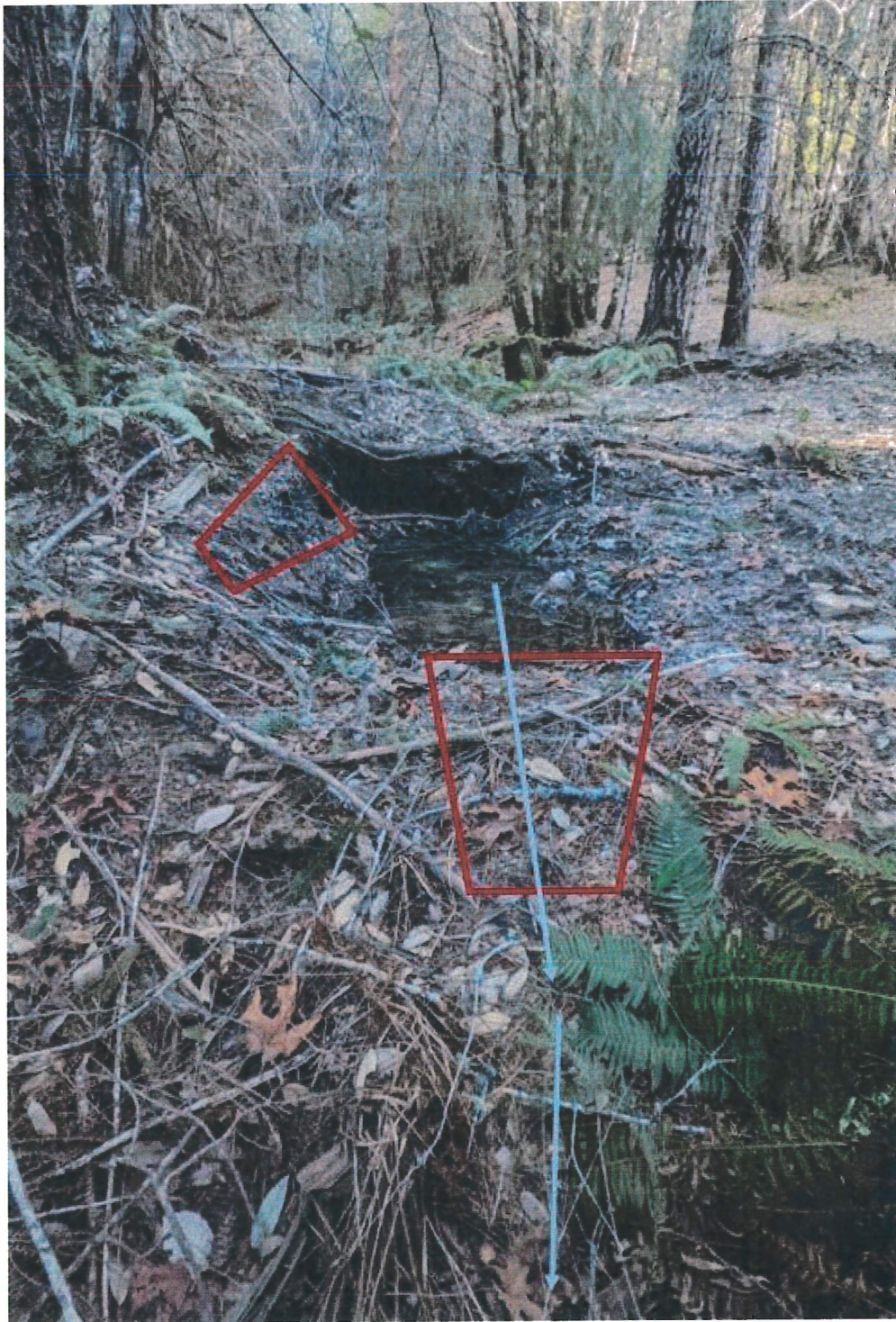
Picture 33: Pool located at the top of the channel where water is daylighting before heading to Crossing 10. The top red area indicates the overly steep slope which shall be pulled back and stabilized. The lower red area indicates the small berm which is causing the pooling and shall be removed to promote flow. The blue arrows indicate flow direction. Photo date 2/2/22.
