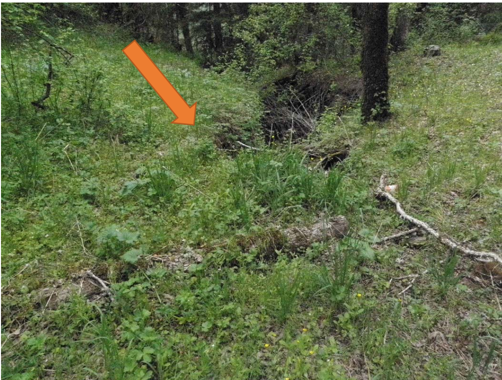
Photo 6 – View of lead pipe protruding below the stream. Photo April 2014
