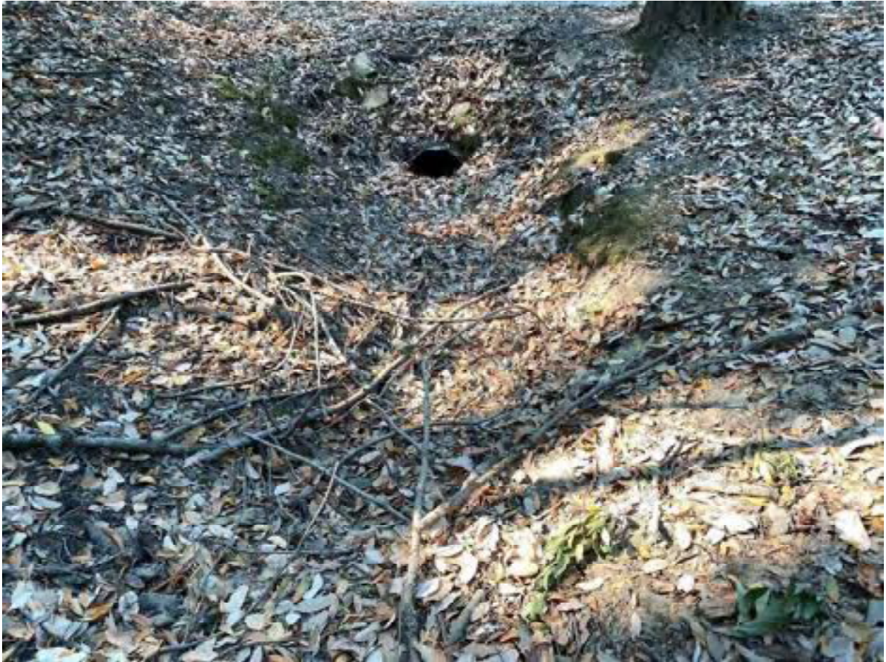
Photo 58: Stream Crossing 23. Looking downstream towards the inlet of the double barreled 18-inch and clogged 12-inch diameter culvert at stream crossing 23. Photo date 9-1-2021.
