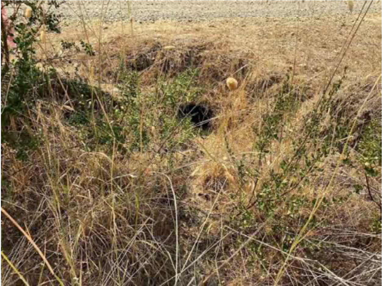
Photo 16: Stream Crossing 05. Looking downstream towards the inlet of the 12-inch diameter culvert at stream crossing 05. Photo date 9-1-2021.
