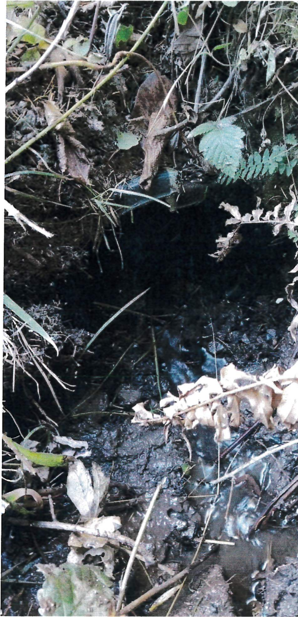
Picture 6: Looking downstream at the inlet to Crossing #2 on a watercourse. Photo date 10-11-19.
