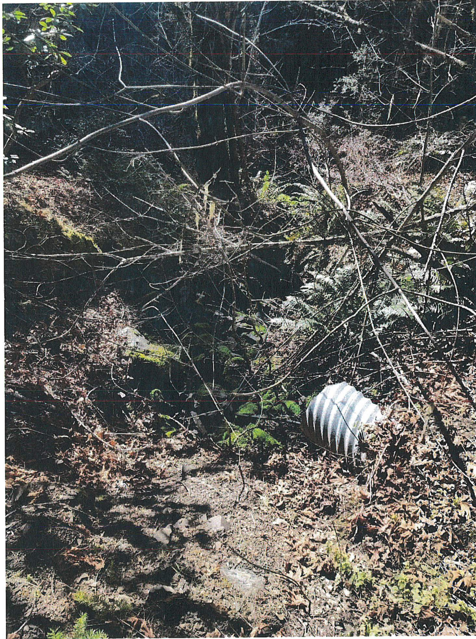
Picture 5: Looking downstream at the outlet from Crossing #1 on a watercourse. Photo date 1-21-21.
