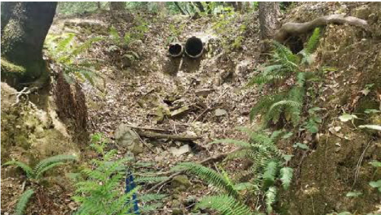
Outlet of watercourse crossing at Site 23. Blue flag represents proposed outlet of culvert upgrade.
