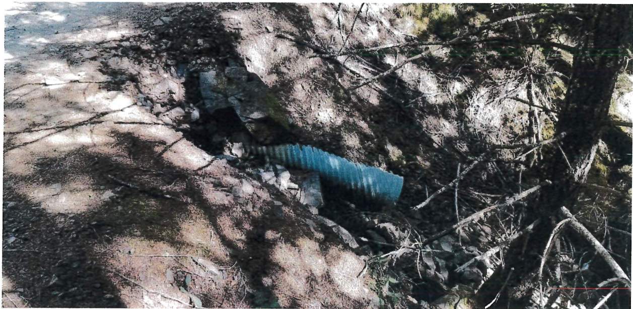
Picture 12 & 13: Looking downstream at the inlet (top) and the outlet (bottom) to Crossing #3. Photos date 10-11-19.
