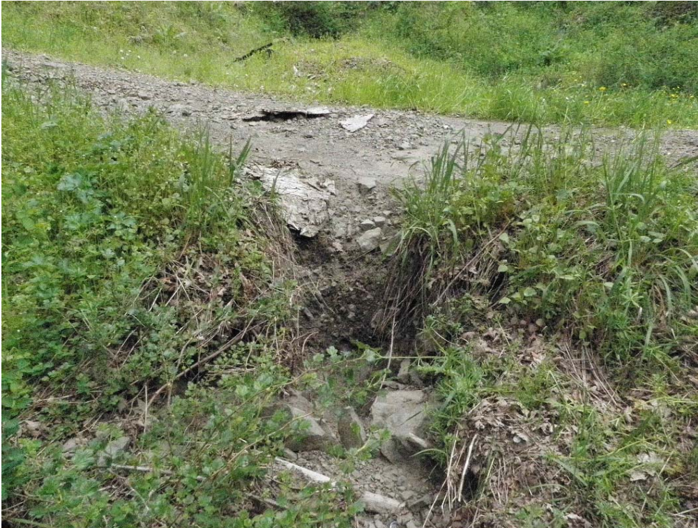
Photo 5 – View of lead pipe protruding in stream at a lead pit forming in the embankment on the left side of the road on the Sierra Leone Photo April 2014
