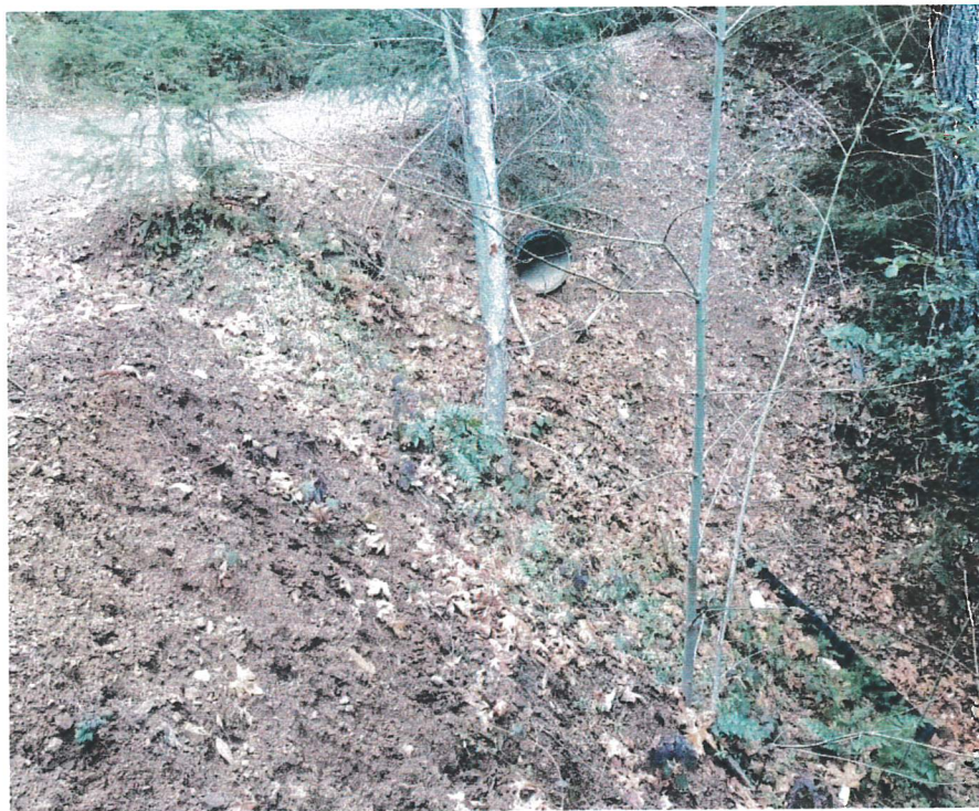
Picture 30 & 31: Looking downstream at the inlet (top) and upstream at the outlet (bottom) to Crossing #7 on a watercourse. Photos date 1-21-21.
