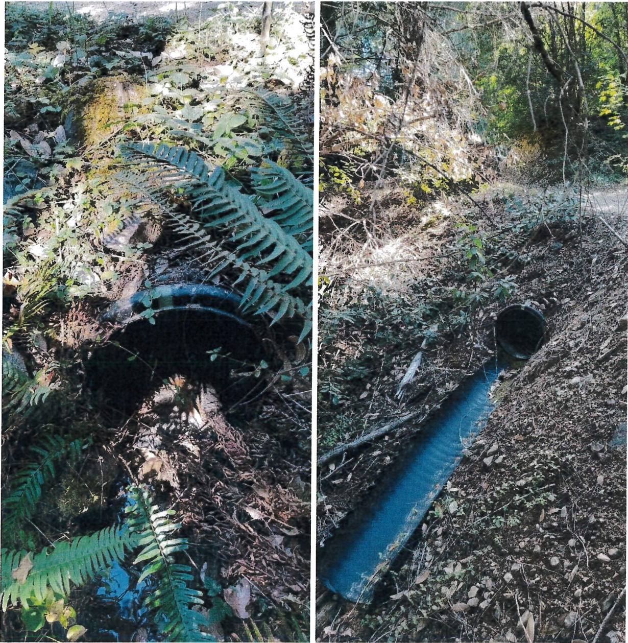
Picture 25 & 26: Looking downstream at the inlet (left) and upstream at the outlet (right) to Crossing #6 on a watercourse. Photos date 10-11-19.
