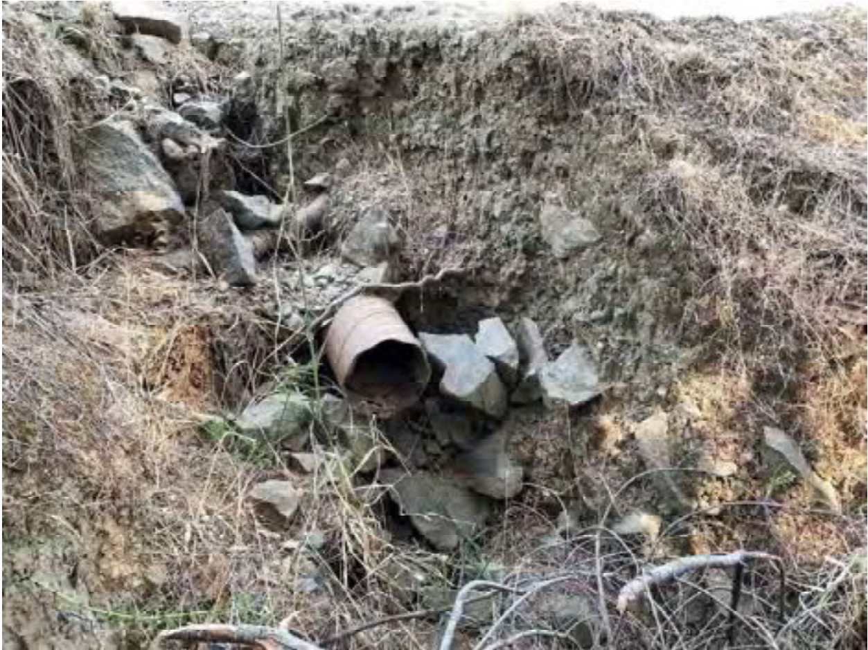
Photo 33: Stream Crossing 08. Looking upstream towards the outlet of the 8-inch diameter culvert at stream crossing 08. Photo date 9-1-2021.
