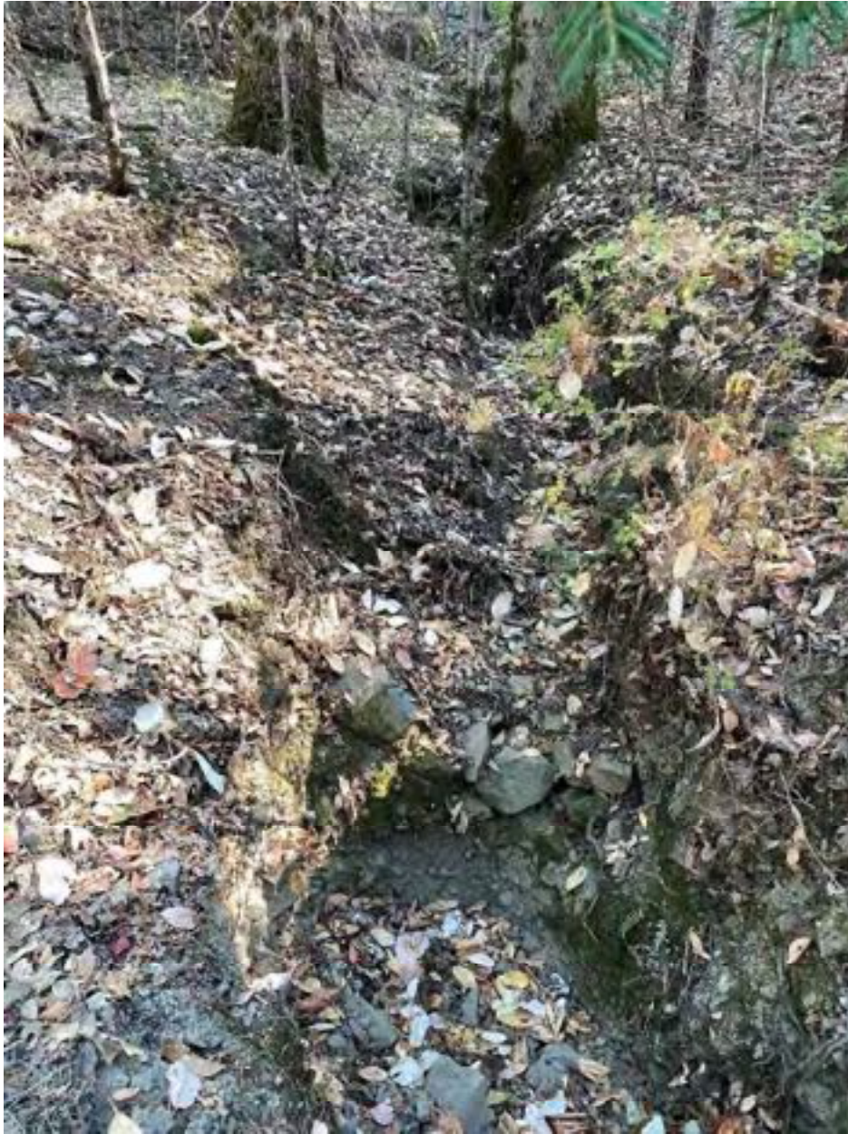
Photo 48: Stream Crossing 17. Looking upstream from the inlet of the 18-inch diameter culvert at stream crossing 17 that is proposed for removal. Photo date 9-1-2021.
