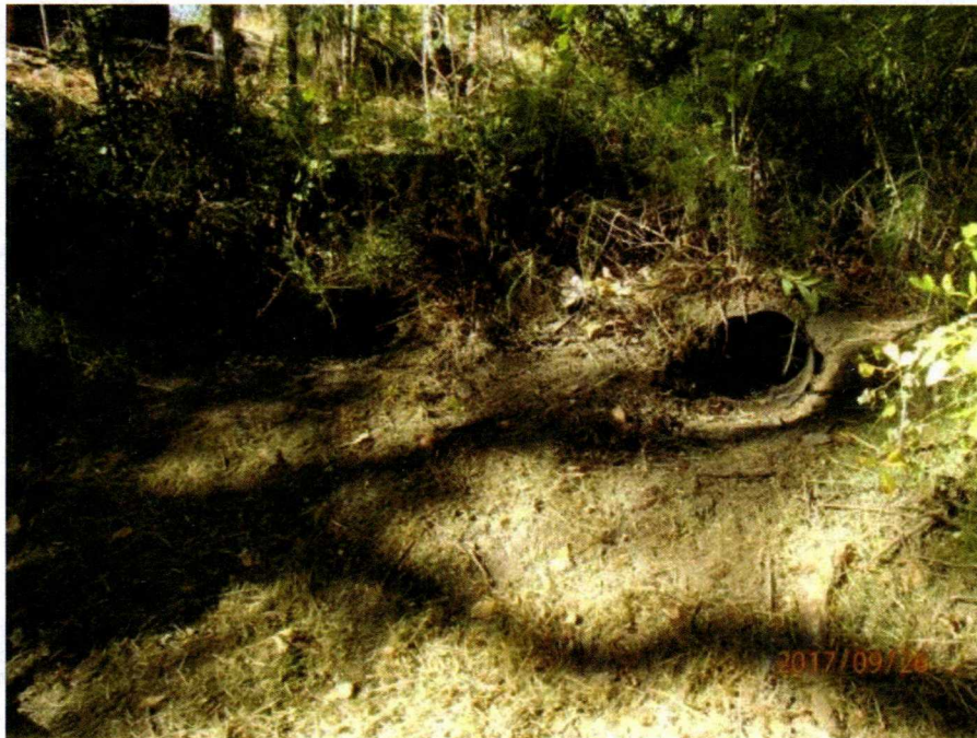
Photo 4 - SC #1. View of the 12-inch diameter culvert inlet near the left edge of the frame and the middle 15-inch diameter culvert inlet looking downstream.
