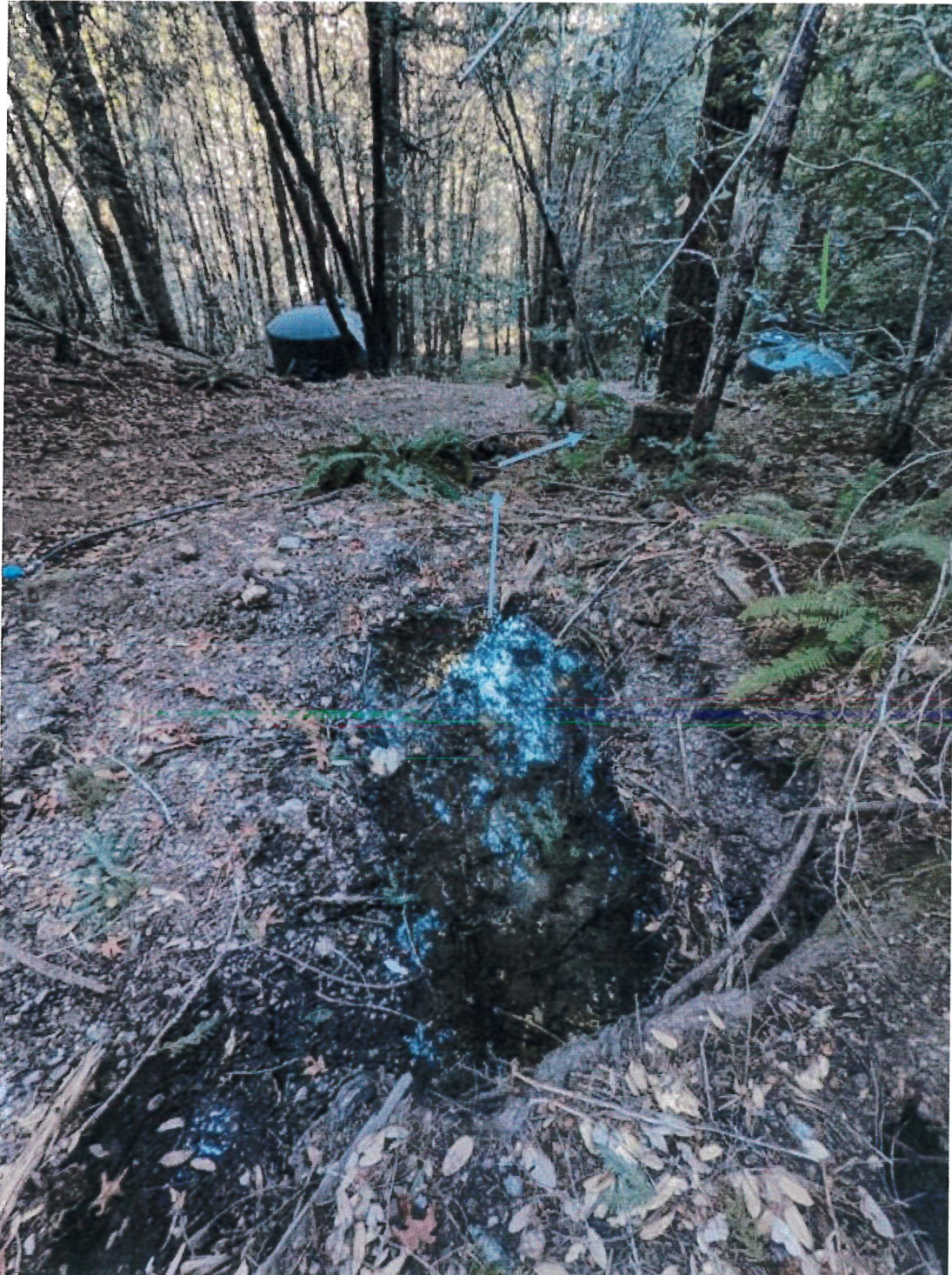
Picture 34: Looking downslope from the pooled area towards the inside ditch and Crossing 10. Blue arrows indicate flow direction. The green arrow indicates the location of the water tank that may need to be relocated. Photo date: 2/2/22.
