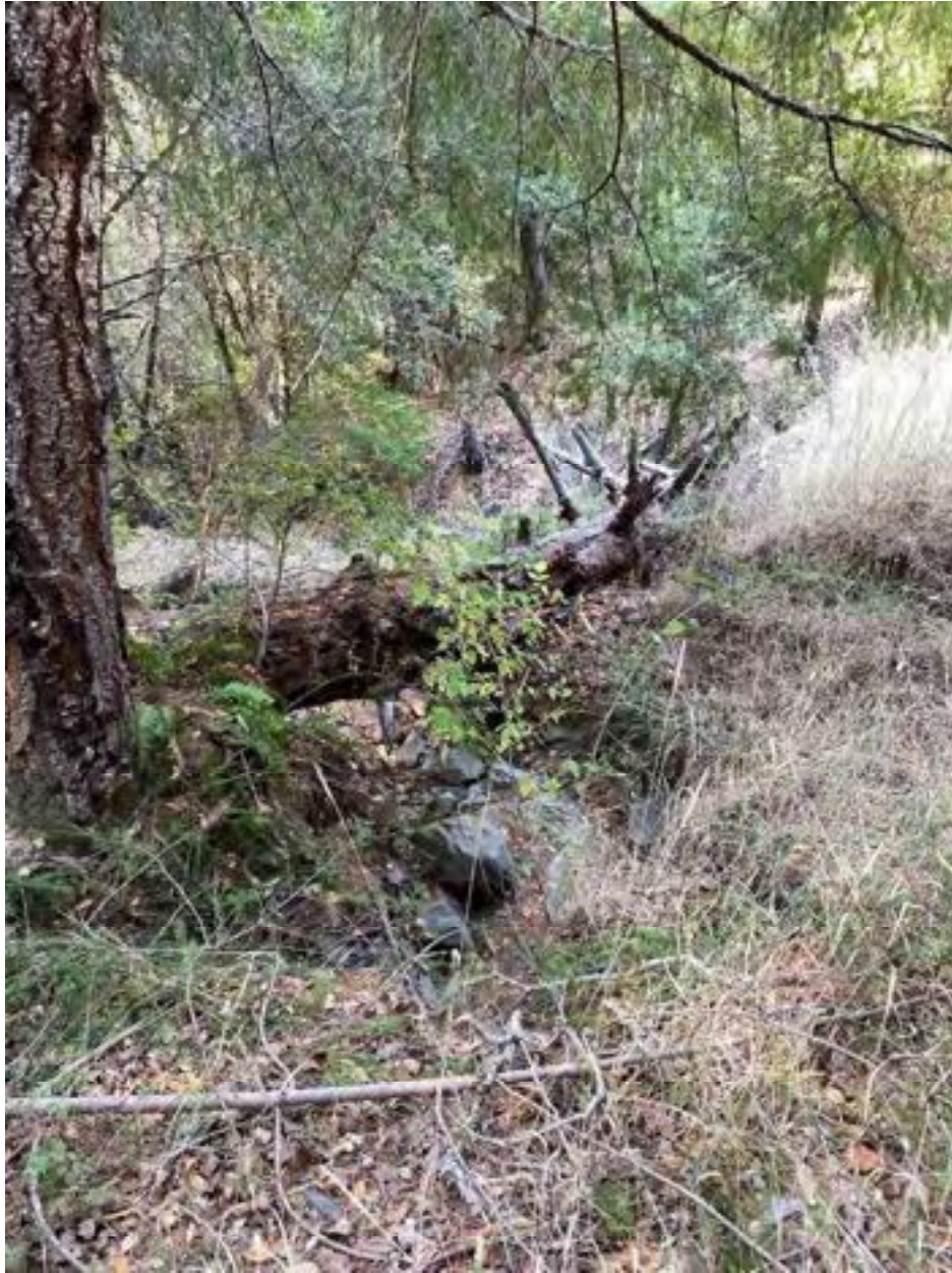
Photo 56: Stream Crossing 19. Looking downstream from the outlet of the 18-inch diameter culvert at stream crossing 19. Photo date 9-1-2021.
