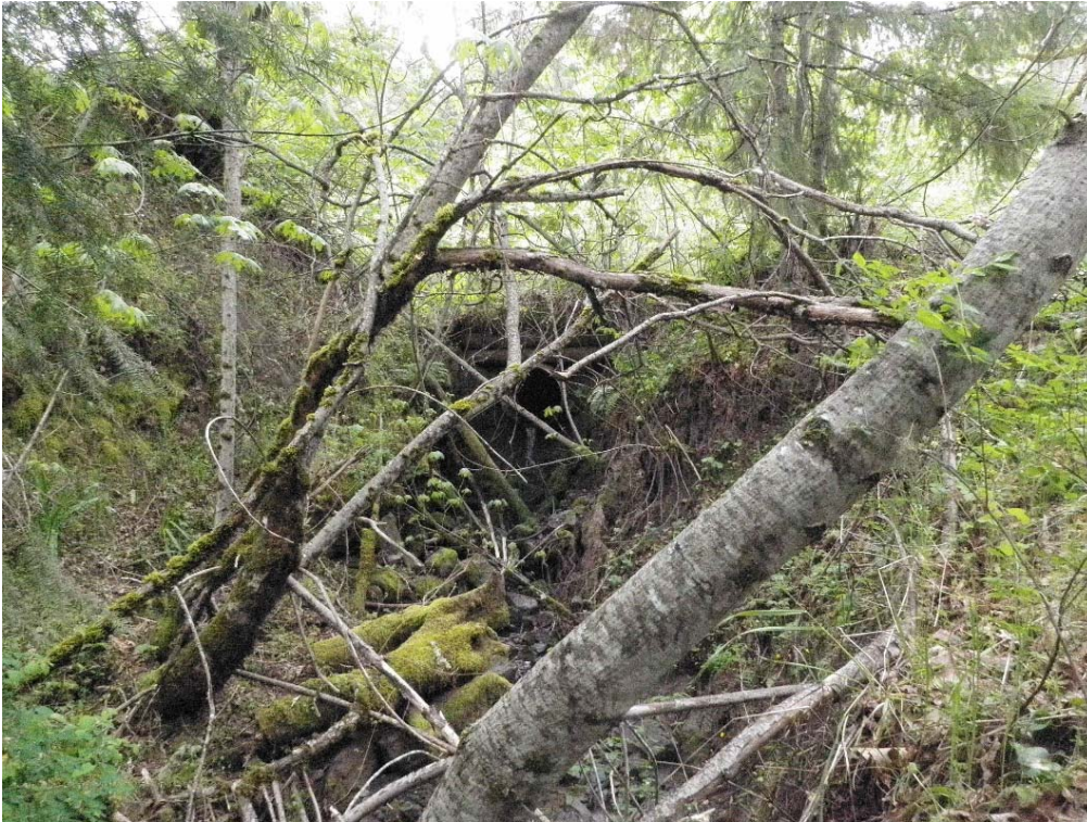
Photo 9 – View of stream at 1-inch diameter culvert outlet on lateral watercourse. Culvert is installed in fill pit at root plane at the culvert outlet. It does not allow for the passage of aquatic organisms. Photo April 2000
