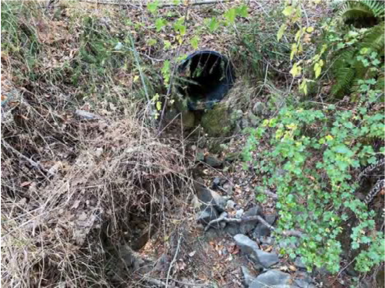
Photo 55: Stream Crossing 19. Looking upstream towards the outlet of the 18-inch diameter culvert at stream crossing 19. Photo date 9-1-2021.
