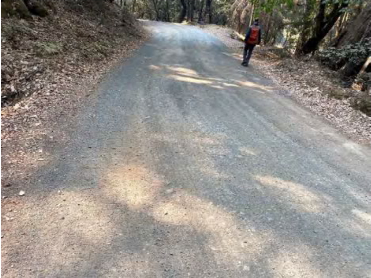
Photo 65: Stream Crossing 24. The roadside approach to stream crossing 24 facing South. Photo date 9-1-2021.
