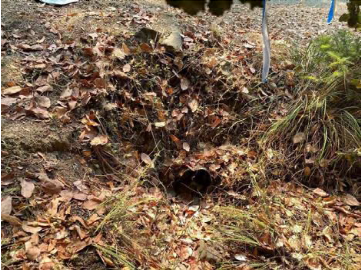
Photo 25: Stream Crossing 07. Looking downstream towards the inlet of the 12-inch diameter culvert at stream crossing 07. Photo date 9-1-2021.
