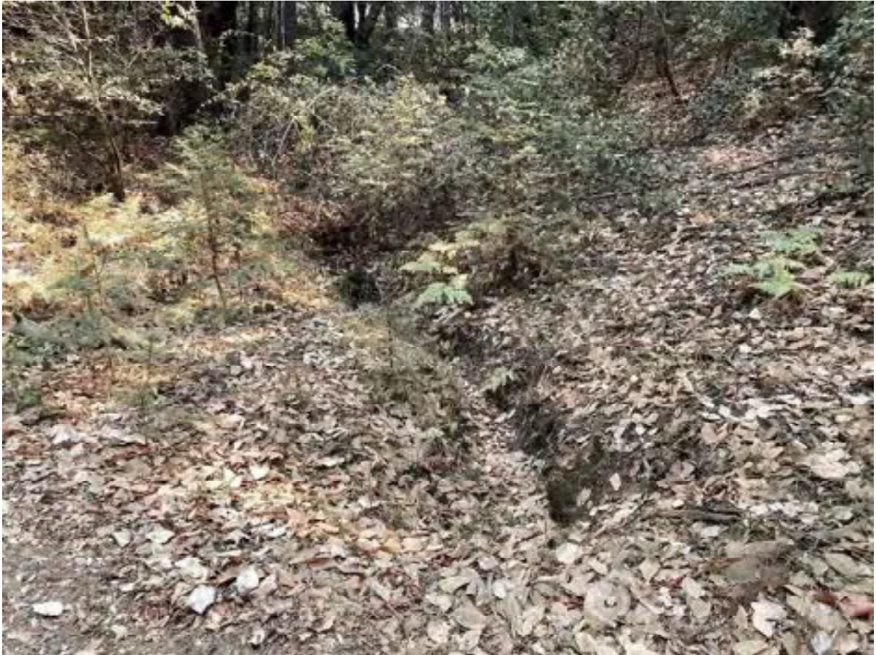
Photo 64: Stream Crossing 24. Looking upstream from the inlet of the 18-inch diameter culvert at stream crossing 24. Photo date 9-1-2021.
