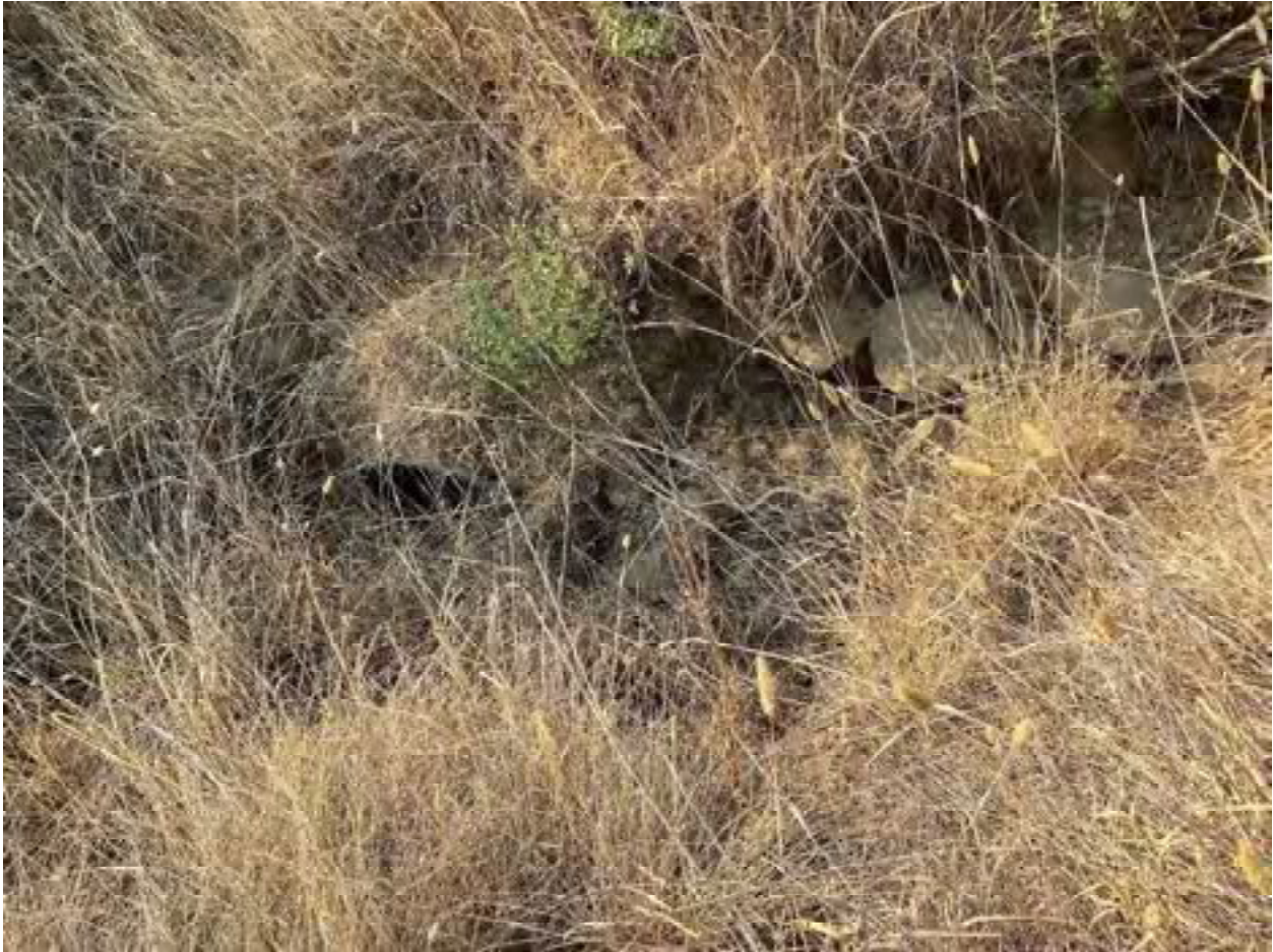
Photo 35: Stream Crossing 11. Looking downstream towards the inlet of the 24-inch diameter culvert at stream crossing 11. Photo date 9-1-2021.
