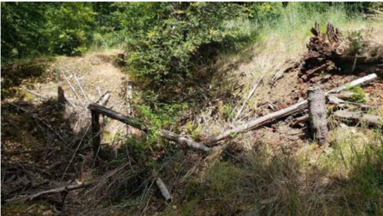
Site 19. Photo of the southeastern embankment of G5/G6/G, immediately down stream of the outlet of the watercourse crossing at Site 19. Note vegetation and rotted tree in the upper right. Indicative that this location has been in this condition for many years and was not recently created.
