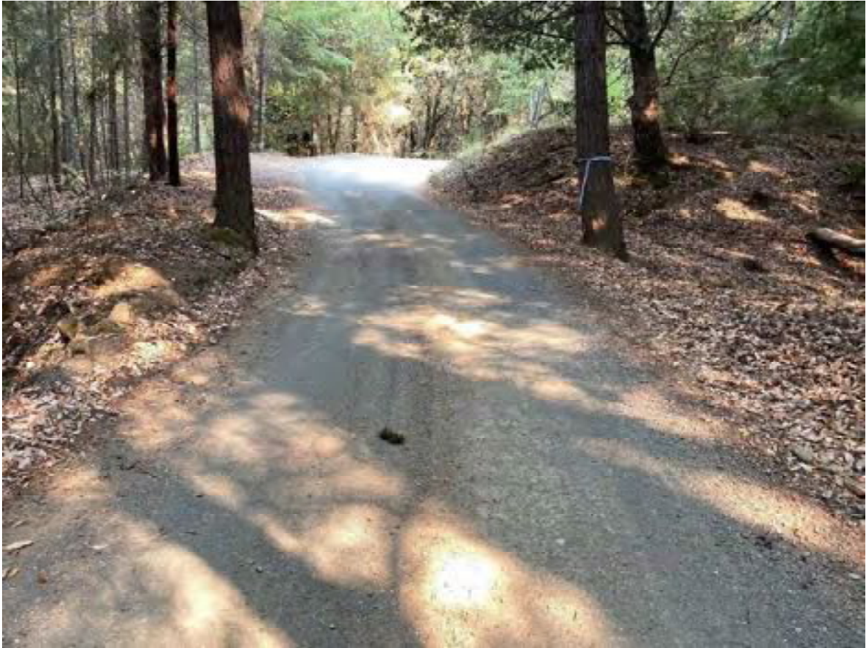
Photo 60: Stream Crossing 23. The roadside approach to stream crossing 23 facing North. Photo date 9-1-2021.
