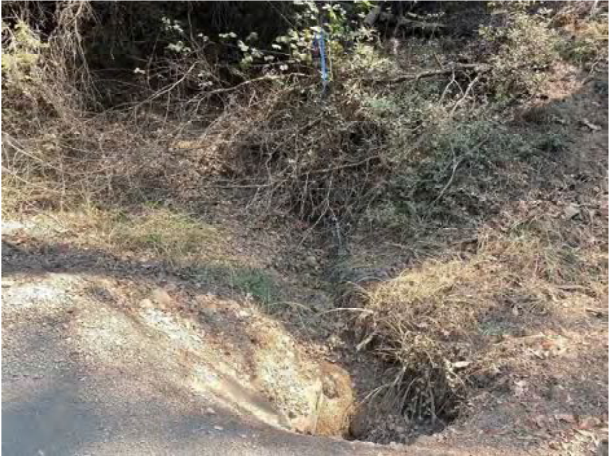
Photo 69: Stream Crossing 26. Looking upstream from the inlet of the 18-inch diameter culvert at stream crossing 26. Photo date 9-1-2021.
