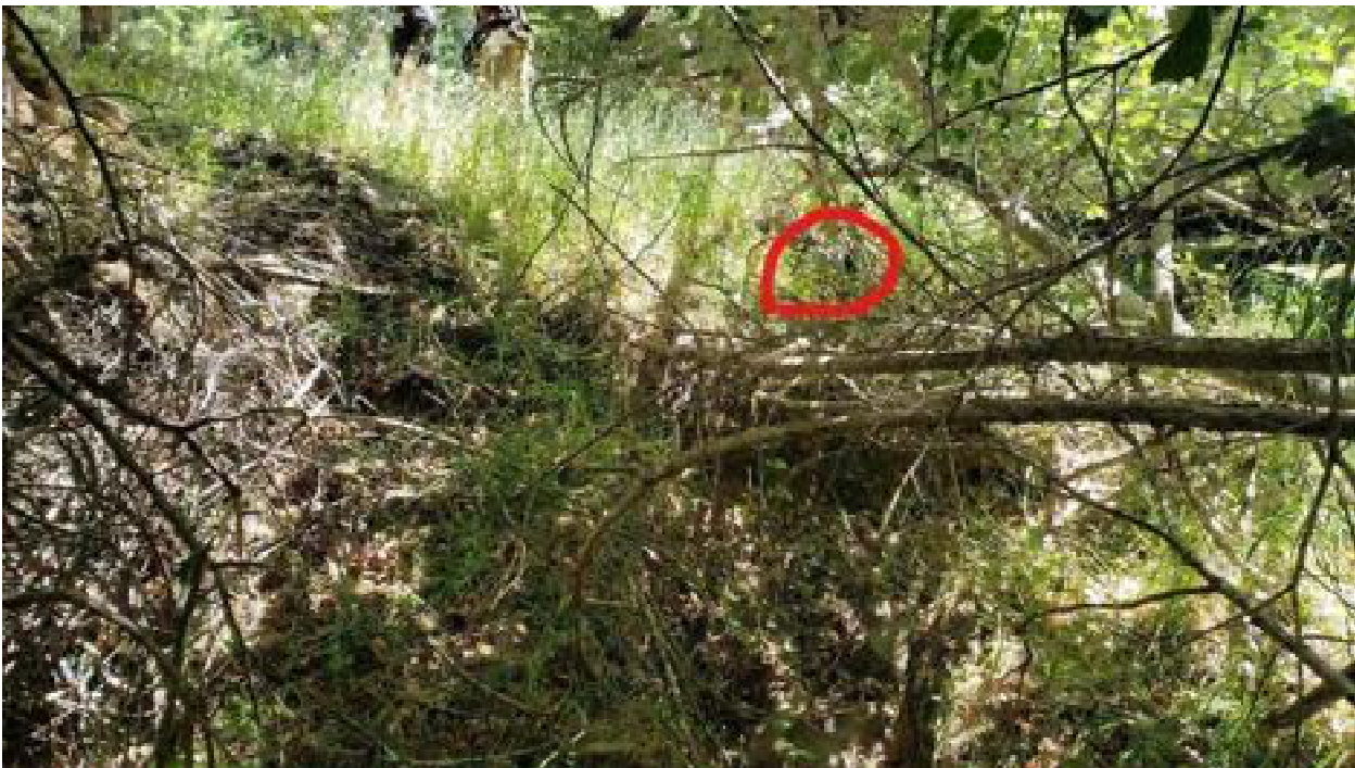
Site 35. Looking at the outlet(circled). The culvert upgrade will re-align the watercourse to its original channel, which will require the outlet to be placed in the lower left of the photo.
