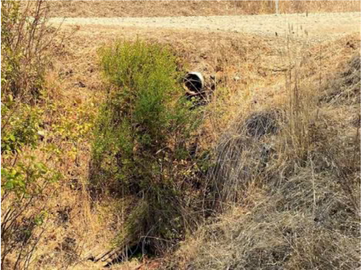
Photo 9: Stream Crossing 03. Looking upstream towards the outlet of the 8-inch diameter culvert at stream crossing 03. Photo date 9-1-2021.
