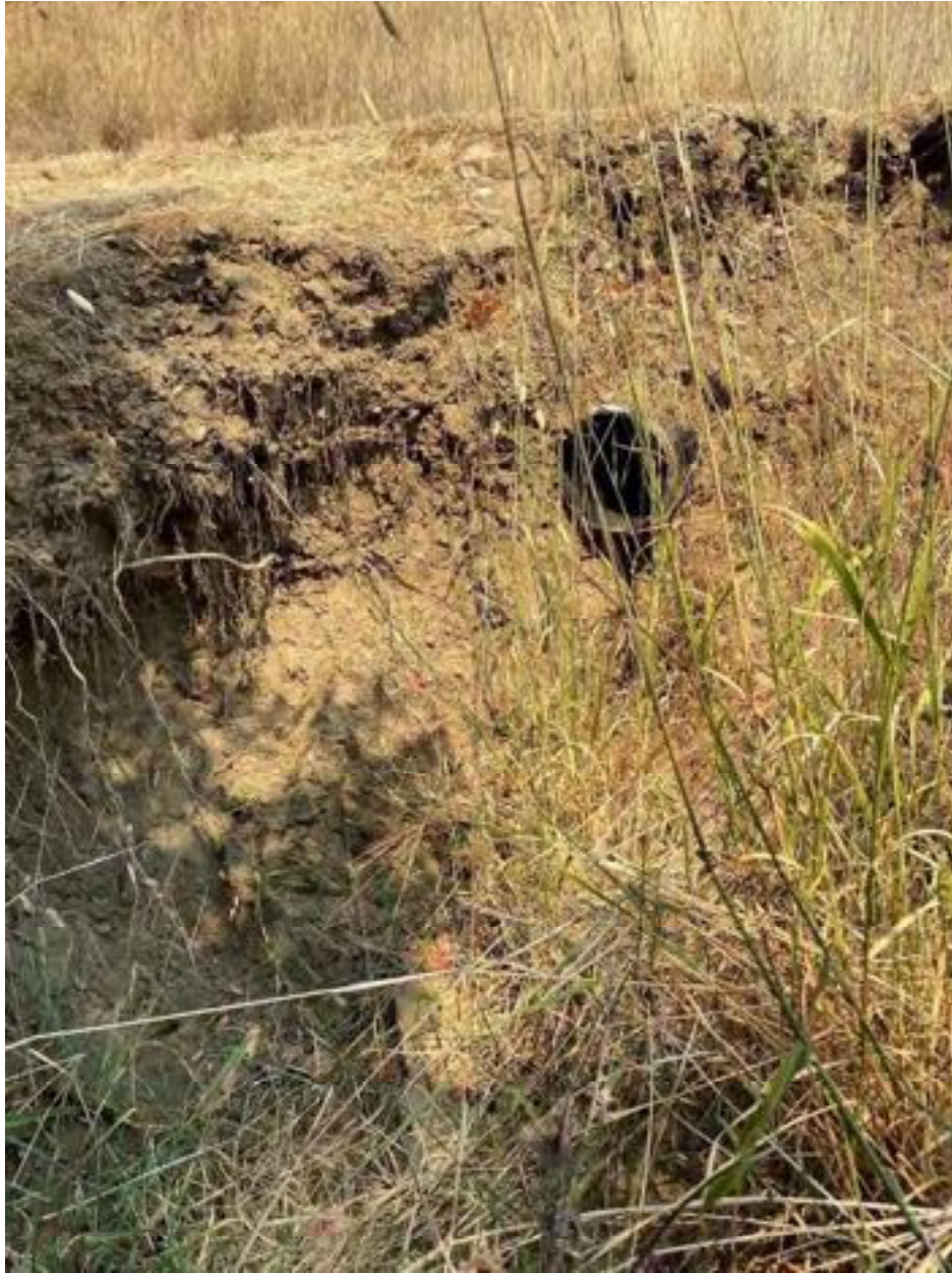
Photo 19: Stream Crossing 05. Looking upstream towards the outlet of the 12-inch diameter culvert at stream crossing 05. Photo date 9-1-2021.
