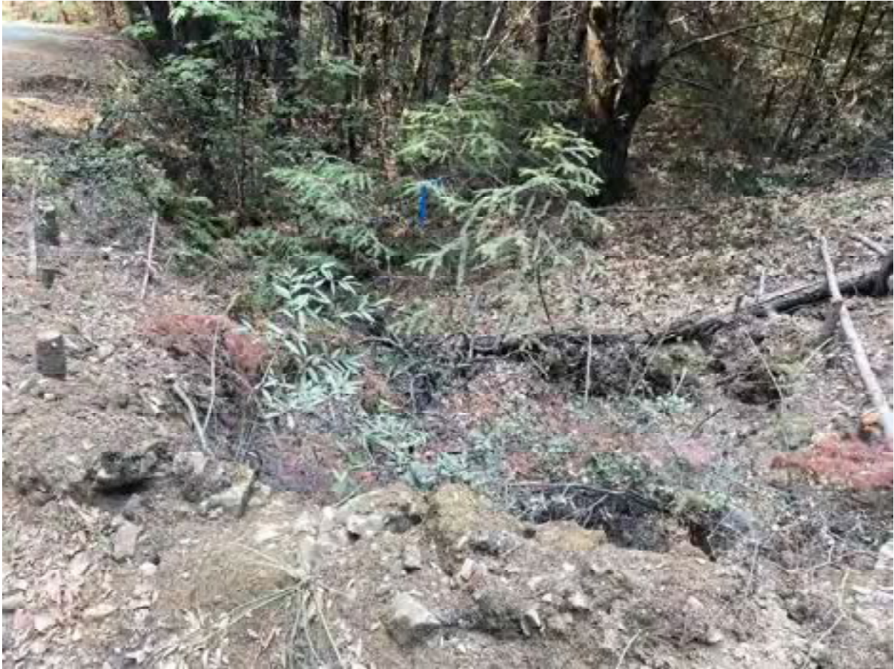
Photo 72: Stream Crossing 26. Looking downstream from the outlet of the 18-inch diameter culvert at stream crossing 26. Photo date 9-1-2021.
