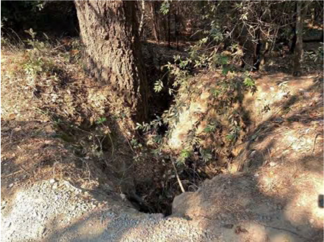
Photo 46: Stream Crossing 13. Looking downstream stream from the outlet of the 12-inch diameter DRC that is the current outlet of the water from stream crossing 13. Photo date 9-1-2021.
