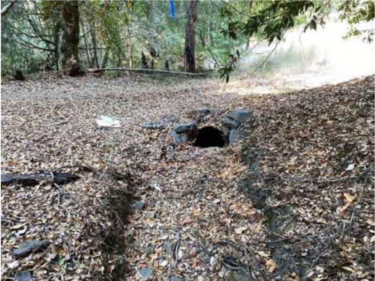
Photo 52: Stream Crossing 19. Looking downstream towards the inlet of the 18-inch diameter culvert that is proposed for removal at stream crossing 19. Photo date 9-1-2021.
