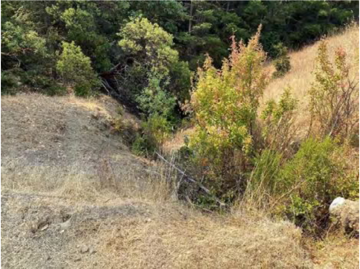
Photo 10: Stream Crossing 03. Looking downstream from the outlet of the 8-inch diameter culvert at stream crossing 03. Photo date 9-1-2021.
