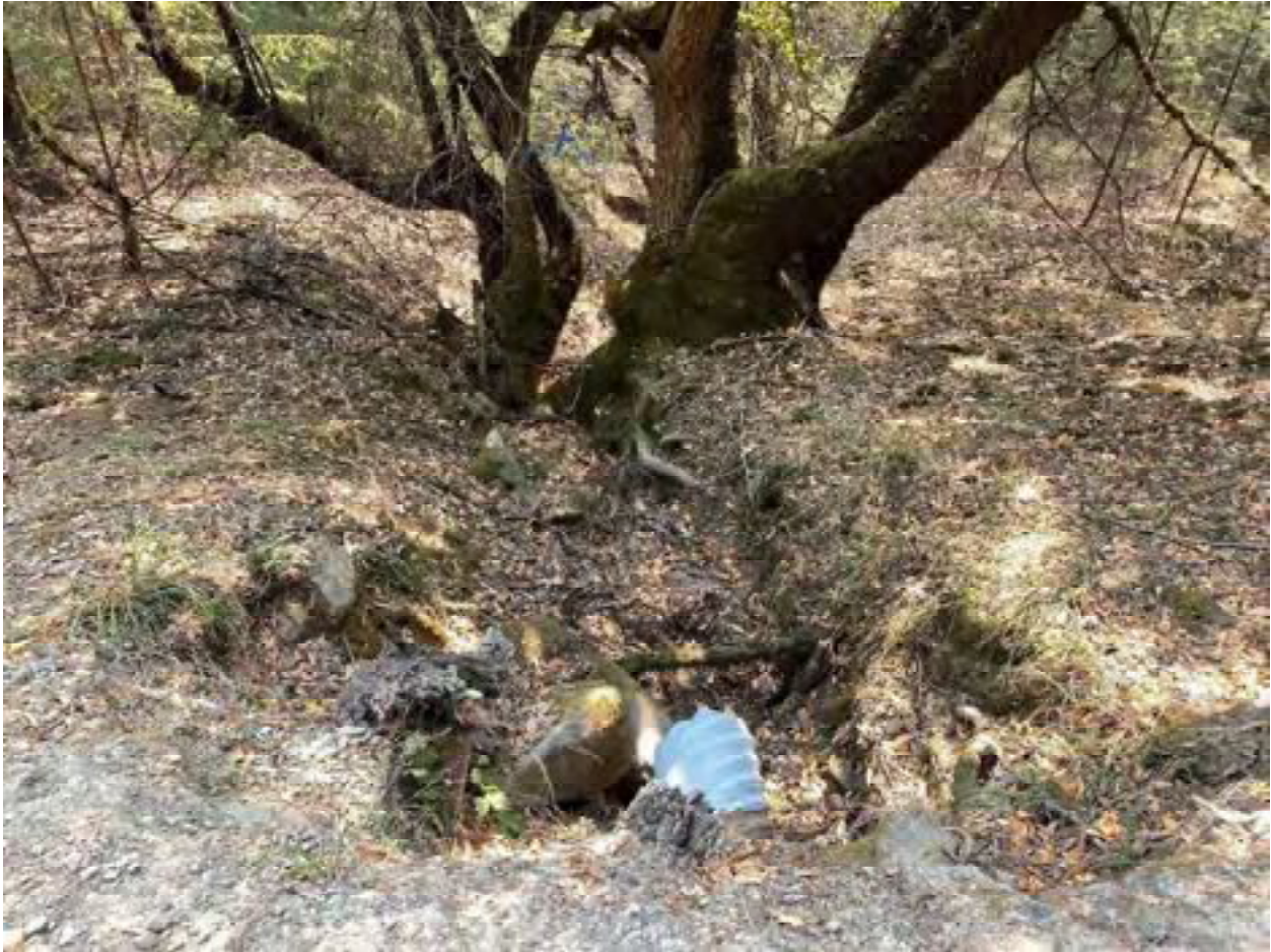
Photo 24: Stream Crossing 06. Looking downstream from the outlet of the 12-inch diameter culvert at stream crossing 06. Photo date 9-1-2021.
