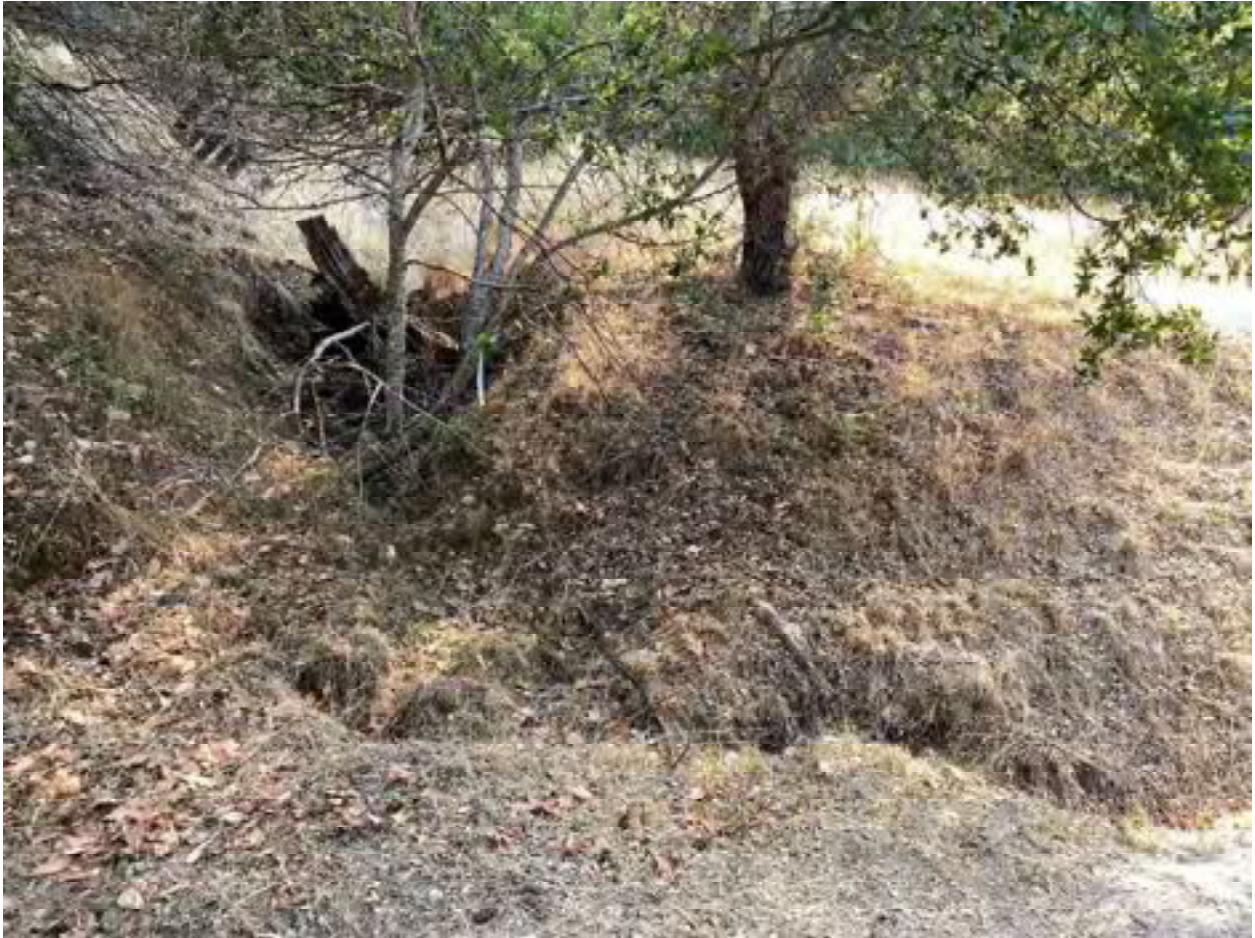
Photo 74: Stream Crossing 35. Looking upstream from the inlet of the 8-inch diameter culvert at stream crossing 35. Photo date 9-1-2021.
