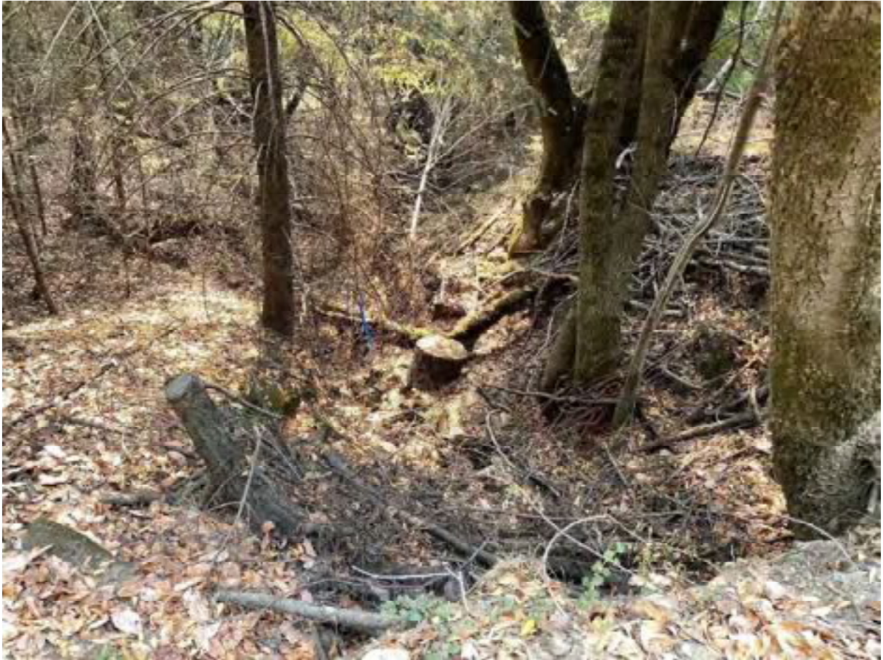
Photo 29: Stream Crossing 07. Looking downstream from the outlet of the 12-inch diameter culvert at stream crossing 07. Photo date 9-1-2021.
