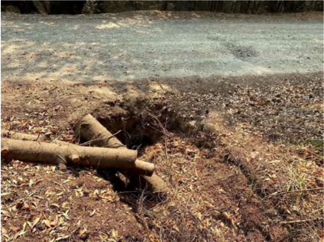
Photo 21: Stream Crossing 06. Looking downstream towards the inlet of the 12-inch diameter culvert at stream crossing 06. Photo date 9-1-2021.
