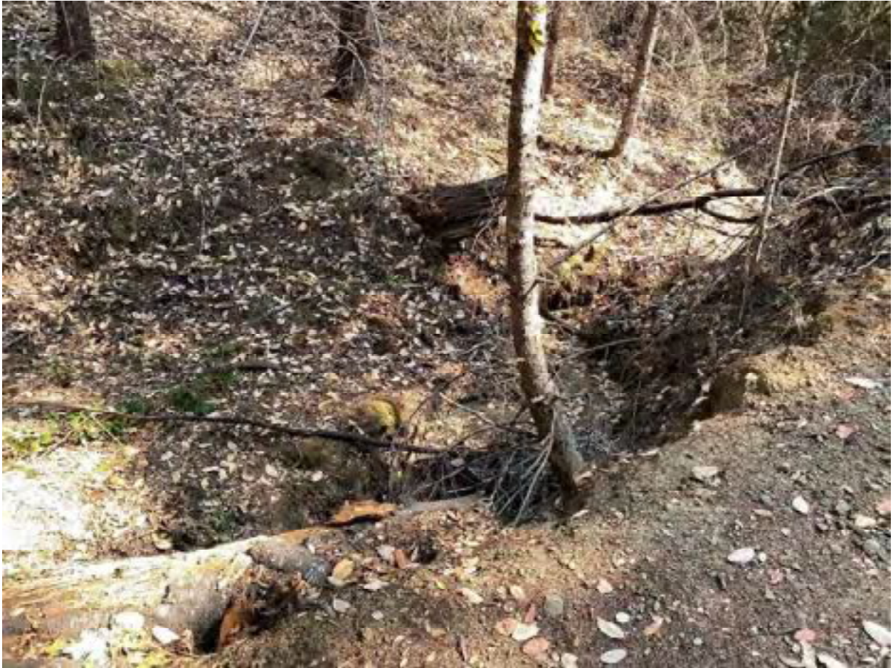
Photo 53: Stream Crossing 19. Looking upstream from the road along the native stream channel that is to be realigned at stream crossing 19. Photo date 9-1-2021.
