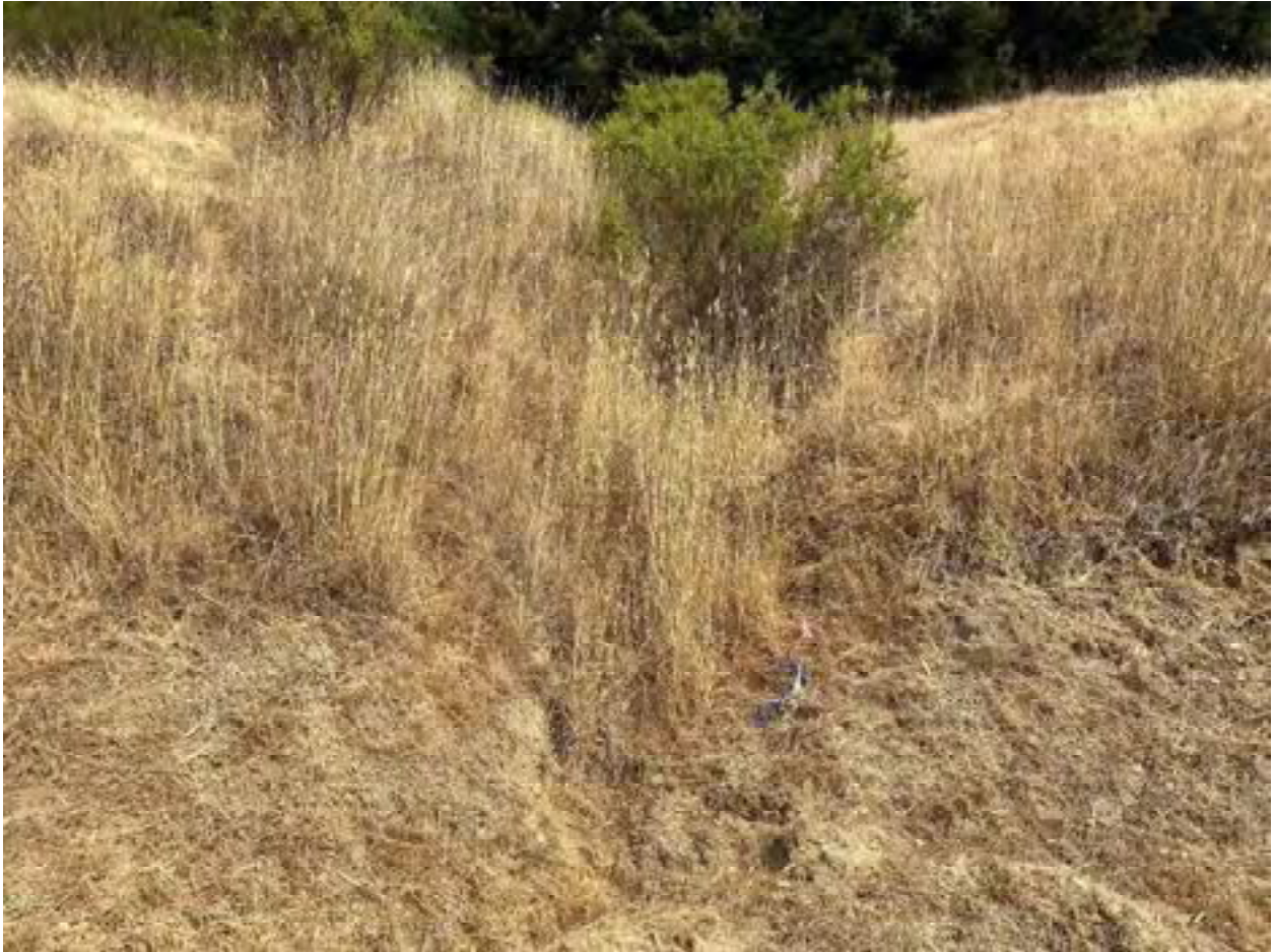
Photo 12: Stream Crossing 04. Looking upstream from the inlet of the 8-inch diameter culvert at stream crossing 04. Photo date 9-1-2021.
