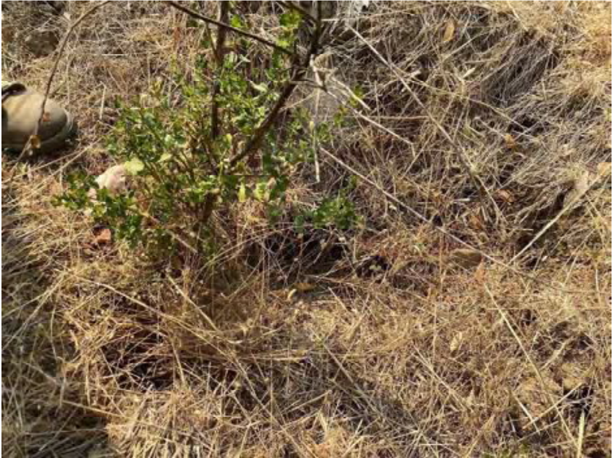
Photo 30: Stream Crossing 08. Looking downstream towards the inlet of the 8-inch diameter culvert at stream crossing 08. Photo date 9-1-2021.
