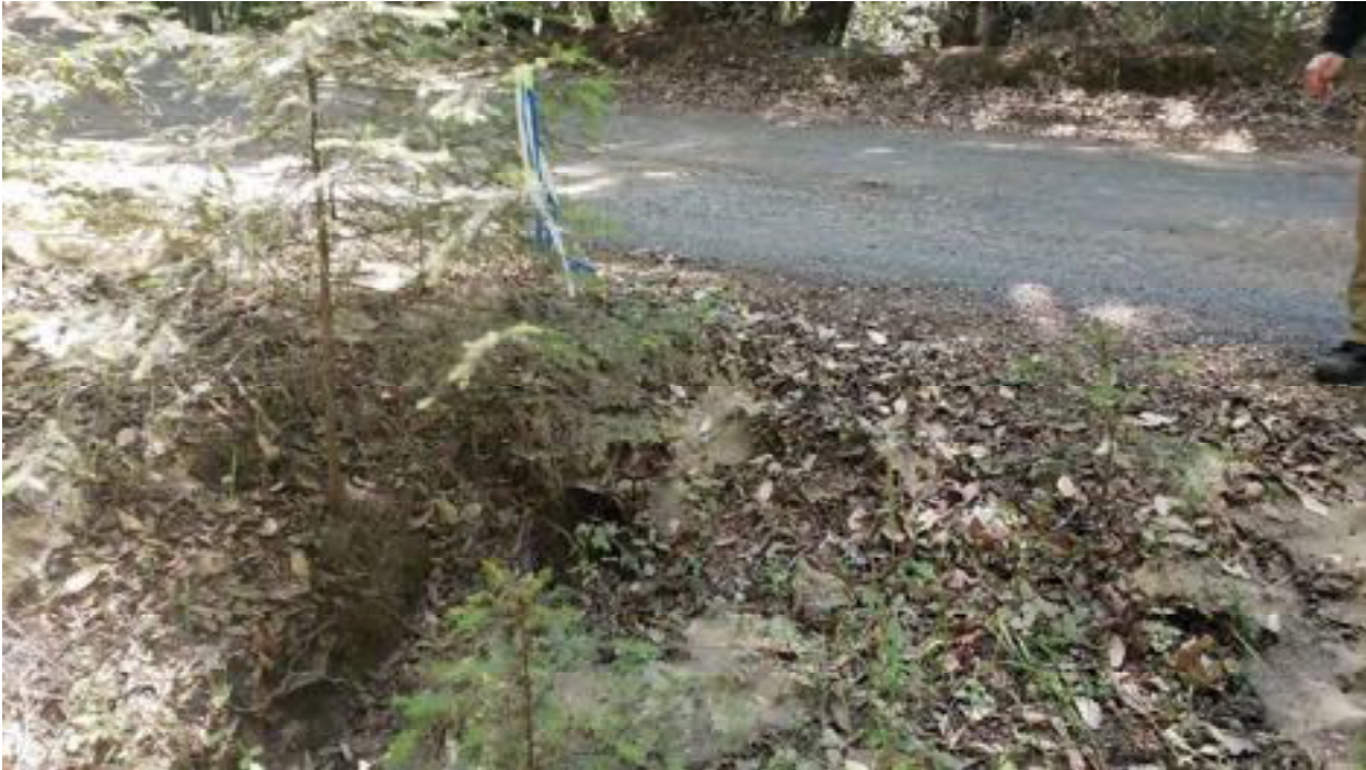
Site 24. Inlet of the watercourse crossing.
