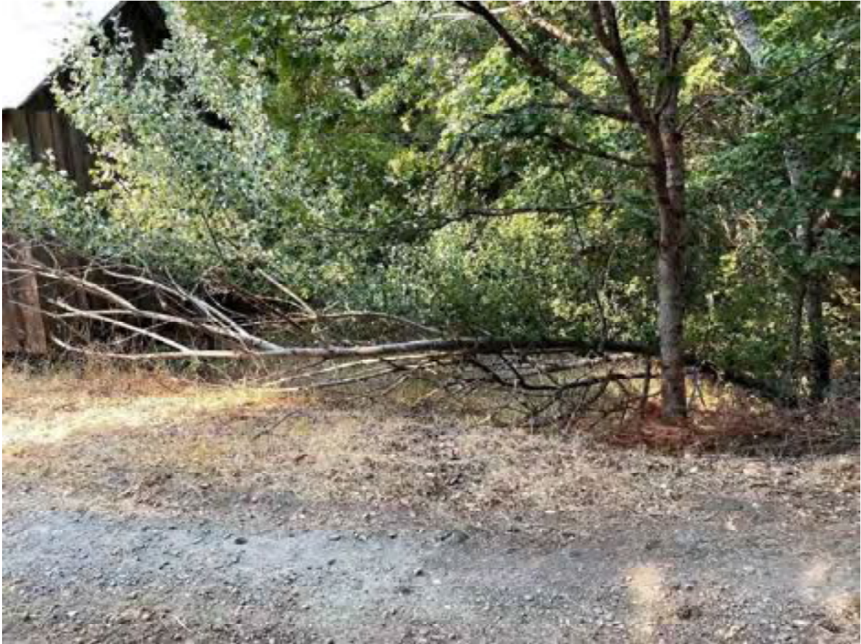
Photo 77: Stream Crossing 35. Looking downstream from the outlet of the 8-inch diameter culvert at stream crossing 35. Photo date 9-1-2021.
