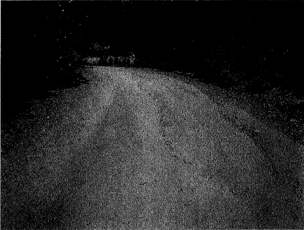
Road Point 1: Evidence of minor surface erosion. Recommended mitigation measure includes implementation of water bar or rolling dip to prevent further erosion. (See figure 36 & 40) July 25 th 2016
