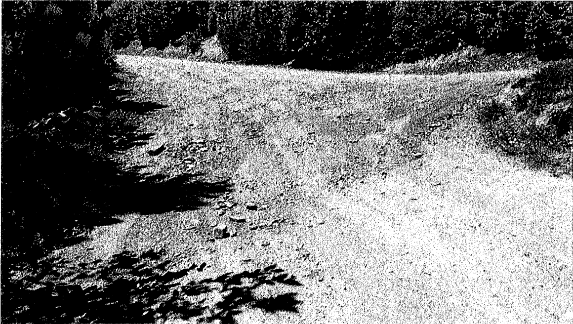
Road Point 3: A rolling dip is installed at this location to direct road runoff off of the road. Owner will monitor and maintain the rolling dip so that road runoff is adequately diverted.
