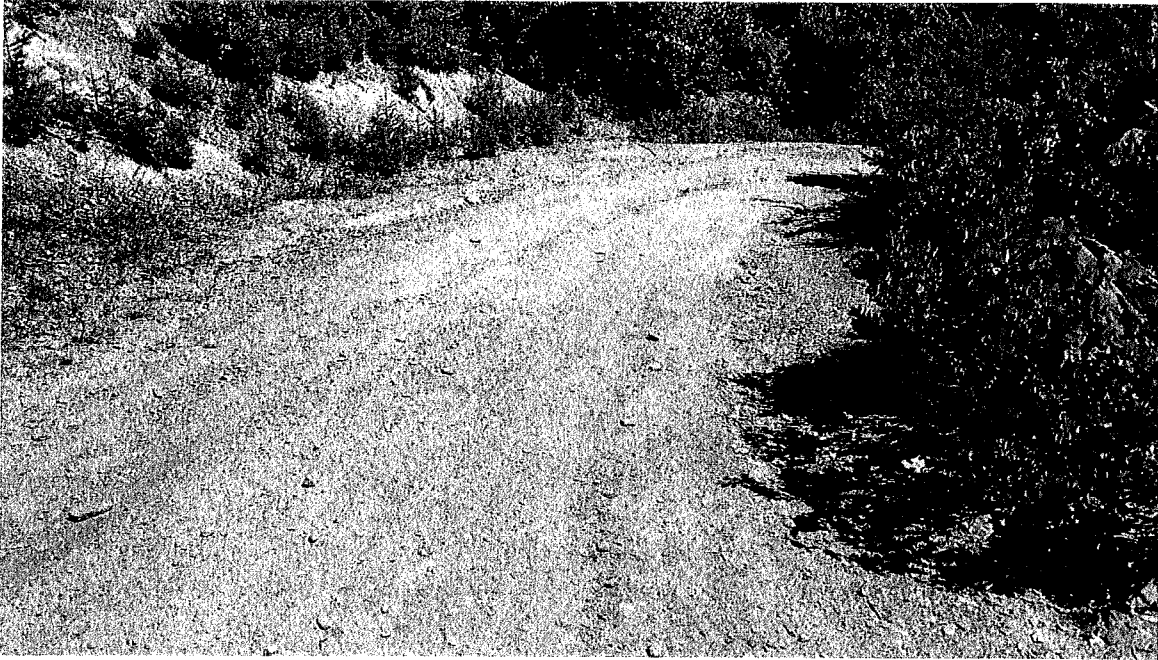
Road point 2: Alternate view of road erosion. Water is running down the middle of the road. We recommend a water bar or rolling dip be implemented to divert surface water off the roadway. The mitigation measures will improve the longevity of the road and reduce sediment delivery in heavy storm events.(See figure 36 & 40) July 25 th 2016
