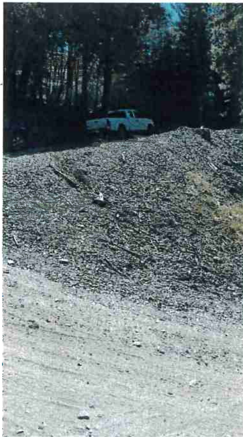
Picture 6: Road Point 4, the fill slope will be stabilized by placing rock on the inside corner and spreading seed to vegetate the rest of the fill slope.
