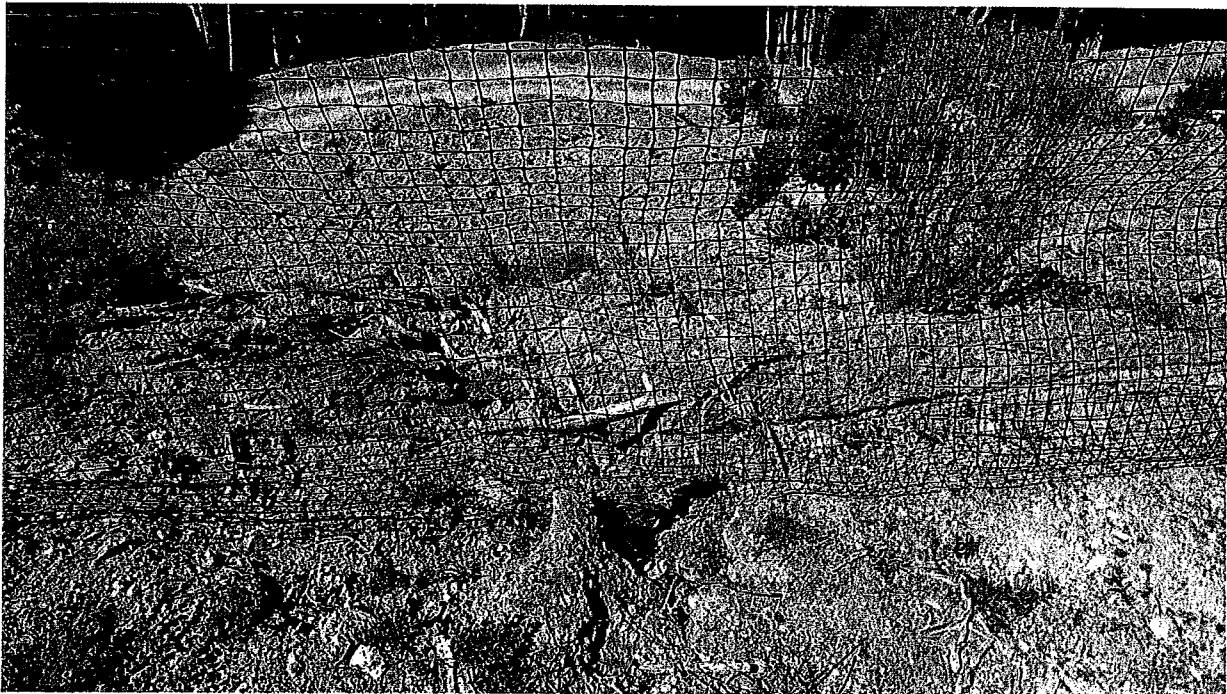
Picture 11: Looking down the fill slope from Map Point 1 showing the beginning of erosion rilling and gullyng.
