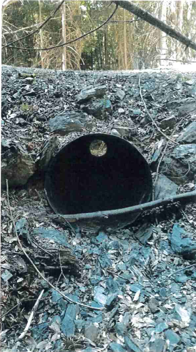
Picture 12: Road Point 9, Class II watercourse crossing with a 30-inch diameter corrugated metal pipe. This culvert has a large branch across the inlet. Removal of this debris is recommended before winter to prevent further accumulation of debris resulting in severe plugging of the culvert.
