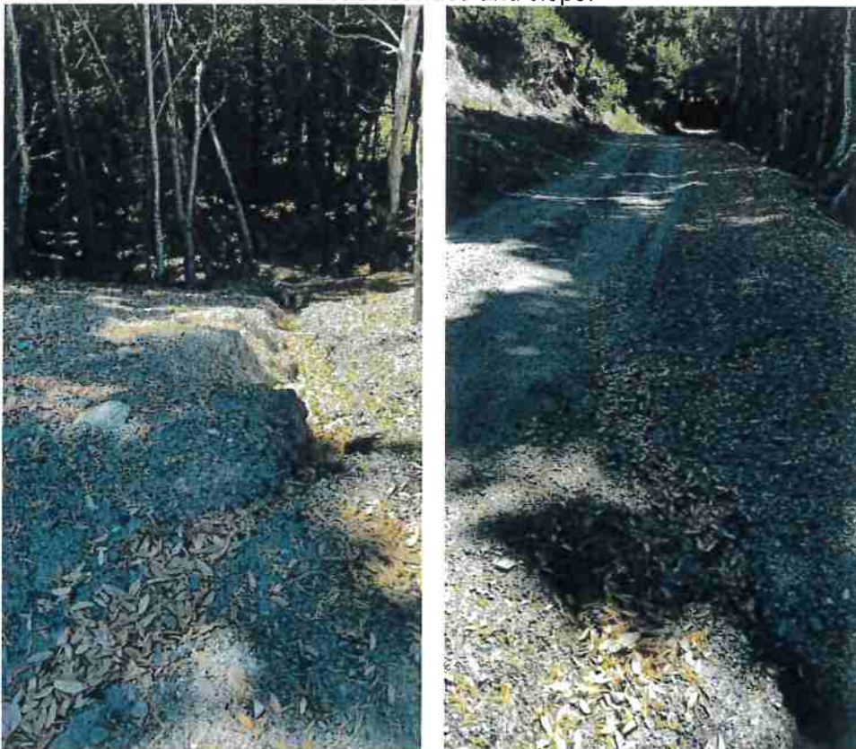
Picture 8: Road Point 14, the Discharger will out-slope the road around the base of the cultivation site fill slope to the armored fill/rocked ford at Road Point 3 and resurface the road with road rock.
