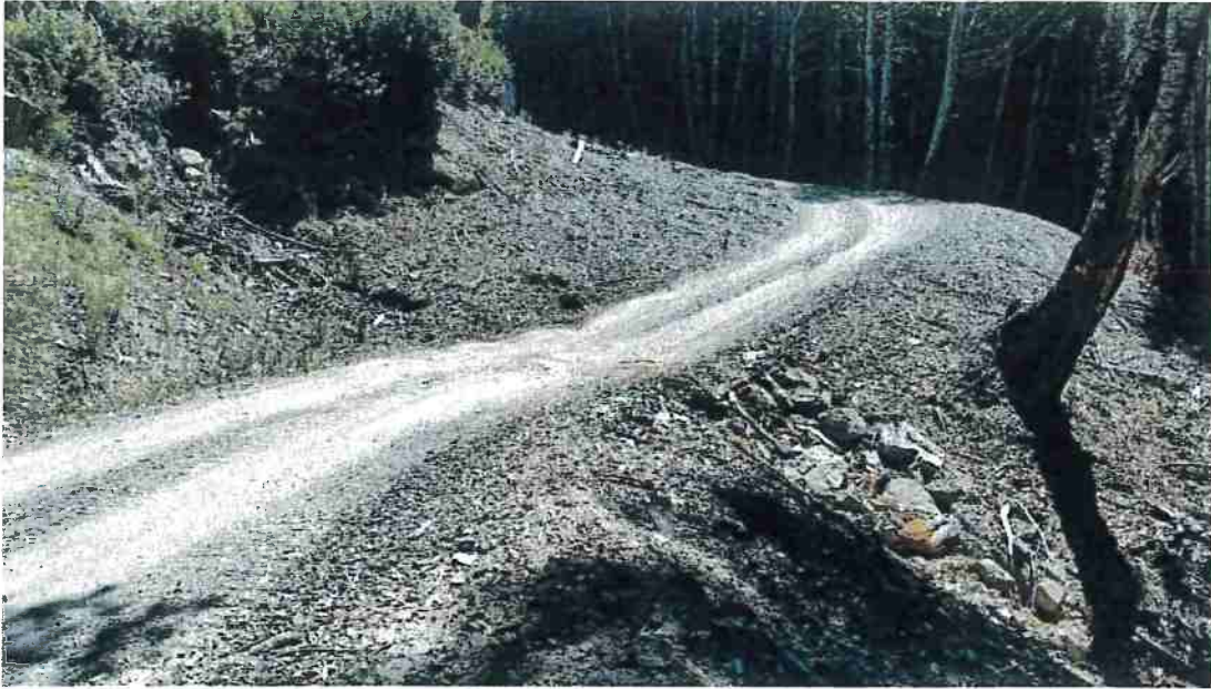
Picture 5: Road Point 3, an armored fill/rocked ford will be placed here to upgrade the degraded existing one.
