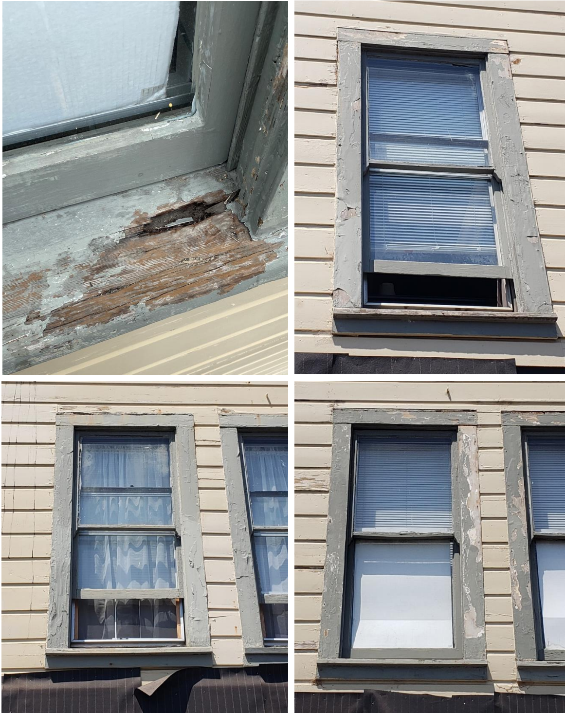
Figure 6: Images of rotted and deteriorated window framing
