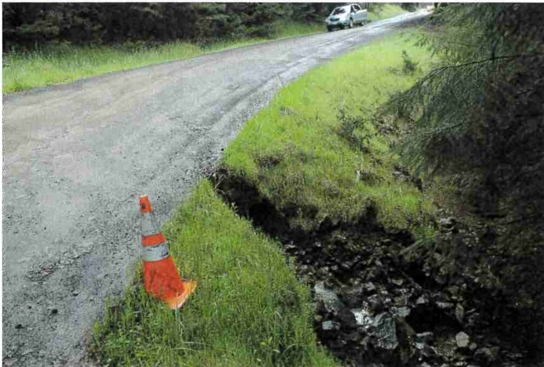
Photo 6. Mile 5.6: Add rock to culvert outlet to prevent erosion of road surface.
