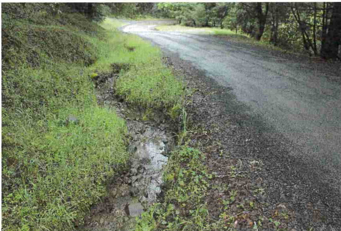
Photo 5. Mile 6.2: Inboard ditch erosion, new culvert at natural swale proposed to eliminate problem.
