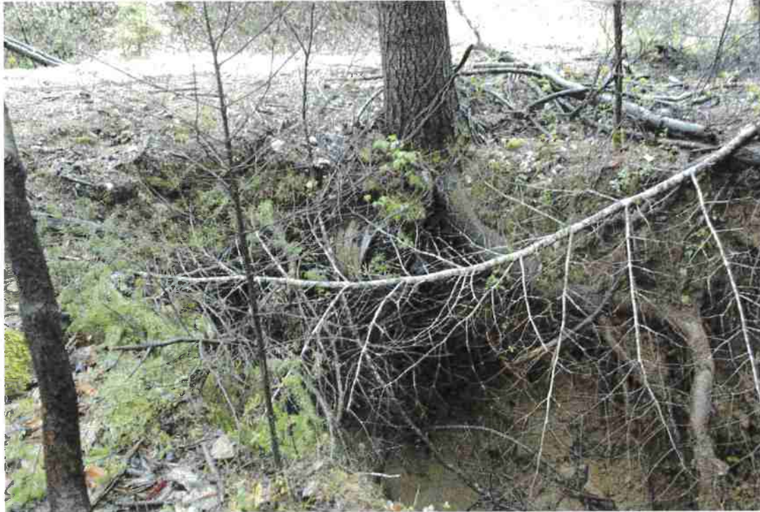
Photo 14. Mile 6.6: Culvert replacement proposed on culvert that is failing and will eventually cause pinch point.
