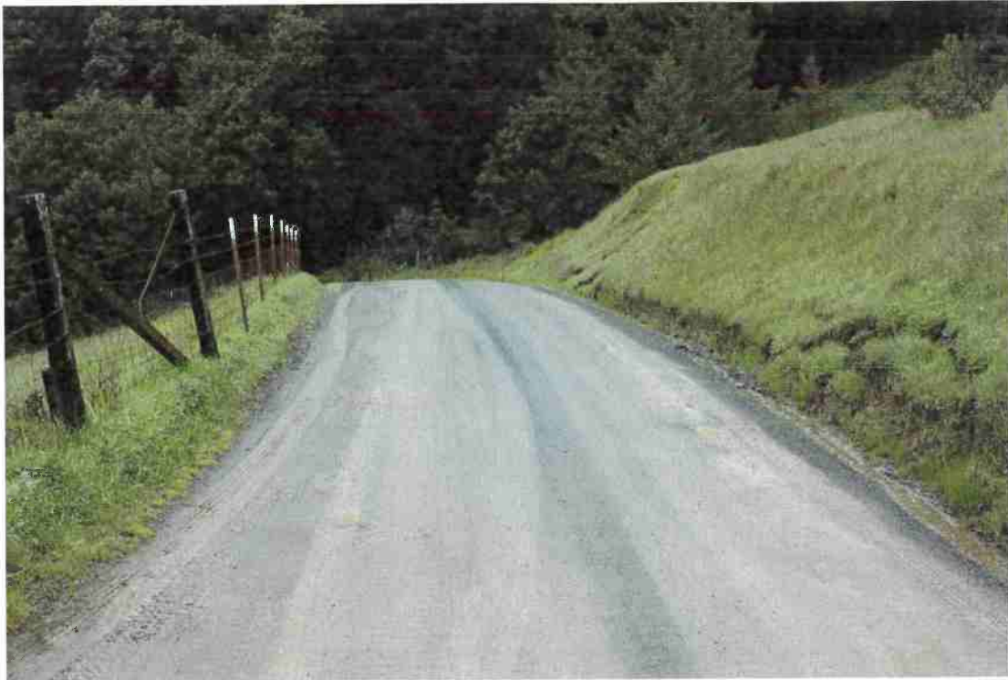
Photo 3. Mile 5.4: 12-ft-wide pinch point with no shoulders.
