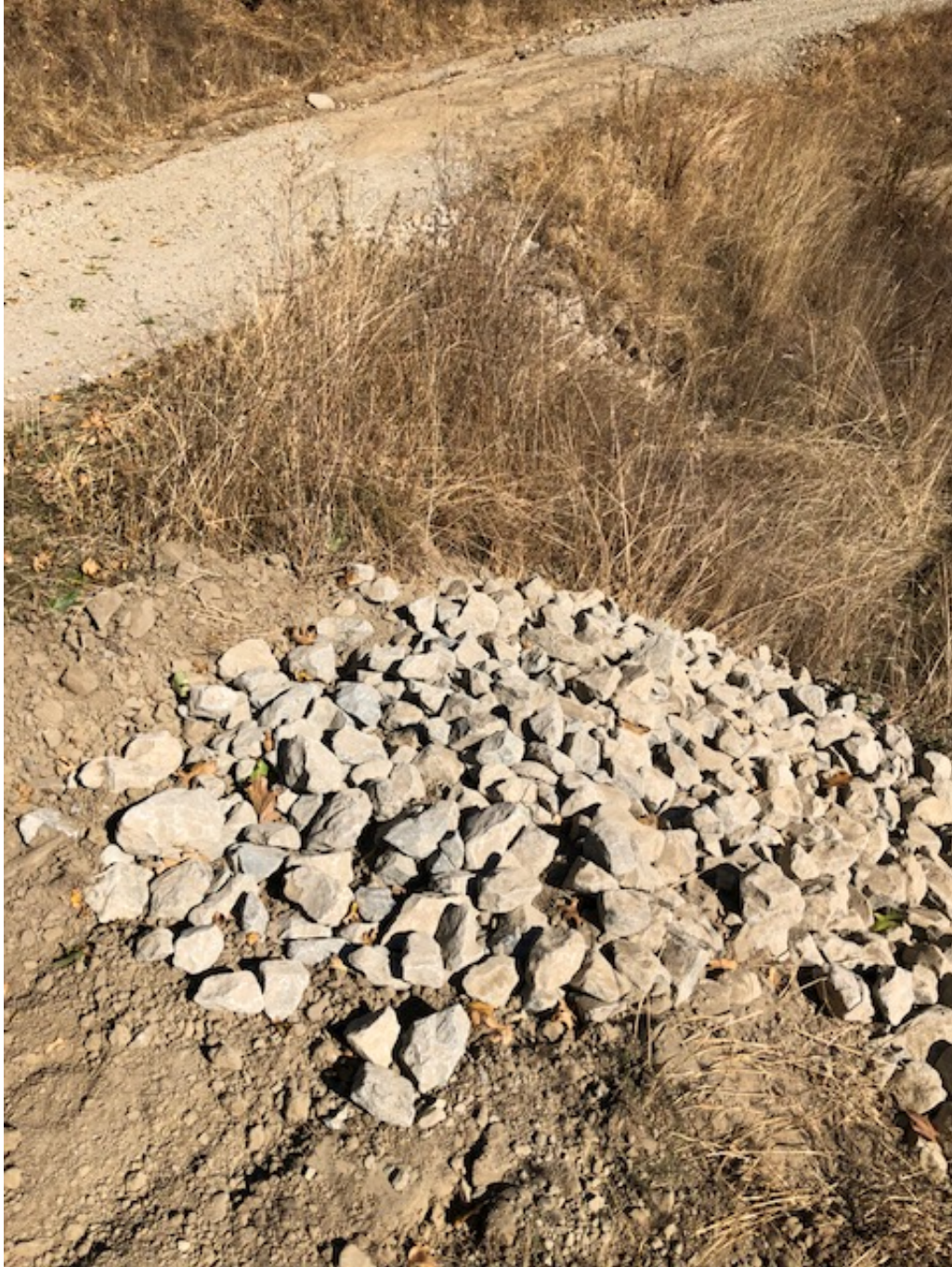
Figure 6: Riprap armored outlet of WB-3, the third waterbar east of the residence.
