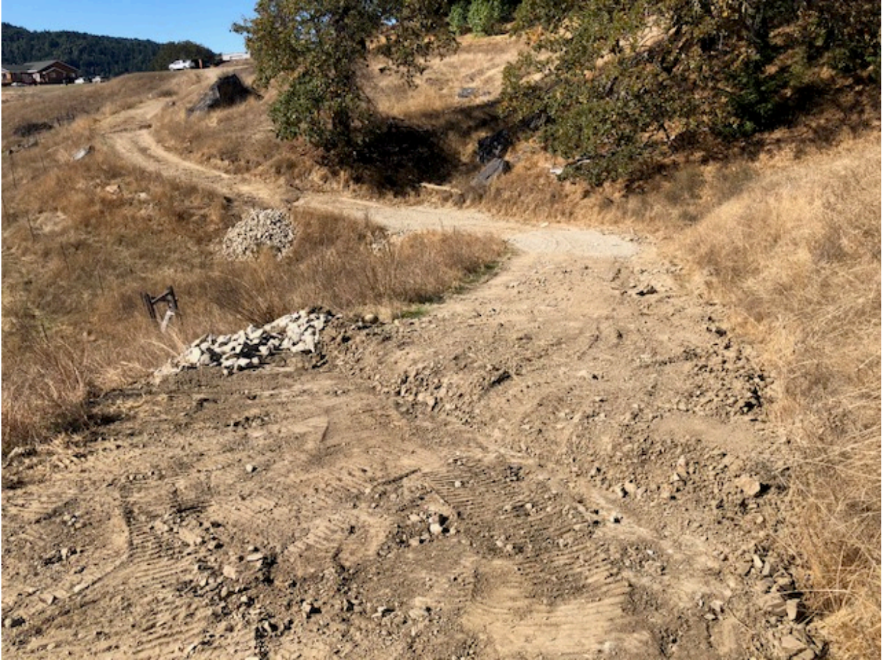
Figure 9: Installation of WB-5 in the foreground and RB-2 in the midground looking west toward residence.
