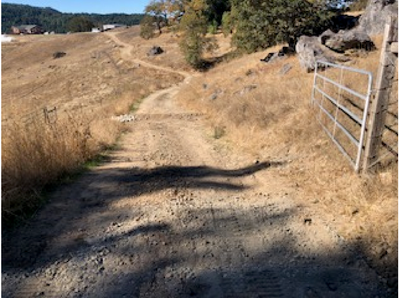
Figure 11: The foreground shows some of the roadbase installed at RB-4, WB-7 is visible in the midground.
