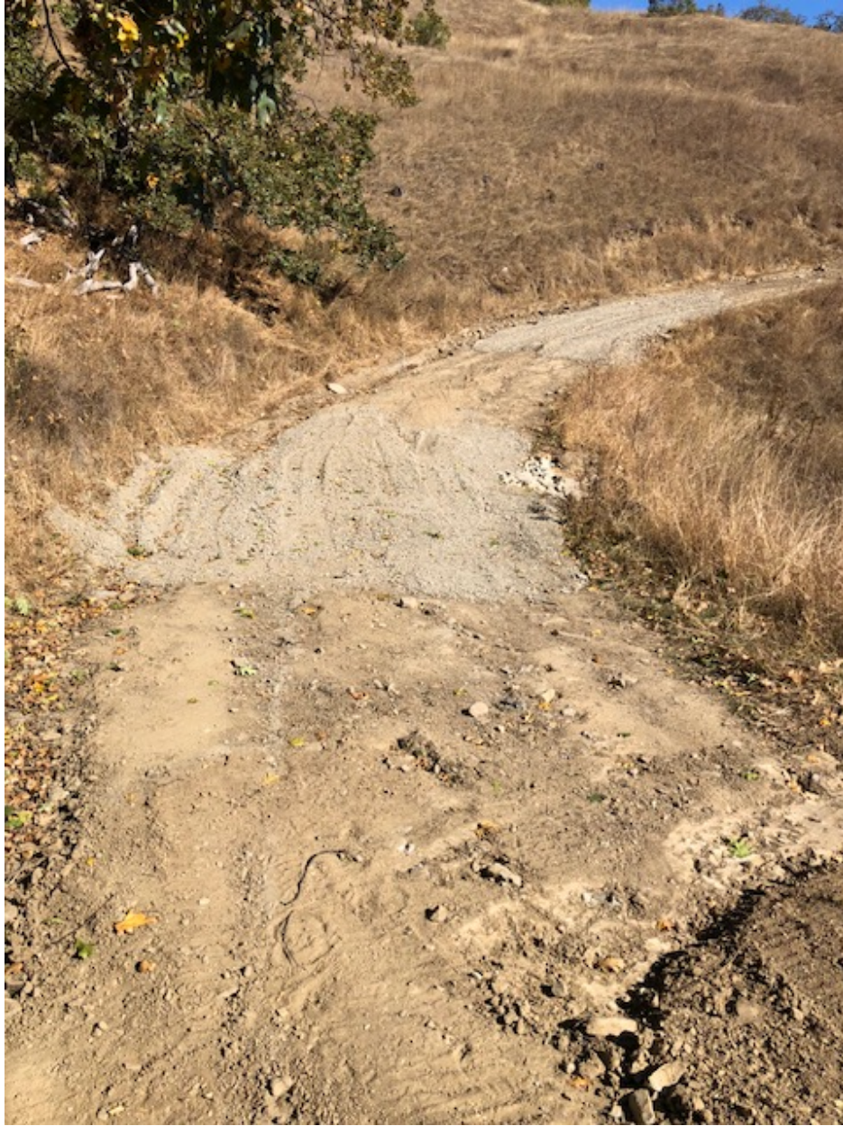
Figure 7: Installation of roadbase at the sites of stream crossings. RB-1 in foreground, RB-2 in background.
