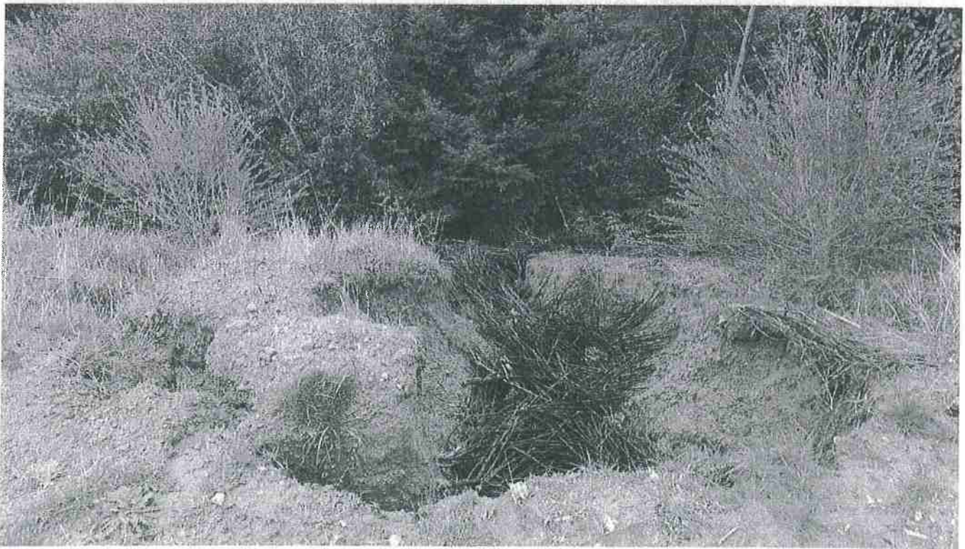
Site 25 – Runoff from the cultivation area is being concentrated and drained onto the landing pads fillslope, resulting in the gulying and caving of the fillslope. Concentrated runoff continues down the hillside to the Mattole River.
