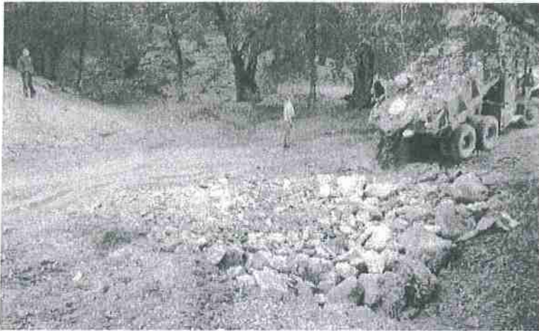
FIGURE 121D. Well graded rock armor is then tumbled into the structure and spread across the breadth of the U-shaped stream crossing, and about one-third the way up the roadbed, so that streamflow will only flow over or come in contact with resistant armor material. The armor must be spread and compacted across the design width of the expected flood flow channel width so peak flows will not flank the armored structure.
