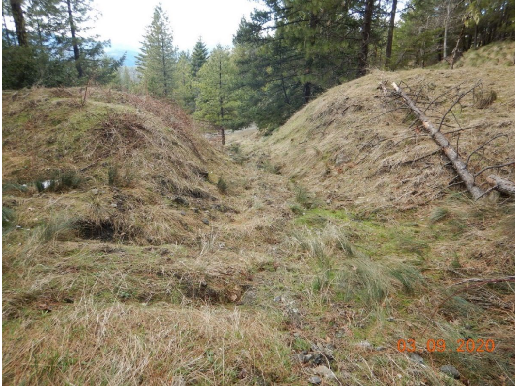
Photo 36. The breached berm of the former pond at Additional Point 1.
