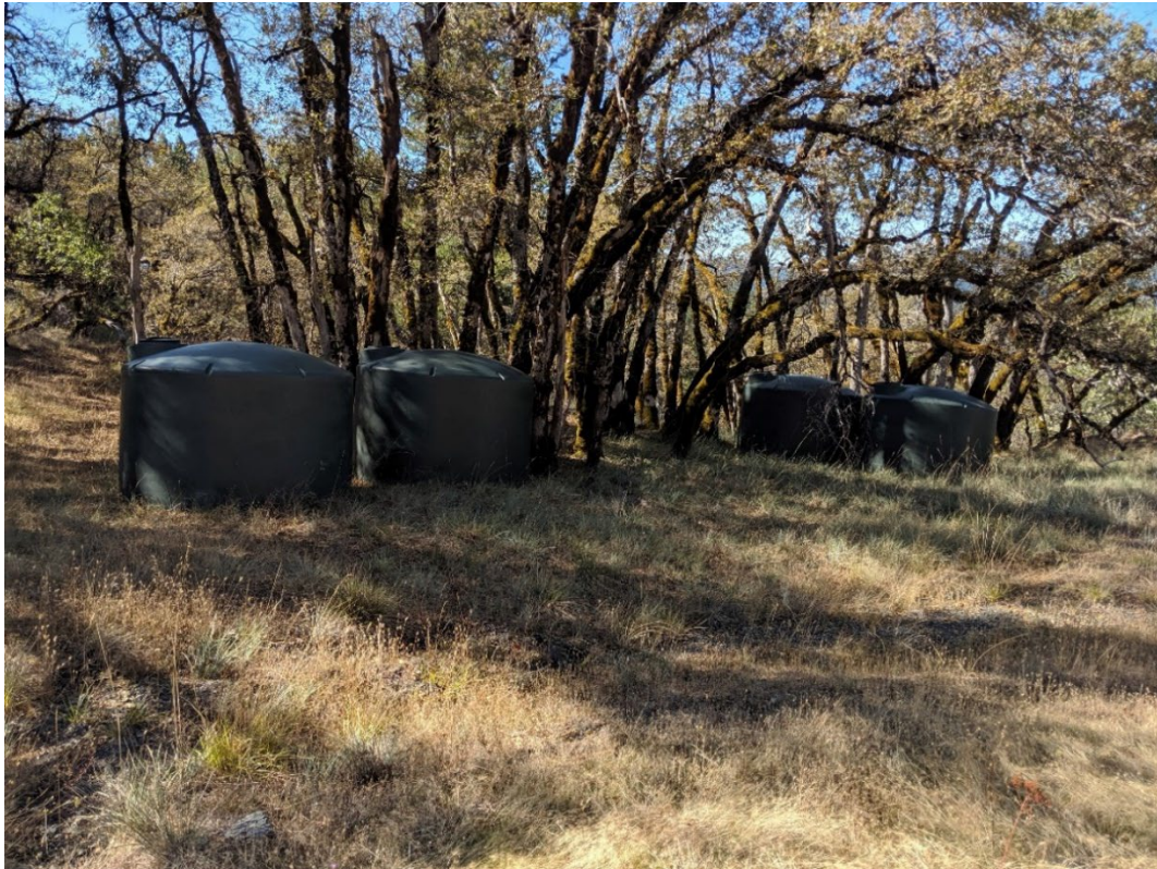
Photo 19. Four 2,500 Gallon hard-sided water storage tanks on APN 210-144-012-000.
