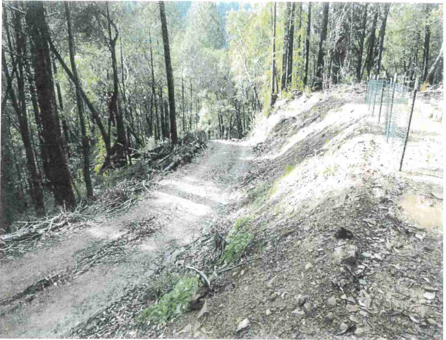
Picture 8: Storm run-off is flowing down this road where it is discharging sediment to a nearby Class III watercourse. A drainage feature such as a rolling dip or water break shall be installed at this location, MP #1, per specifications attached with this document. Photo date: 03/09/2018.
