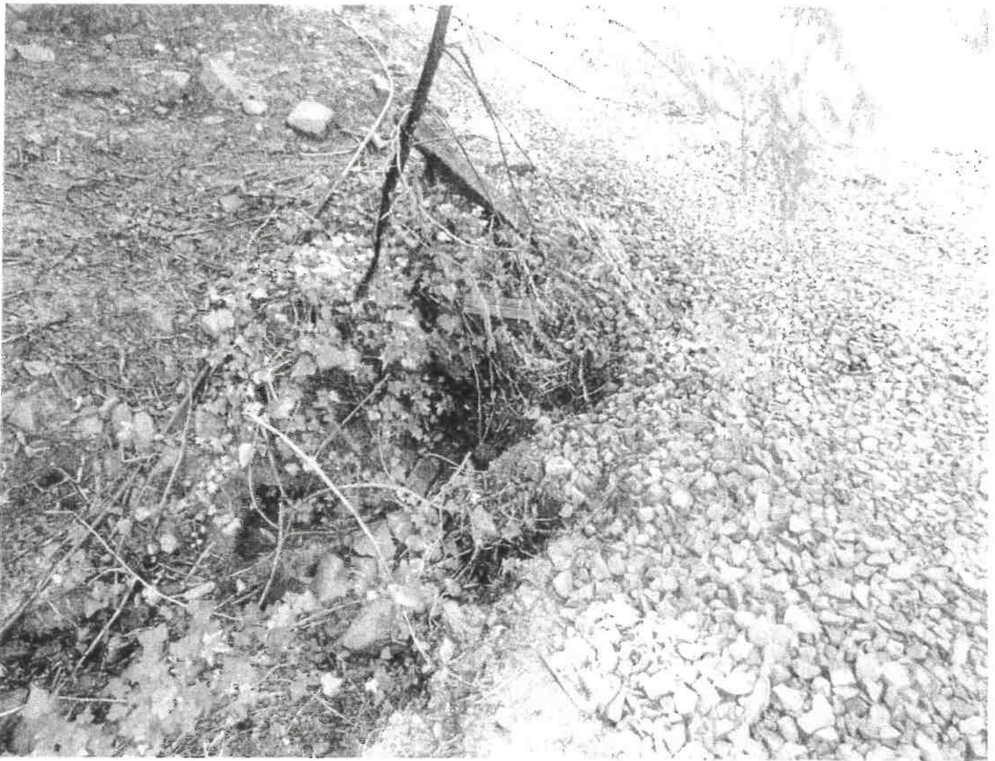
Picture 17: Outlet of 24" diameter Stream Crossing #1. The outlet has been driven over multiple times. The Discharger shall upgrade this crossing to a minimum 36" diameter culvert (metal or plastic). Photo date: 03/09/0218.
