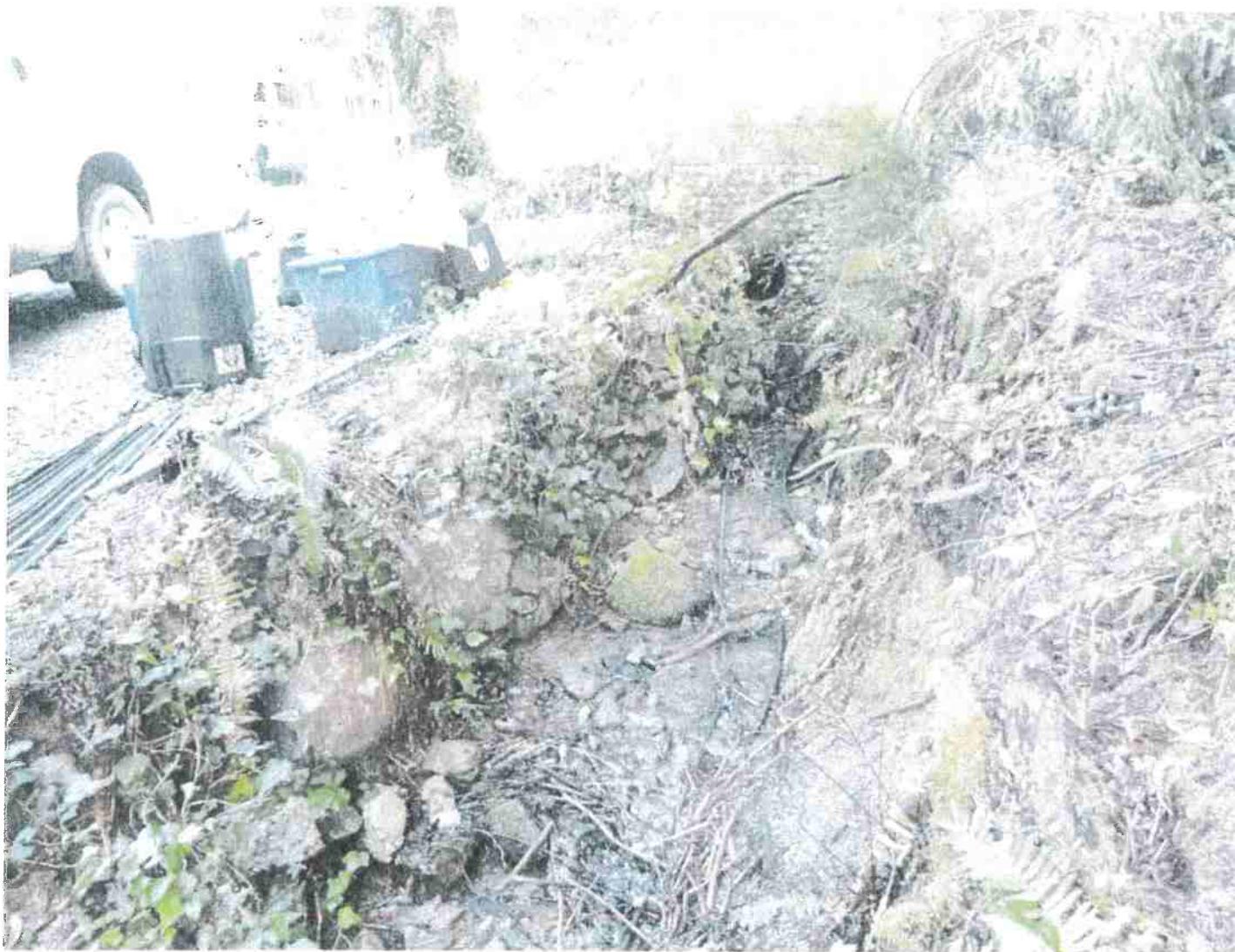
Picture 20: View of the outlet of SC #2 looking up from the inlet of SC #1. In the event that SC #2 either plugs with debris or backs up due to excess surface flow, water will flow around the garage and back into the channel due to topography. Photo date: 03/09/2018.
