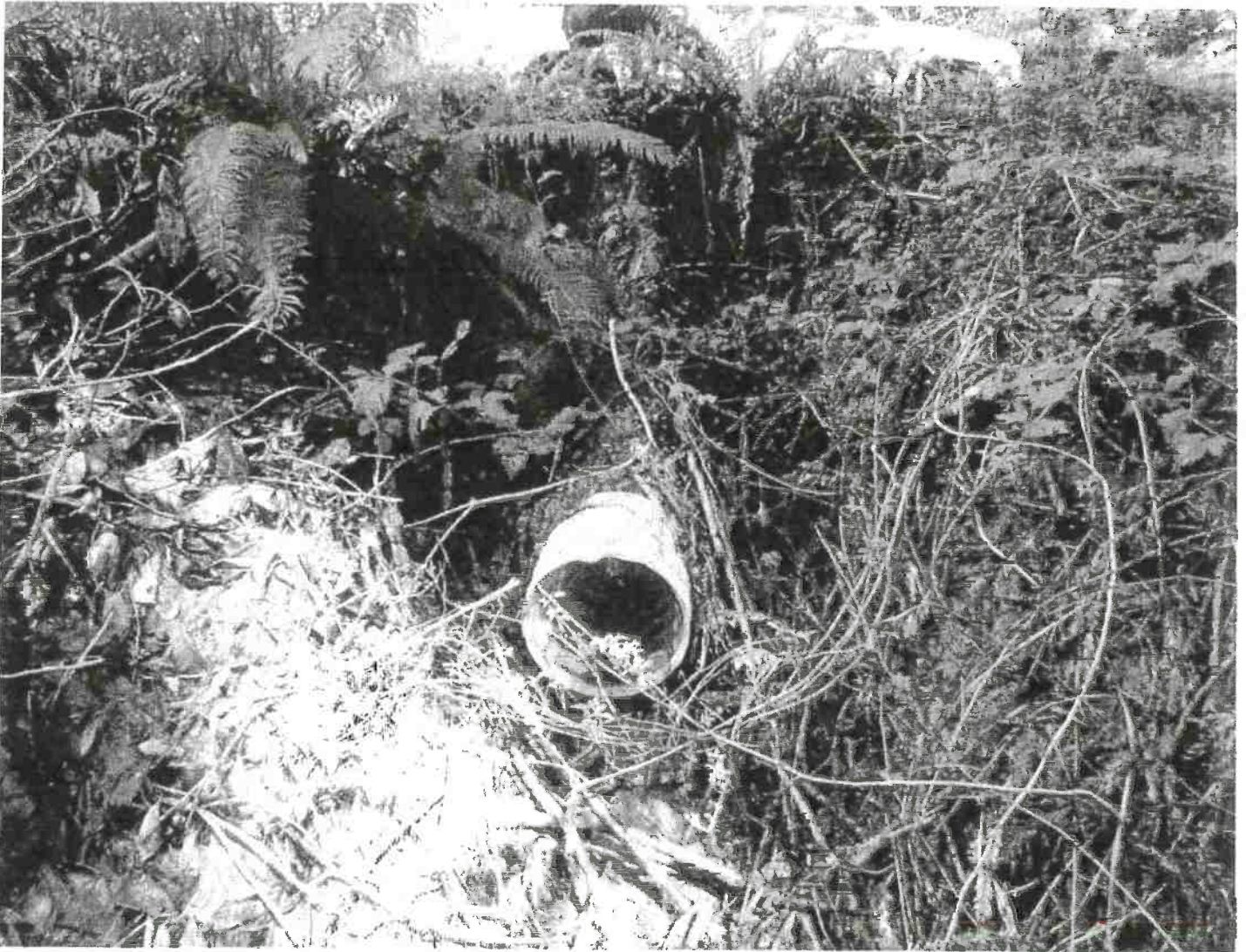
Picture 15: Damaged outlet of the 12" diameter relief culvert located at MP #5. This location shall be upgraded to a minimum 15" diameter culvert and installed per attached specifications. Photo date: 03/09/2018
