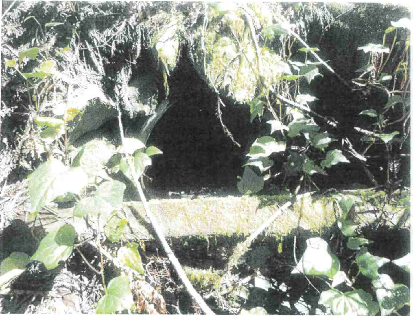
Picture 16: Inlet of 24" diameter Stream Crossing #1. This crossing is located where an unnamed Class II watercourse intersects with a permanent road. Photo date: 03/09/2018
