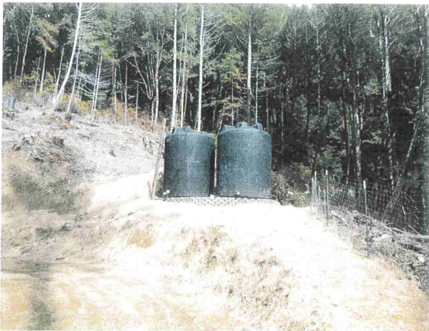
Picture 4: The well is located in between these two 5,000 gallon rain catchment/storage tanks. Photo date: 03/09/2018.
