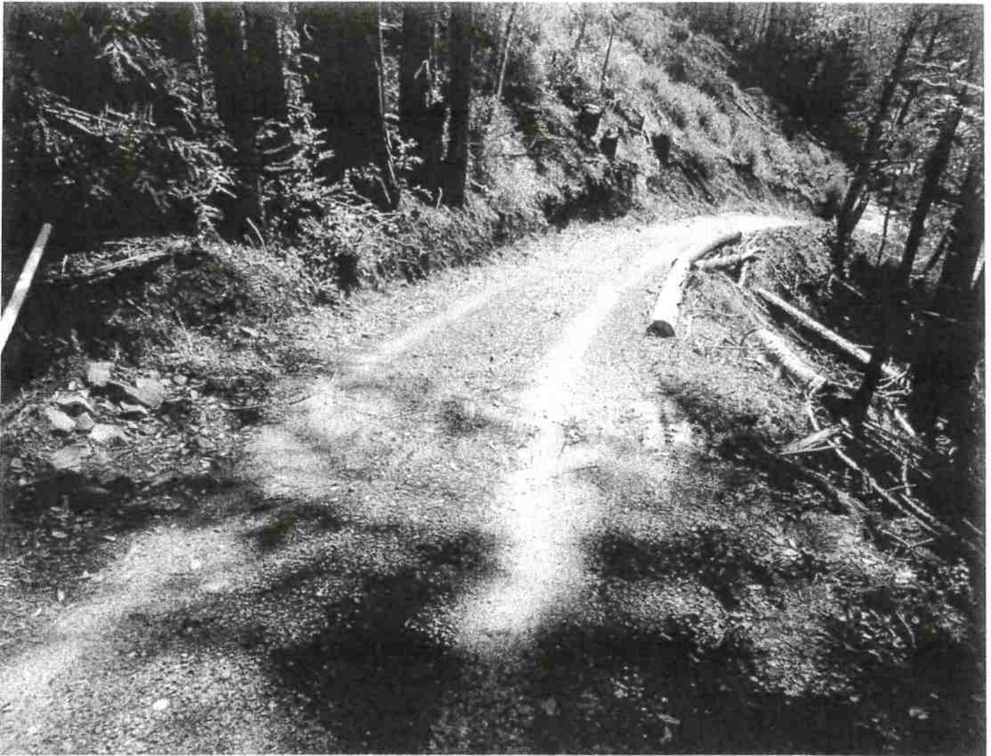
Picture 11: MP #4 is where a swale feature intersects with the access road on the property. The Discharger shall install a relief culvert per attached stream crossing specifications at this location. Photo date: 03/09/2018
