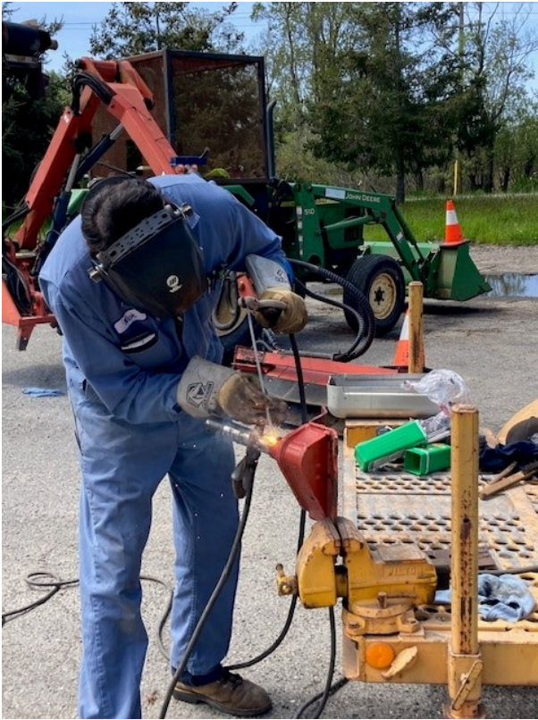
Lead City Mechanic working on equipment maintenance.
