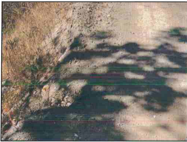
Photo #145 River Rd Looking @ Erosion Issue From Lack of Functioning Culvert
