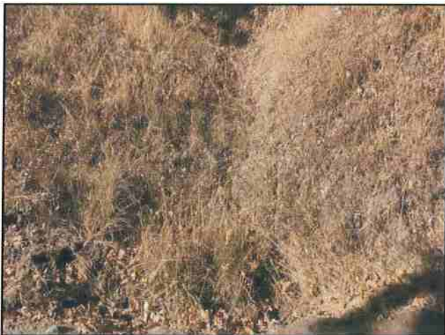
Photo #51 River Rd Looking North @ Slide Area Feeding Culvert In Photo #50
