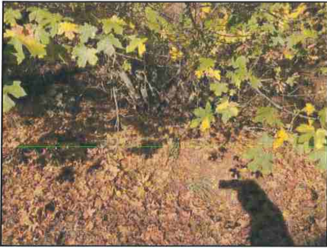
Photo #301 River Rd Looking @ Partially Clogged 24" Culvert In
