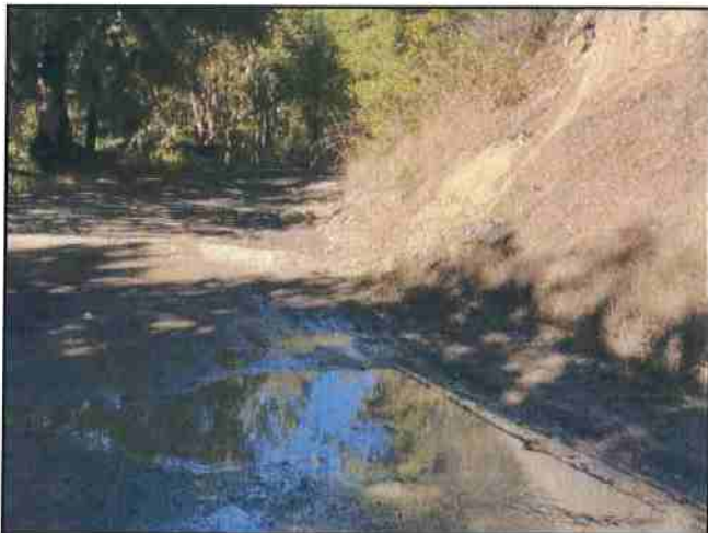
Photo #261 River Rd Looking NW @ Curve w/ Turnout & Drainage Issue
