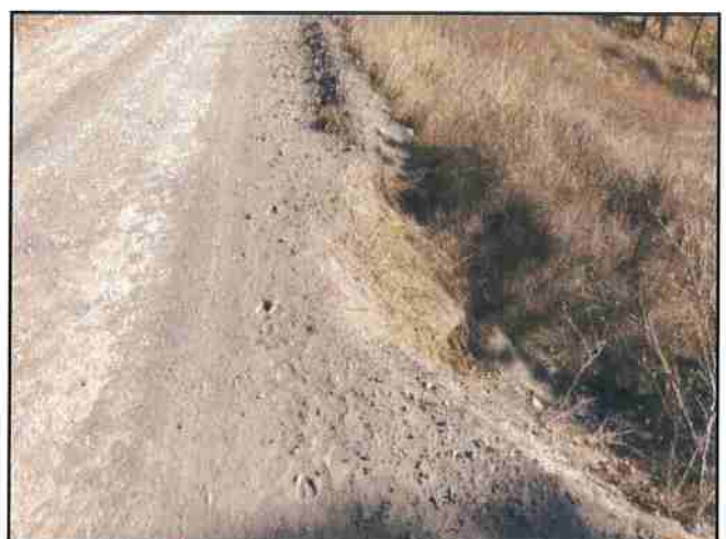
Photo #30 River Rd Looking SE @ Erosion
