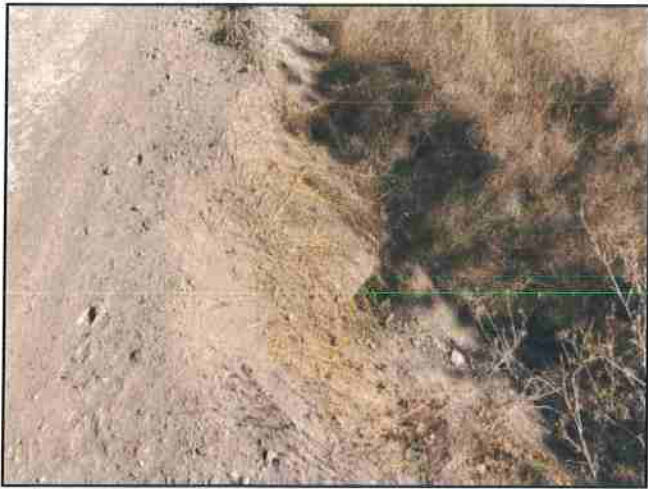
Photo #31 River Rd Looking SE Closeup @ Erosion
