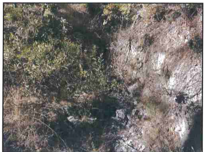
Photo #90 River Rd Looking @ Clogged 24" Culvert In
