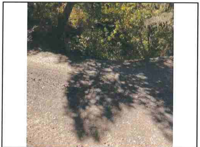
Photo #244 River Rd Looking @ Erosion Occur- ing
