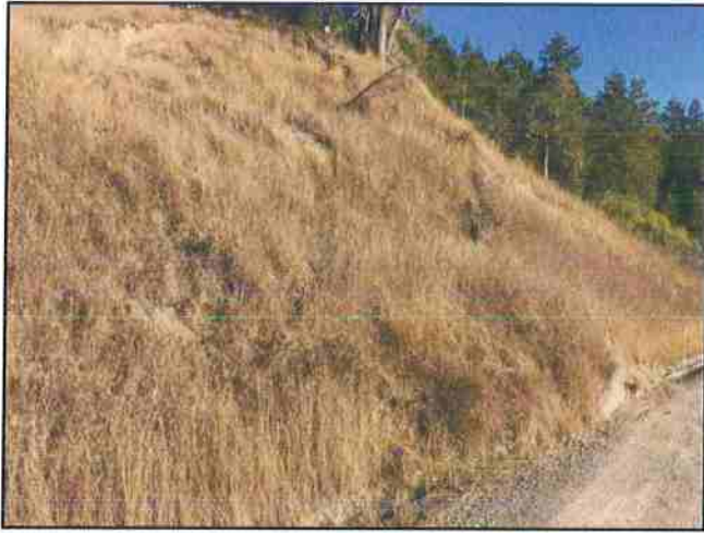
Photo #223 River Rd Looking @ Hillside Slip
