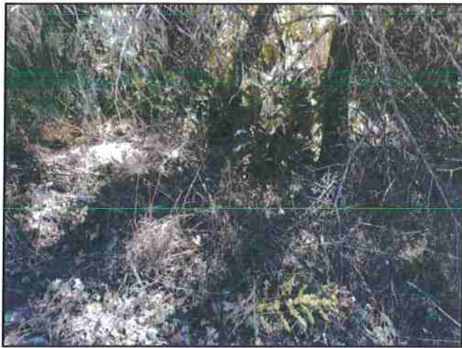
Photo #61 River Rd Looking @ Clogged Culvert In
