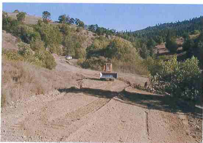
Figure 31. Bulldozer reshaping road surface to out-sloped condition to improve drainage. Photo: Jared Gerstein.
