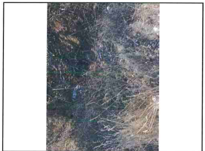
Photo #28 River Rd 12" Clogged 12" Culvert Out
