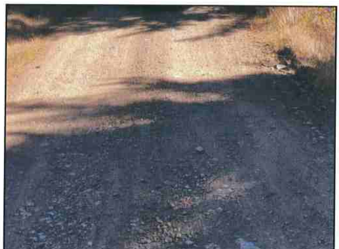
Photo #310 River Rd Looking @ Drainage Issue w/ Pooling Water Location
