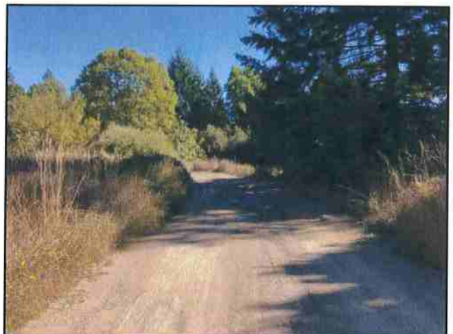
Photo #430 River Rd Looking SE @ Curve w/o Turnout & Drainage Issue
