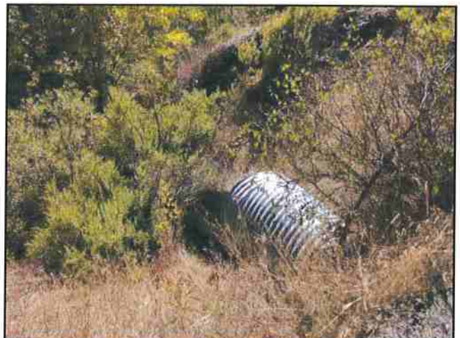
Photo #358 River Rd 36" Culvert Out
