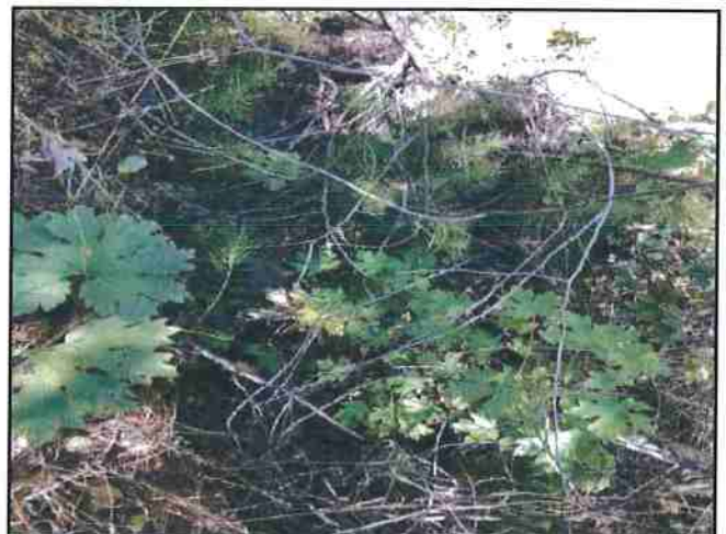
Photo #154 River Rd Looking @ Partially Clogged 36" Culvert In
