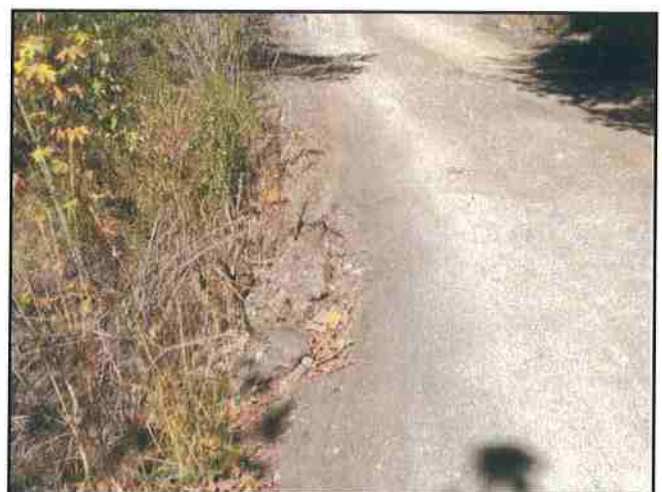
Photo #270 River Rd Looking @ Drainage & Erosion Issue
