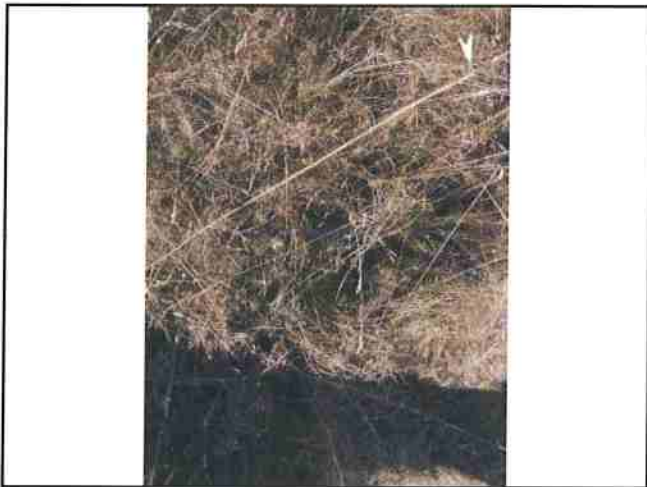
Photo #33 River Rd Possible Culvert In. No Culvert Out Was Identified.
