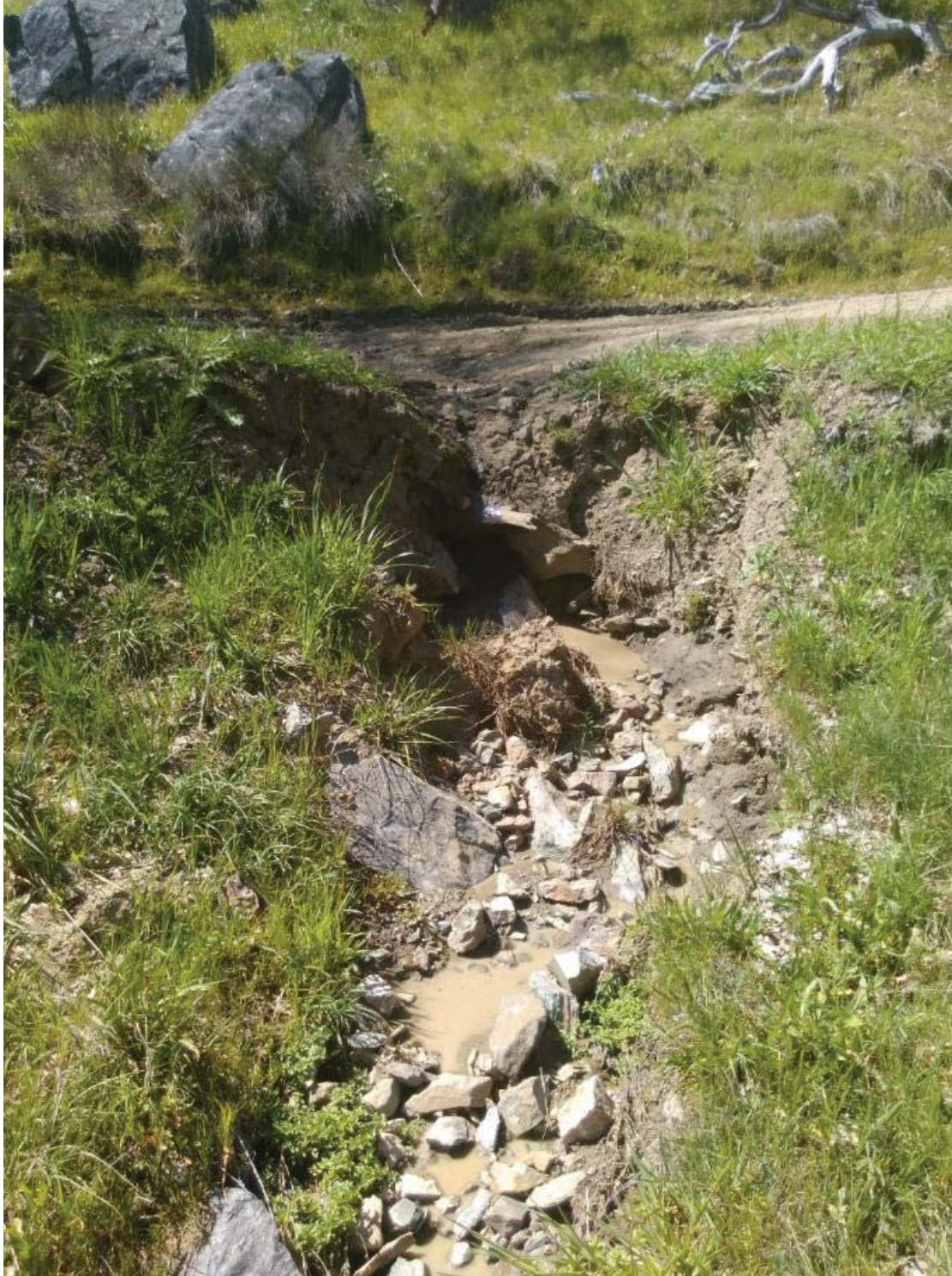
AC-1. View of erosion on the downslope side caused by hydrologic connectivity.
