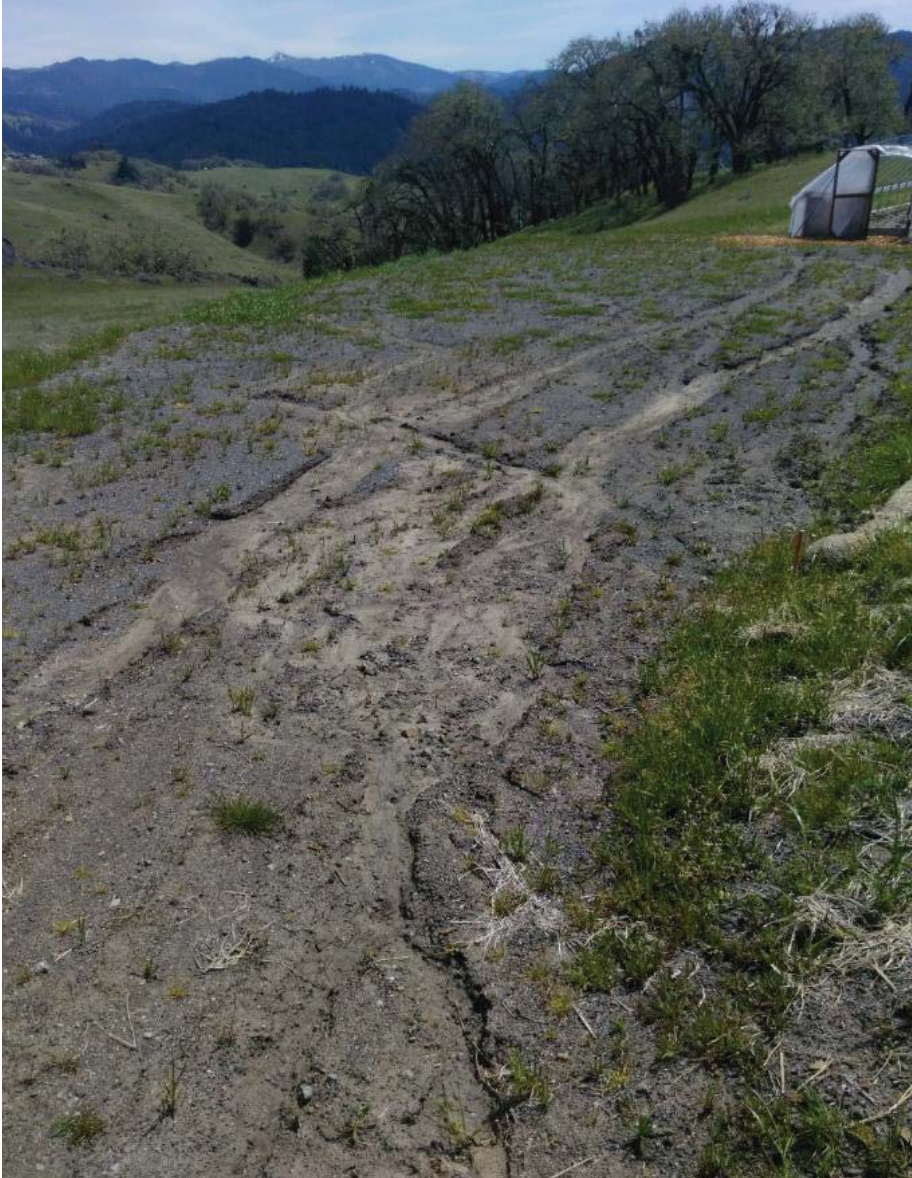
Landing at the NE corner of CA-5 showing channelization and erosion from runoff
