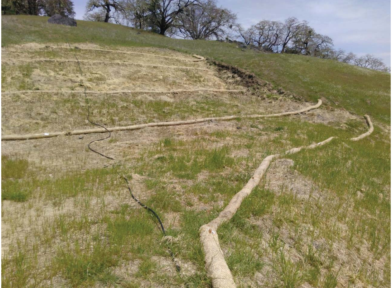
NW corner of CA-3 showing raw exposed banks, site of NOV-4, Above drainage of CV-2
