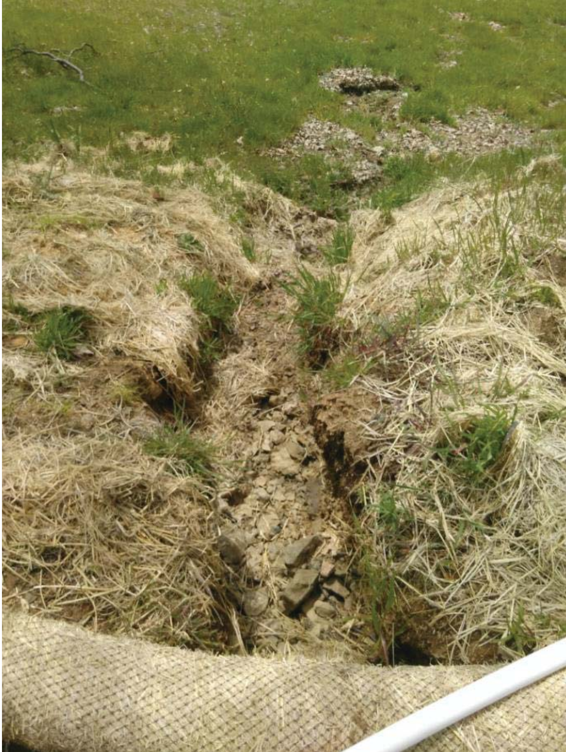
Outlet at SW corner of CA-2 and sediment deposition. Silt fences to be installed as a protective measure until further revegetation is achieved.
