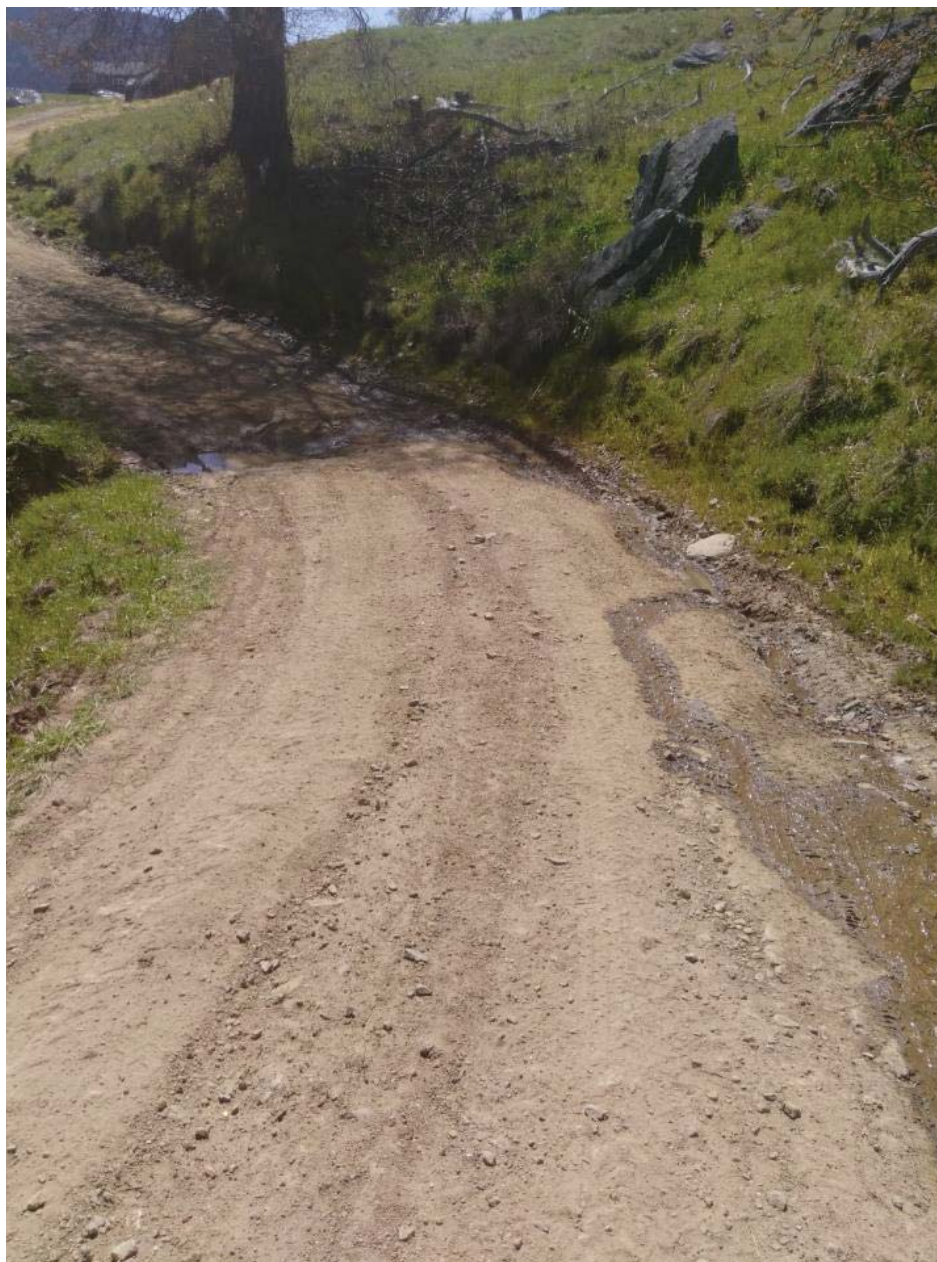
AC-1. Seepage from both directions on the roadway forms a dip and spills off the roadway at this low point. Armored crossing to be installed or alternate road access. Road segment to be improved per PWA Roads Manual.
