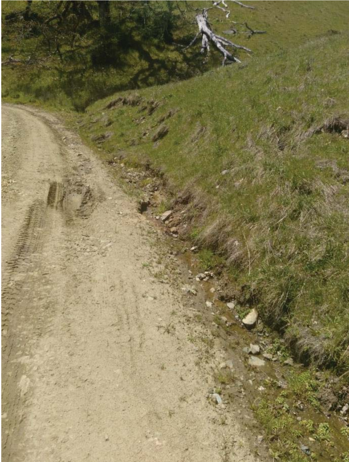
Inboard ditch between CV-1 and CV-2 is poorly defined and hydrologically connected to inlet of CV-1
