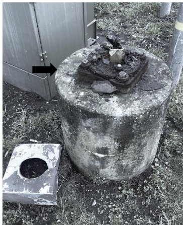
Image 1: Rusted and corroded light pole base.
