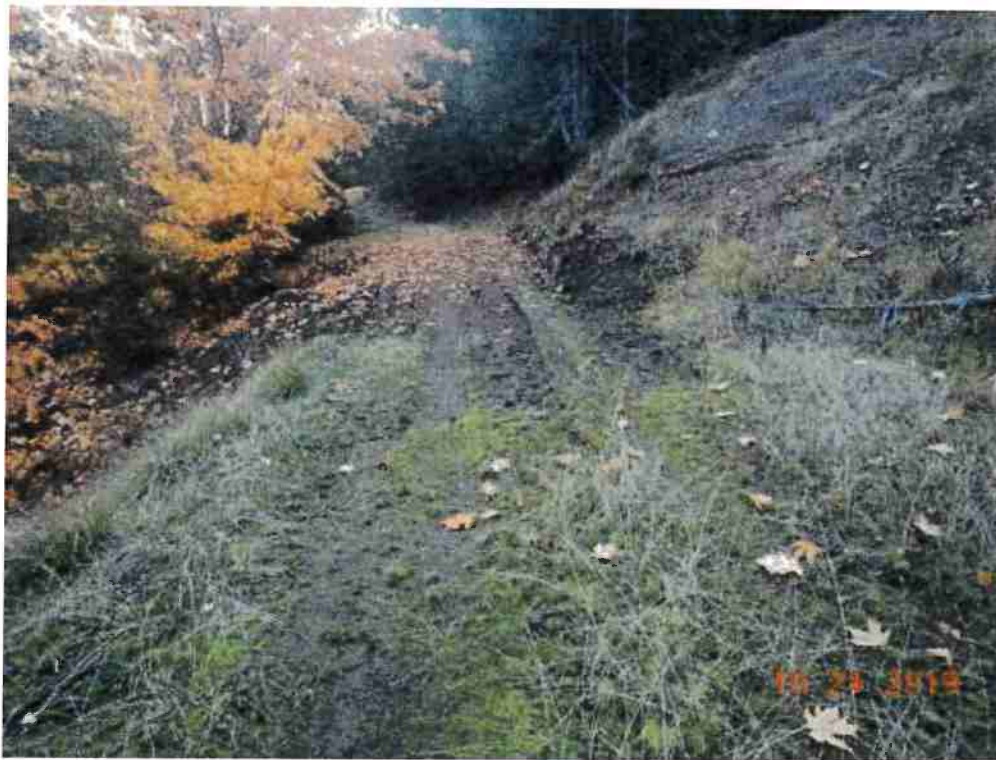
Photo 26. Right approach of 60" crossing, goes through historic landslide
