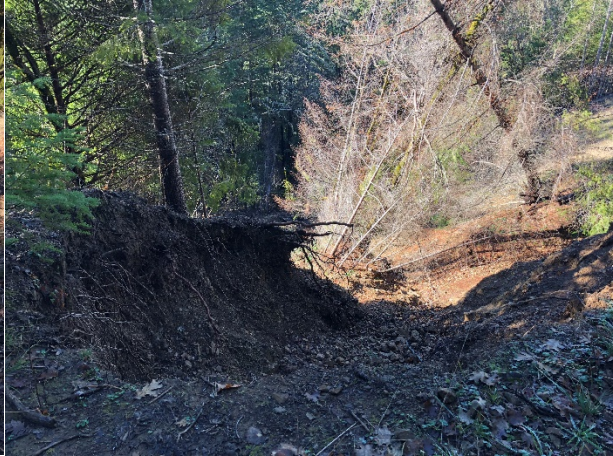
Picture #20 On PG&E esmt looking SW @ erosion.
