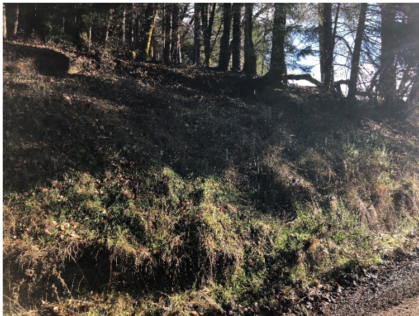
Picture #11 Cobb Rd looking NE @ sloughing of embankment
