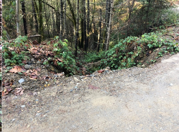
Picture #8 road washout due to culvert being clogged.
