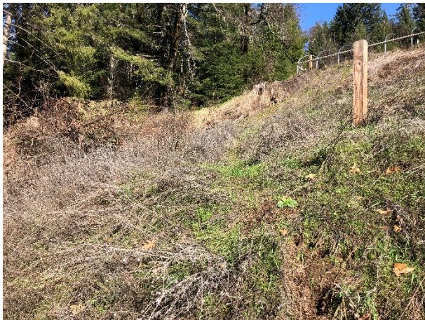
Picture #59 Looking uNW @ erosion @ outlet of culvert in Picture 58
