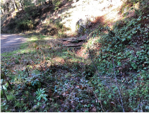
Picture #49 Cobb Rd @ double 12" culvert w/ dam in middle
