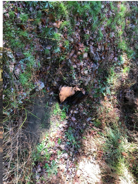
Picture #46 Cobb Rd looking at 12" crushed CMP inlet
