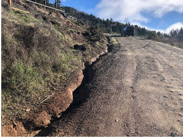
Picture #13 Cobb Rd looking NE @ erosion due to drainage
