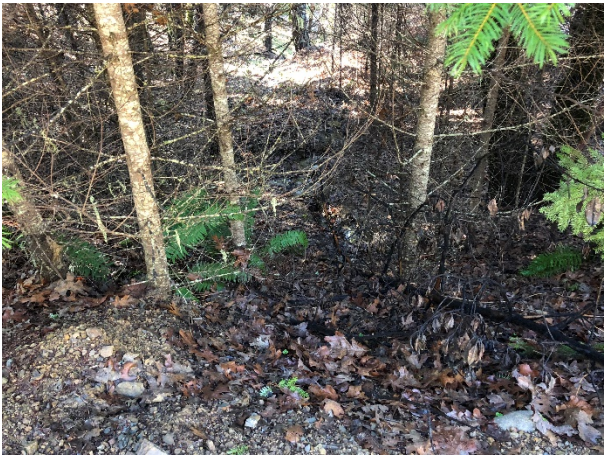
Picture #27 Cobb Rd outlet & erosion from culvert @ Picture 26
