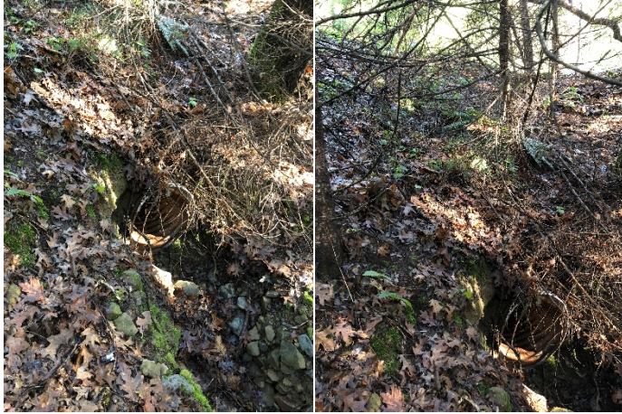
Picture #43 Cobb Rd inlet of 12" culvert Picture #44 Cobb Rd outlet from culverts in Pictures 42 & 43.
