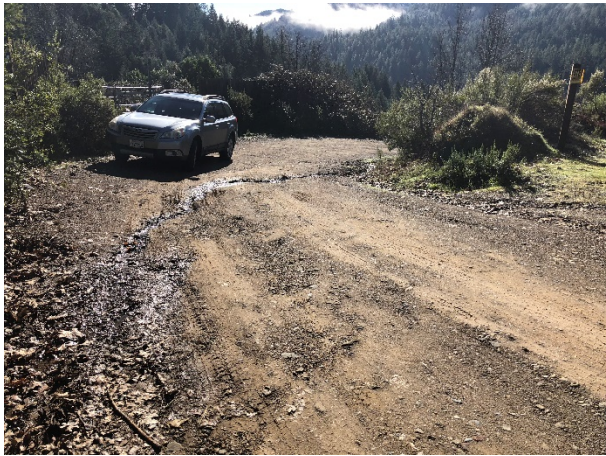
Picture #15 Cobb Rd looking SE towards curve in 14 w/ erosion
