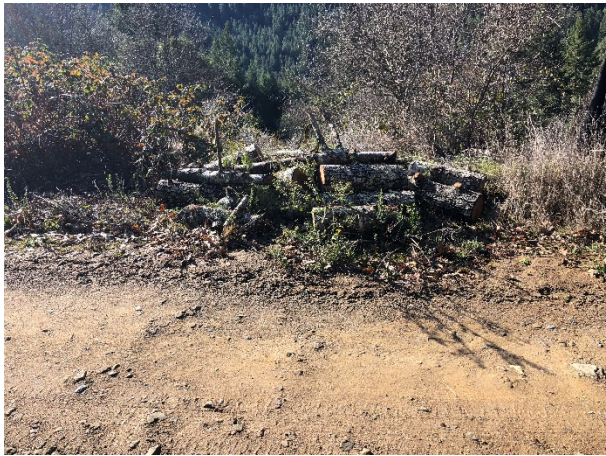
Picture #57 Cobb Rd @ outlet of culvert where water tops road
