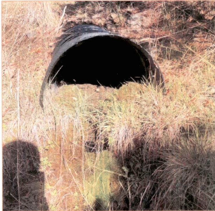
RP9) Clean and maintain DRC outlet.
