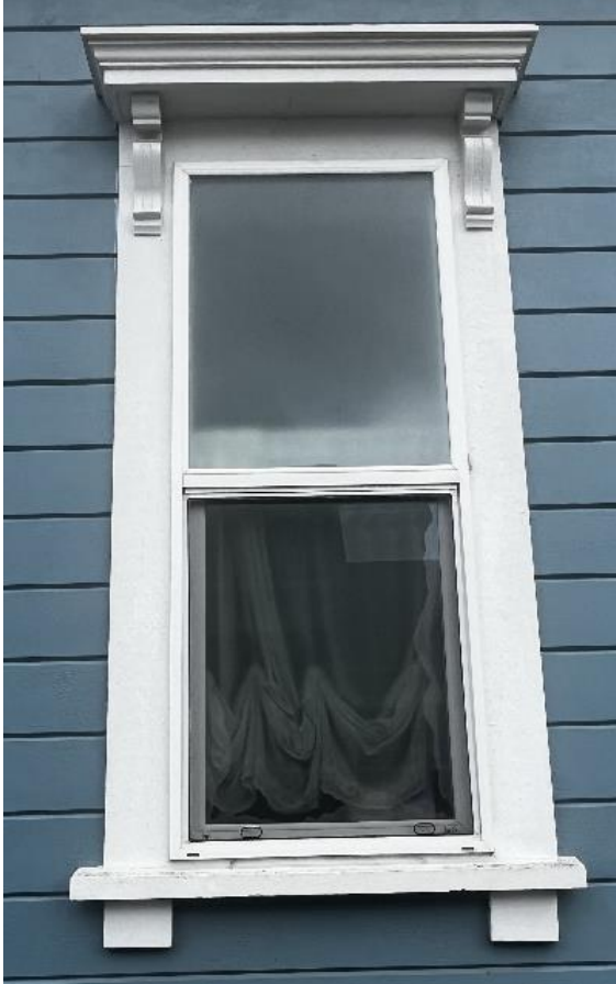
Figure 10: Close up view of visible water damage on the bottom right corner of 1 of 6 single-hung vinyl window to be replaced, photo taken on April 24, 2024
