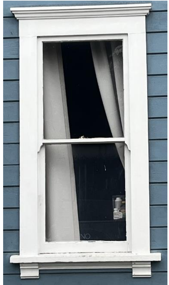
Figure 9: Only existing original wooden window to be repaired, photo taken on May 14, 2024
