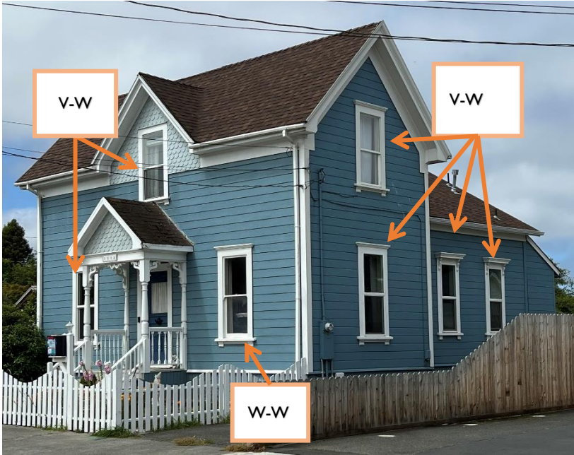
Figure 8 Street-view of 6 vinyl windows to be replaced and original wooden window to be repaired (vinyl windows labled V-W, wood window labled W-W)
