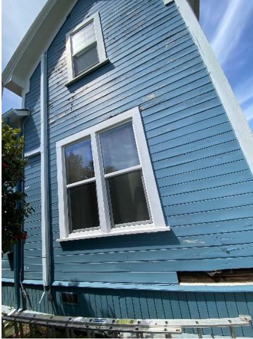
Figure 4: View of southern-facing façade prior to replacing pine siding and single-hung vinyl windows, photo taken September 2023
