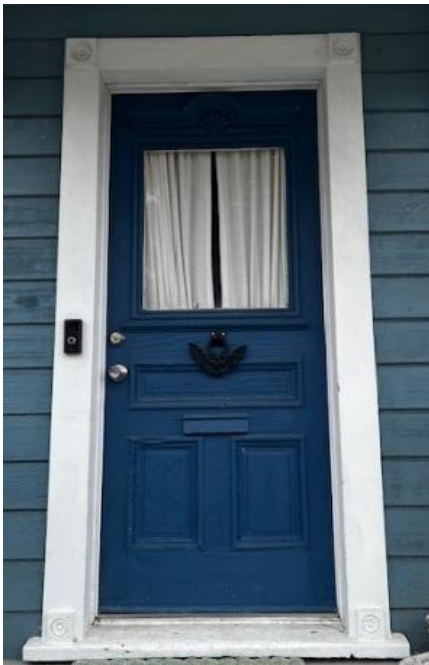
Figure 6: Front Door to be replaced, photo taken on April 25, 2024
